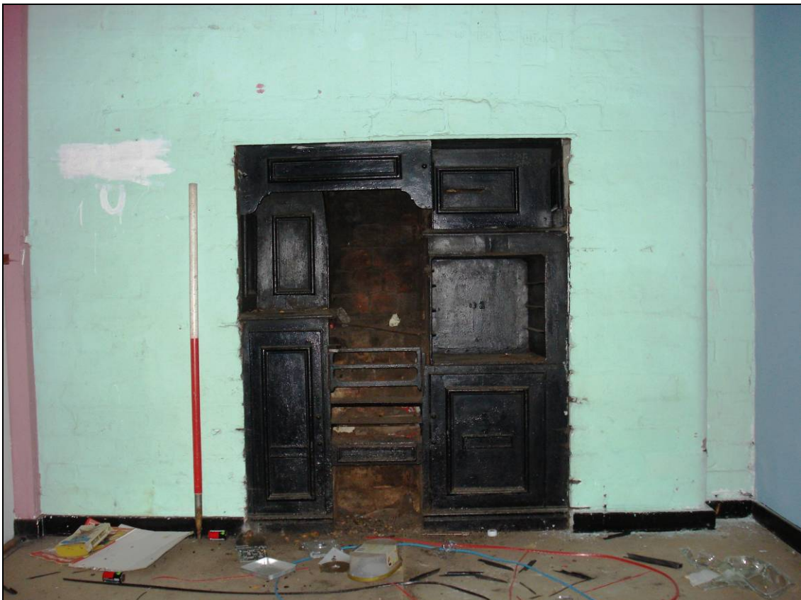
Figure 58: Cooking range within the western room of the ground floor, looking north (scale 1m)
