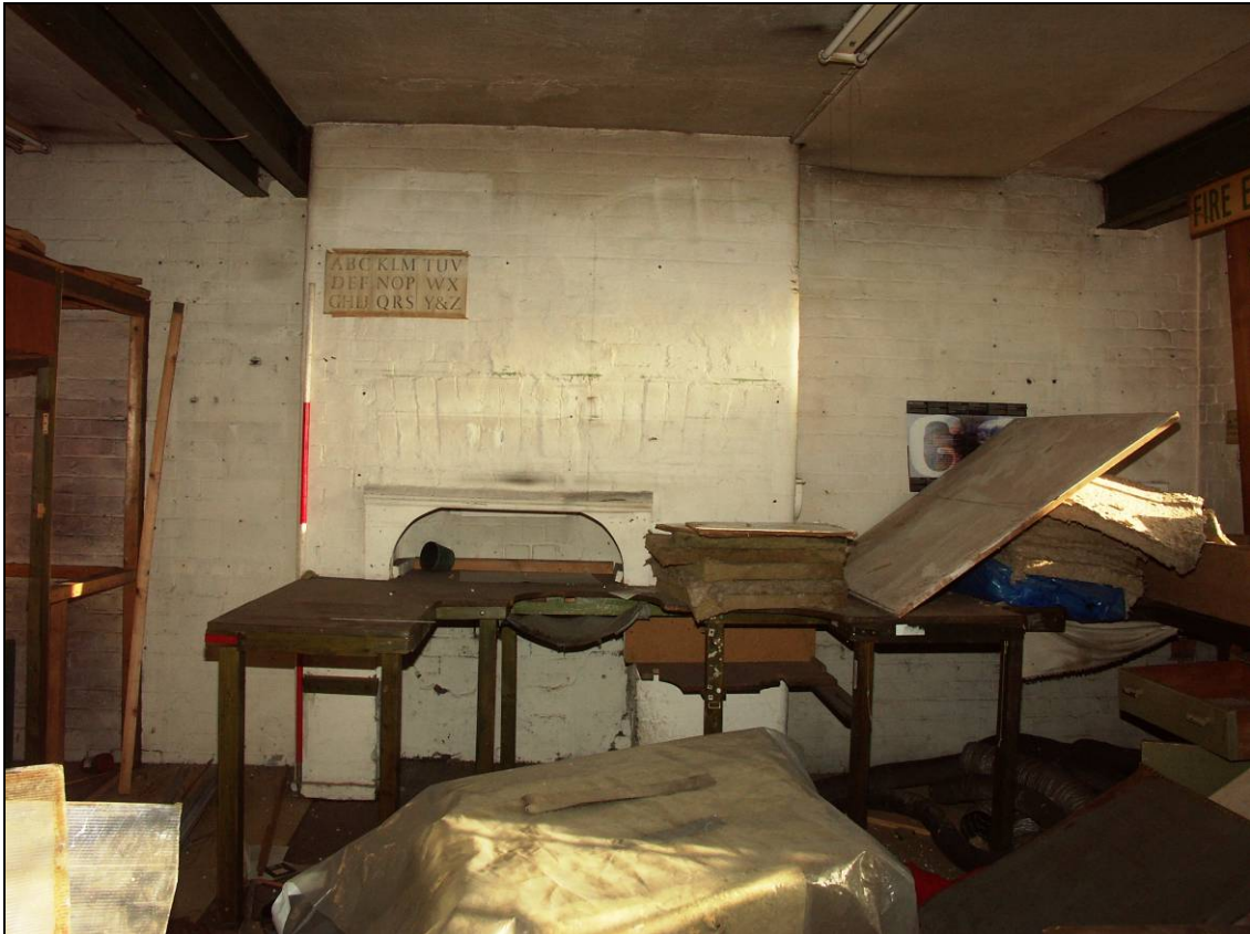
Figure 72: Chimney breast within the east end of the third floor (scale 2m)
