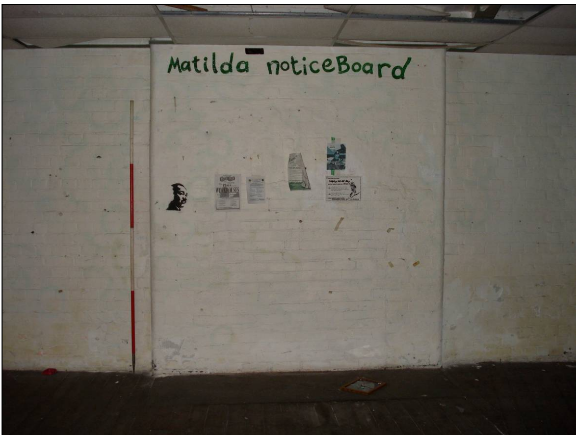
Figure 56: Chimney breast with blocked fire place along the central section of the east wall (scale 2m)
