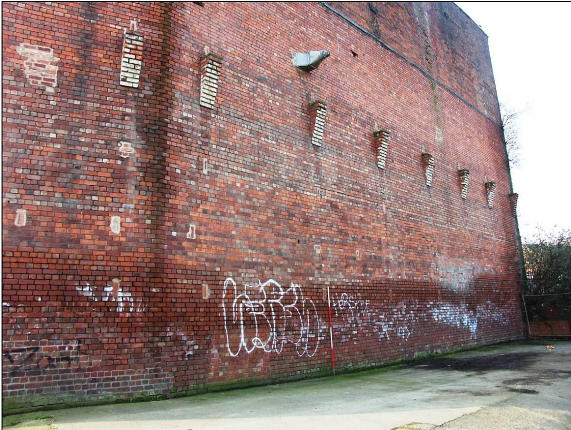
Figure 46: Detail of the north elevation facing the car park, looking west (scale 2m)
