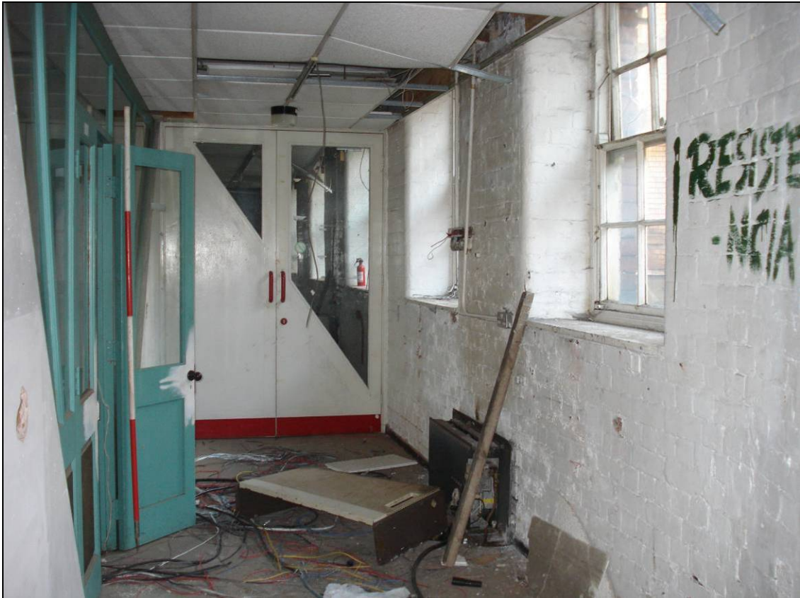
Figure 57: Western end of the ground floor of Building 2, looking east (scale 2m)
