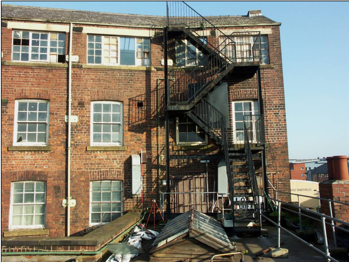
Figure 44: Fire exit staircase to the eastern end of the south elevation (scale 2m)
