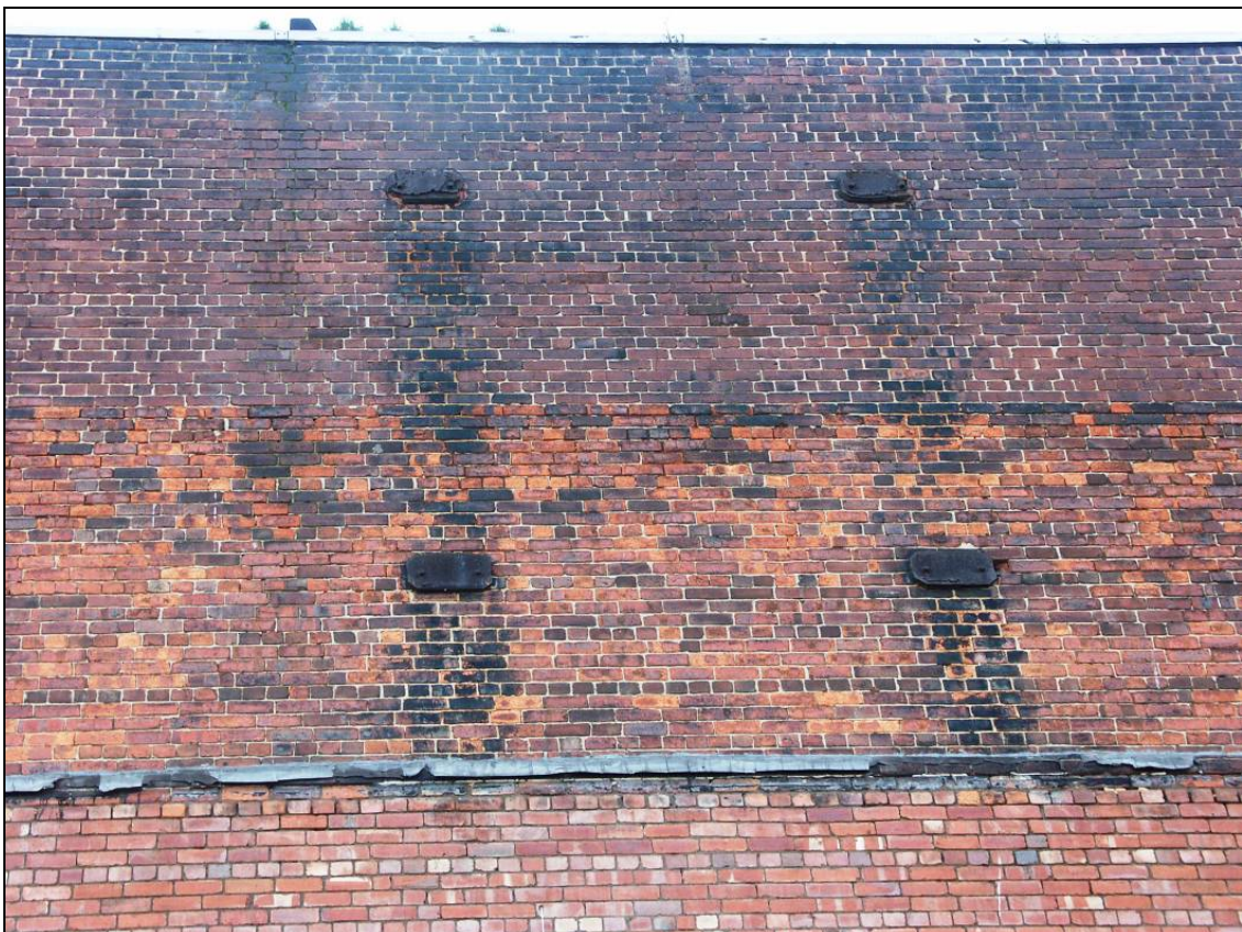
Figure 47: Detail of wall plates of internal RSJ stanchions within the upper storeys, looking south
