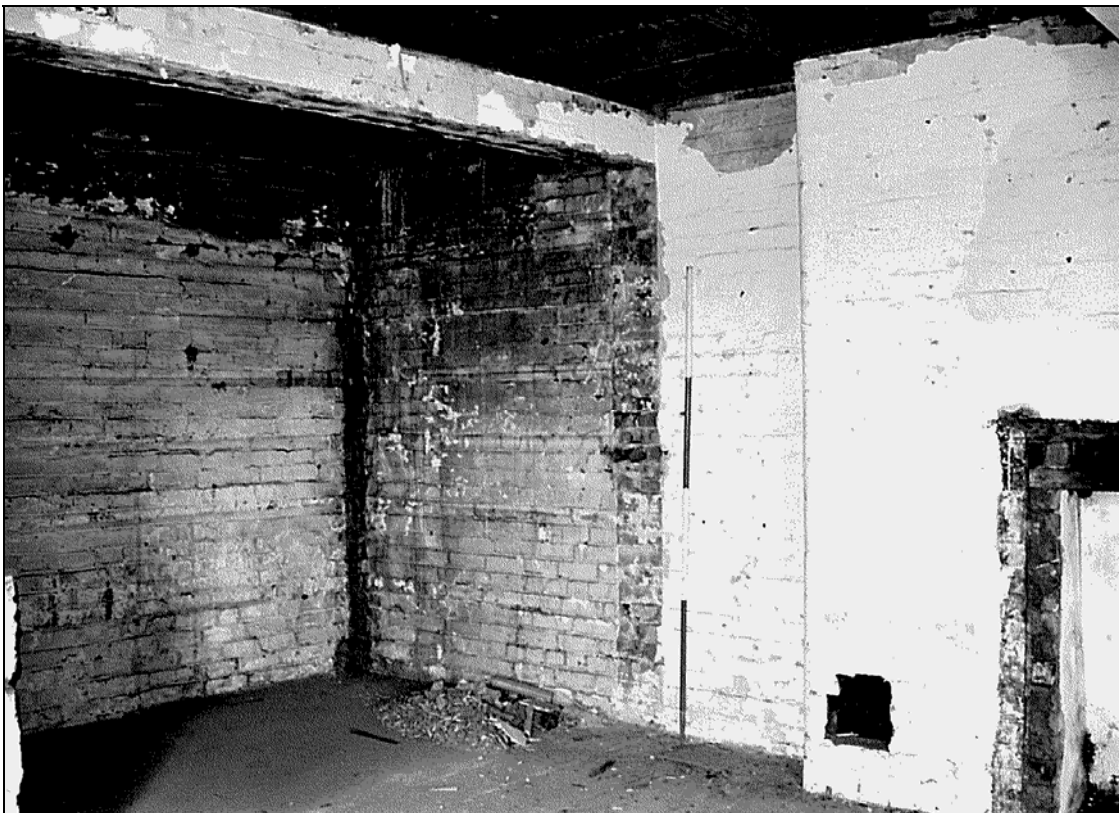
Figure 71: Internal view of the safe following demolition of partition wall, looking north-west (scale 2m)
