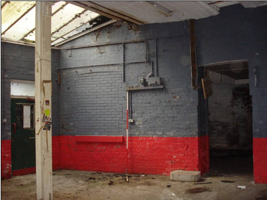
Figure 23: Northern room of the eastern wing leading into Building 2, looking north (scale 2m)
