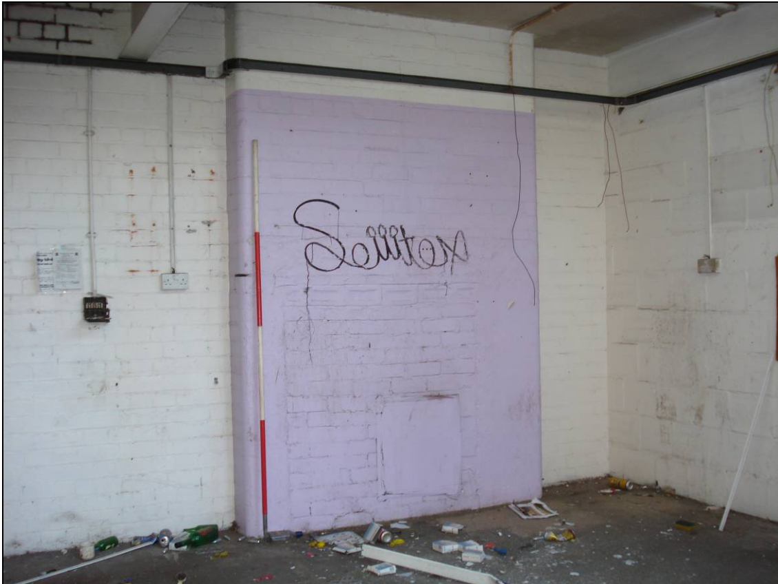
Figure 37: Chimney breast within the north end of the eastern wing, looking east (scale 2m)
