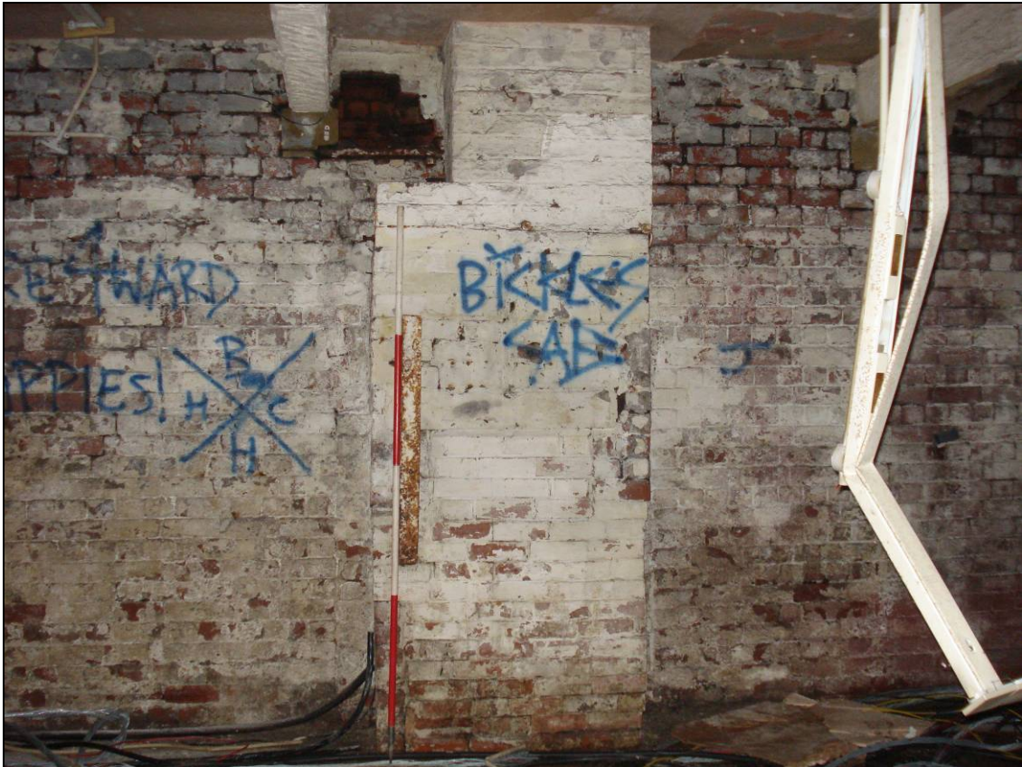
Figure 52: Central chimney breast along the north wall of the basement (scale 2m)
