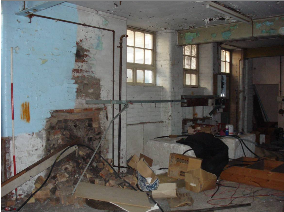
Figure 24: Ground floor of the southern wing with fire place, looking north-east (scale 2m)
