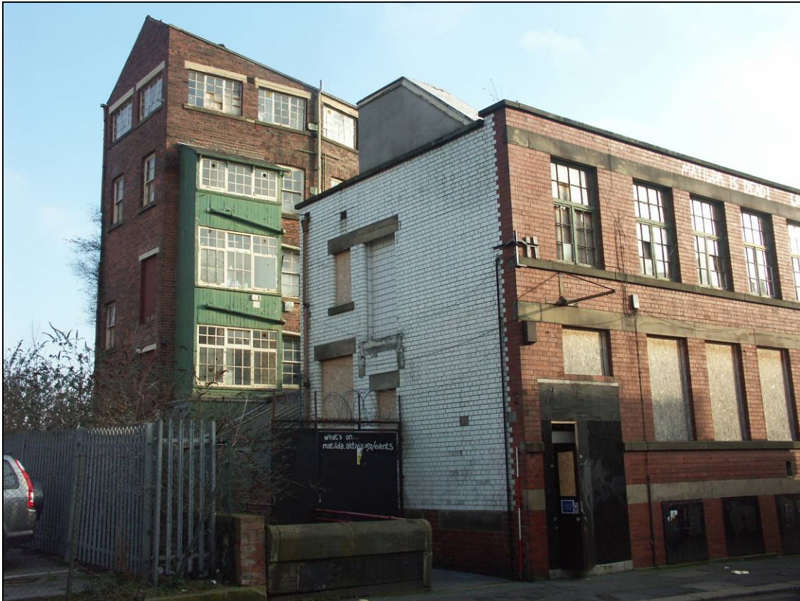
Figure 6: West elevation of the southern wing facing to the Porter Brook, looking north-east (scale 2m)
