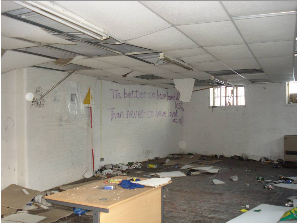
Figure 60: General view of the first floor of Building 2, looking west (scale 2m)
