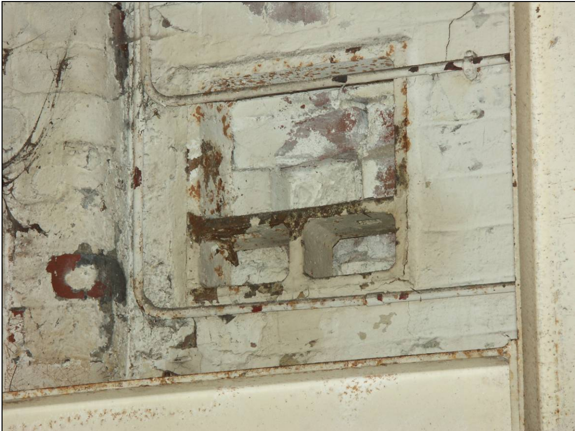
Figure 19: Detail of bearing housing within the partition wall to the electrical switch board, looking north
