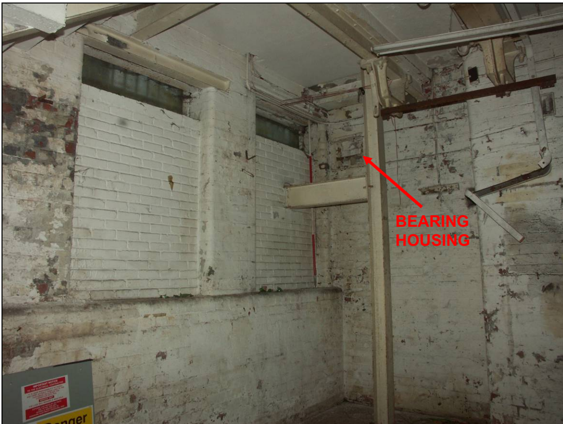
Figure 18: Blocked windows along the Porter Brook and former bearing housing within adjacent wall
