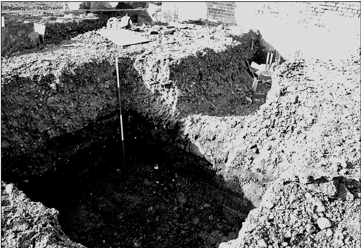
Figure 5: Foundation trench within the south-western area of the site, looking west (scale 2m)
