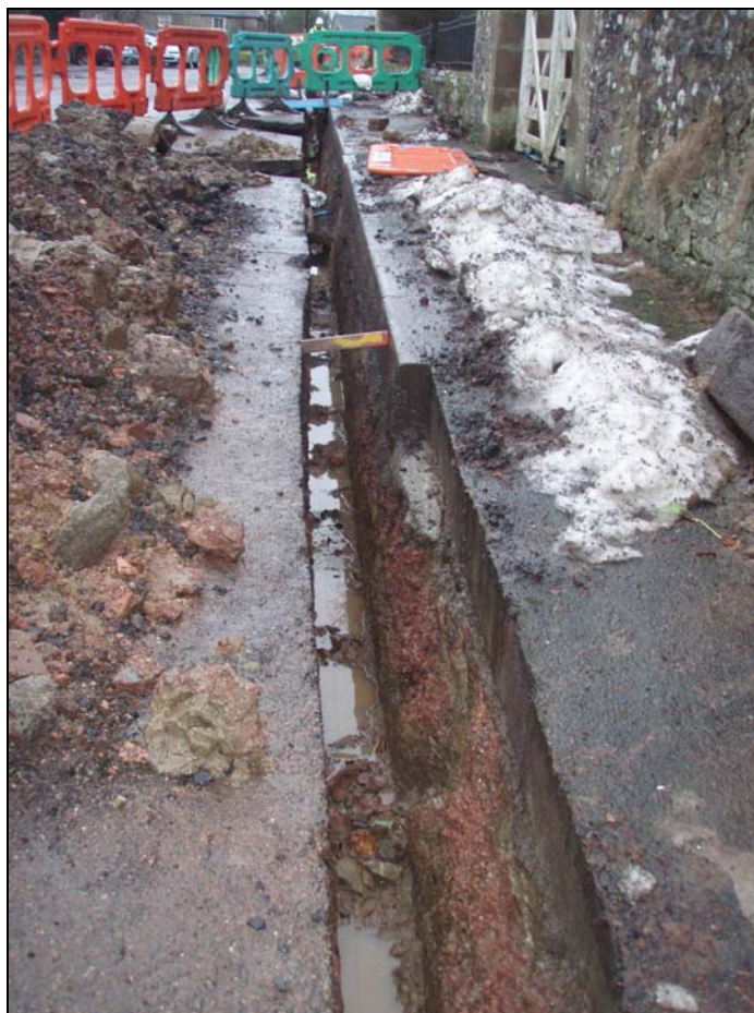
Figure 5: The service trench running from north to south through the centre of the village.
