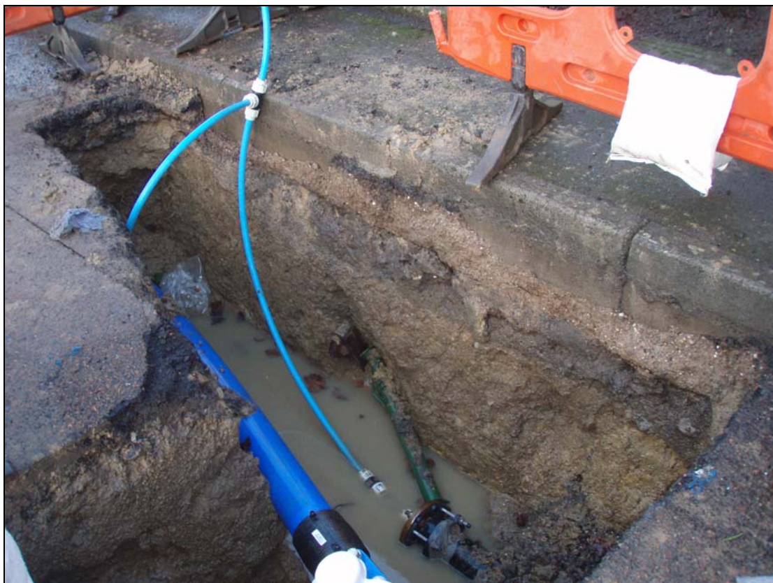
Figure 3: One of the service trenches showing the various layers of road makeup.
