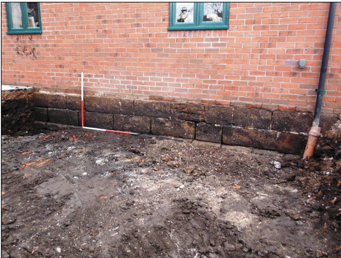
Figure 10: Excavated central area exposing further stone wall, looking south (scale 2 x 1m)
