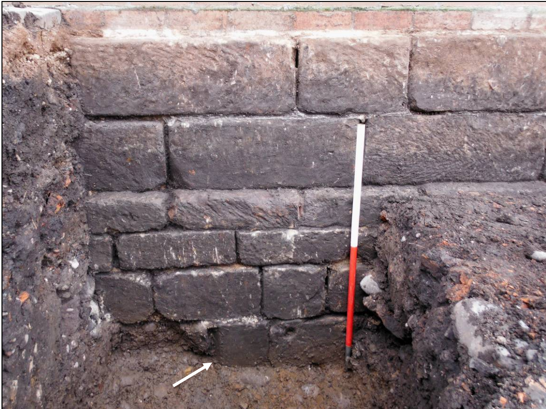
Figure 9: Foundation wall (307) with reused chamfered fragment indicated by an arrow (scale 1m)
