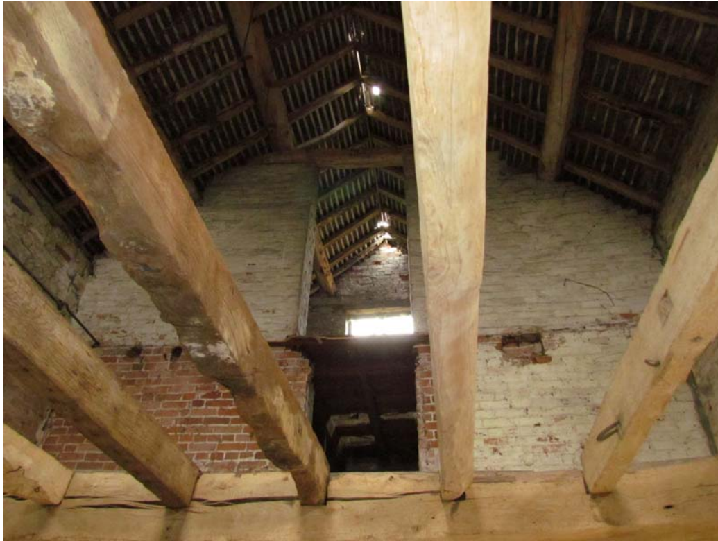
Figure 33: View of Internal Wall at Bin and Loft Floor Level, Looking South.
