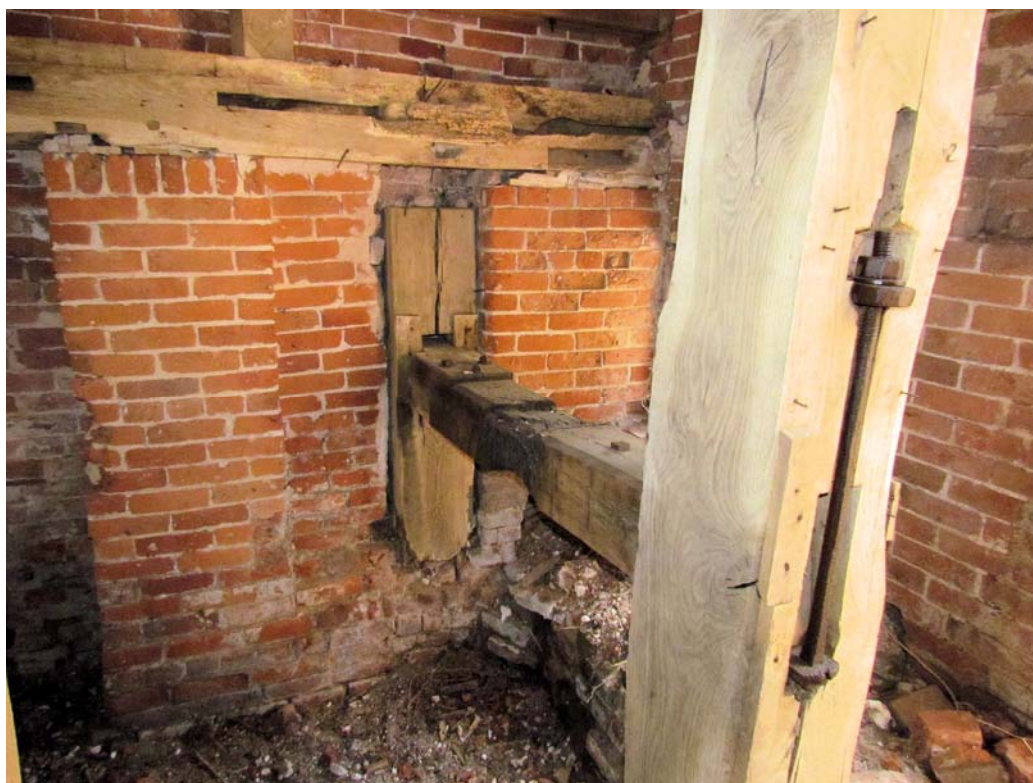
Figure 24: Detail of Hurst Structure for South Wheel Gearing and Structural Beam, Looking South.
