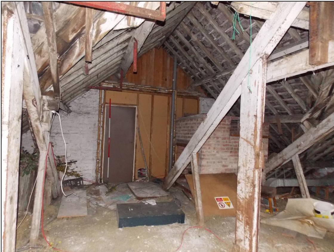
Figure 72: Loft with a doorway to the adjacent Building B, looking north (scale 2m).
