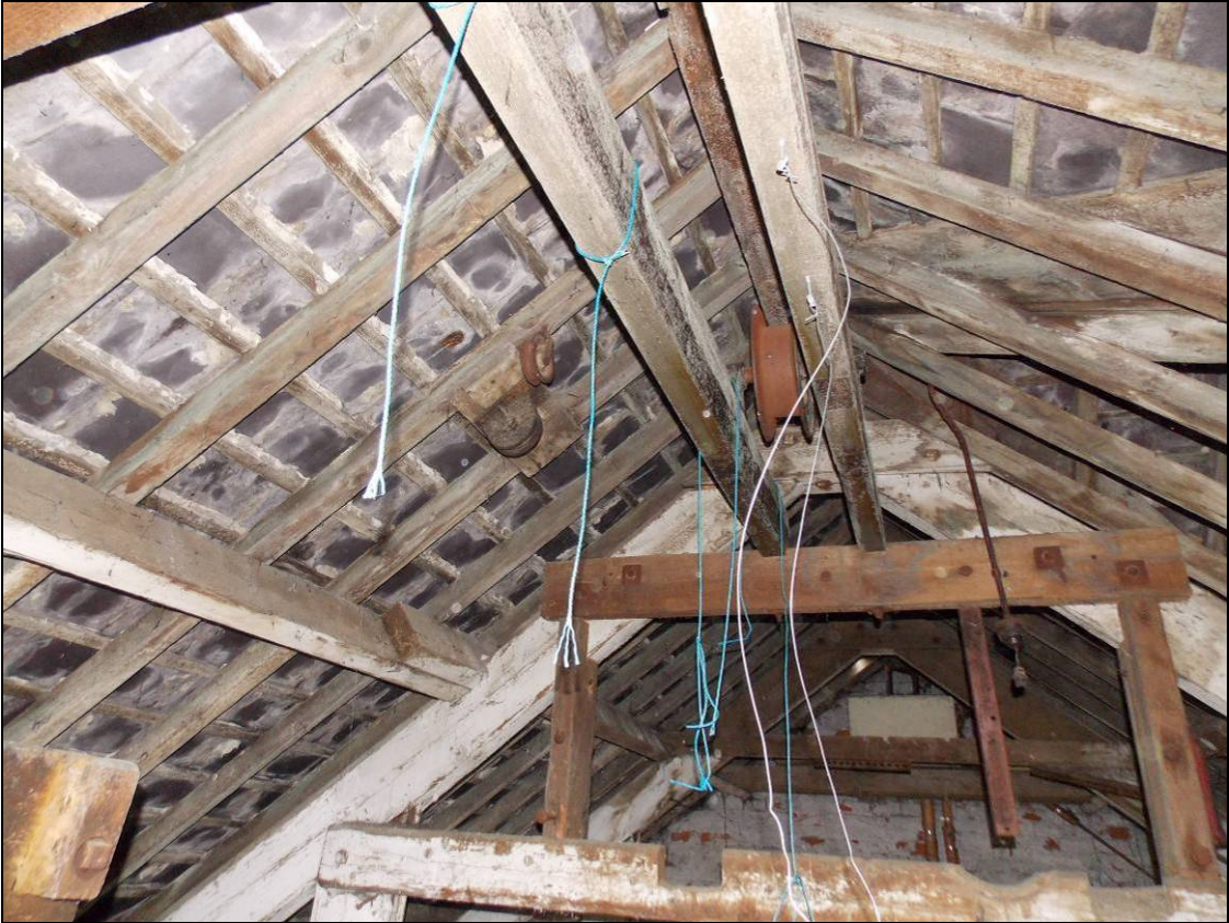
Figure 79: Central pulley wheel and additional smaller wheels attached to common rafters, looking east.
