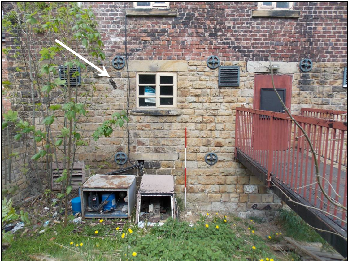
Figure 18: Scars of former pitched extension and sawn-off side purlin (arrow) (scale 2m).
