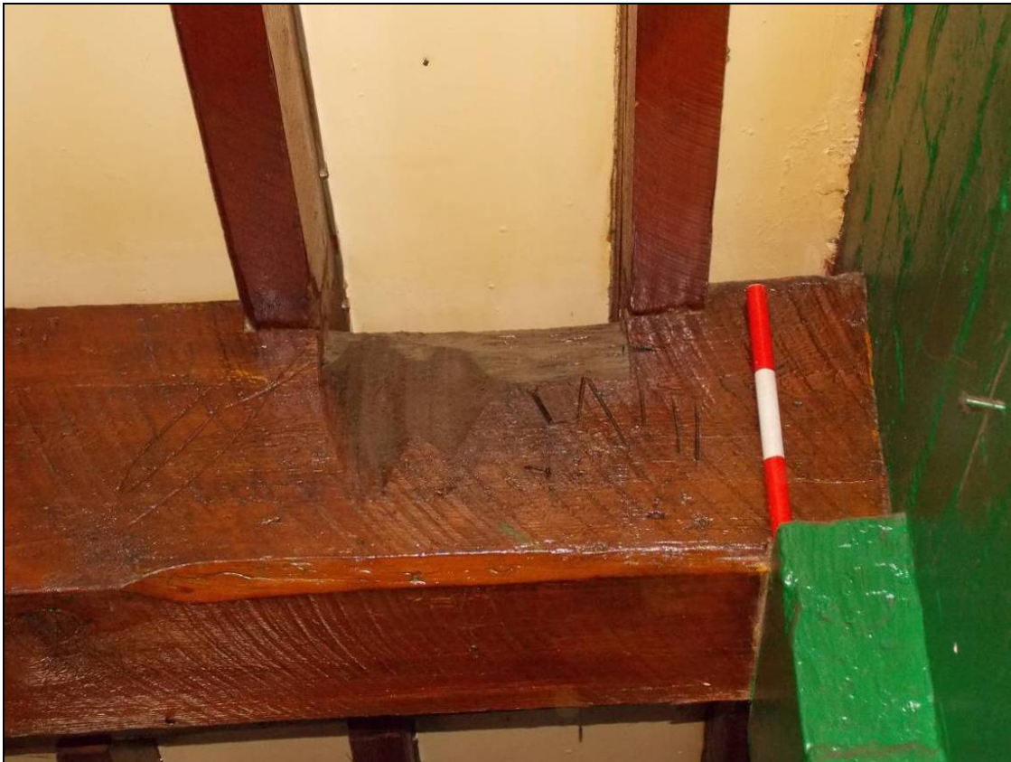
Figure 132: Northern end of the eastern beam with carpenter's mark and later grooves (scale 300mm).
