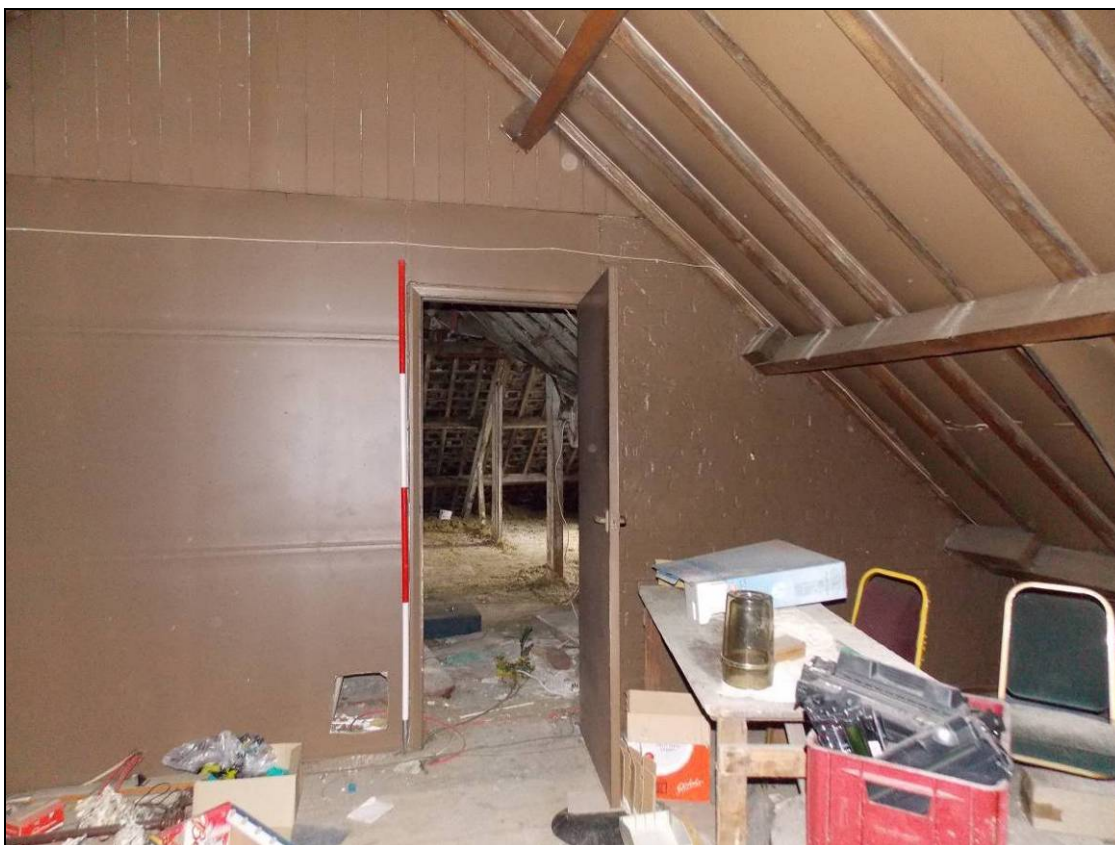
Figure 146: Southern bay with doorway to the adjacent Building A, looking south (scale 2m).
