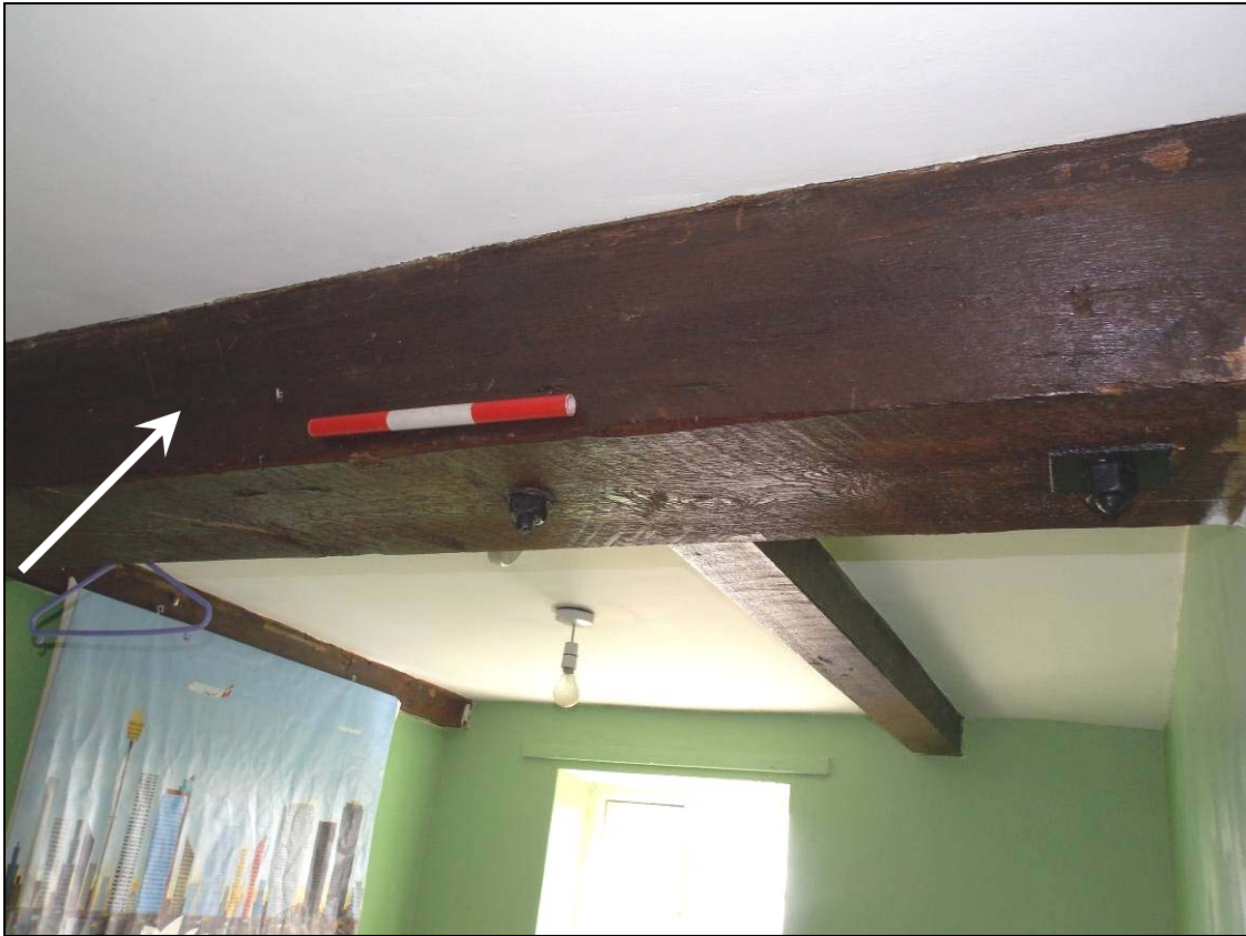
Figure 65: Eastern tie-beam with carpenter's marks (arrow) and trimmer beams, looking east (scale 300mm).
