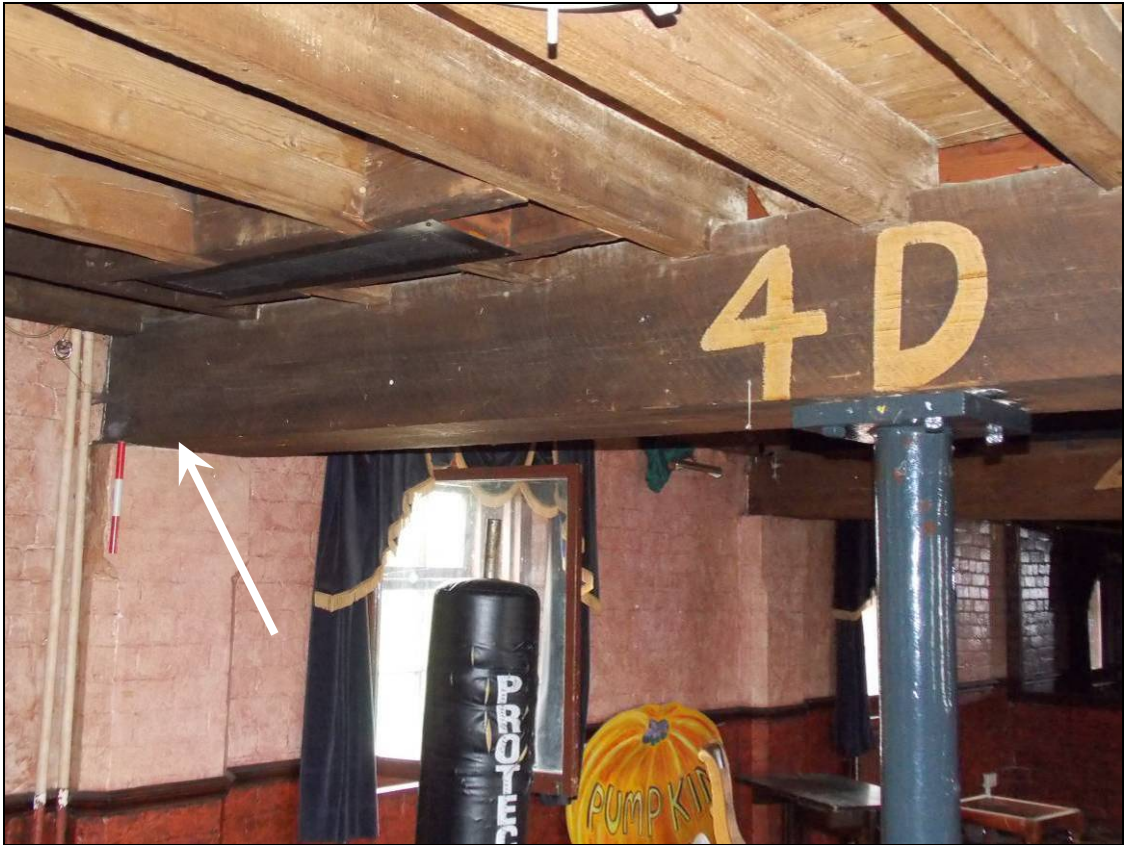
Figure 140: Western side of the southern tie-beam with carpenter's marks (arrow) (scale 300mm).
