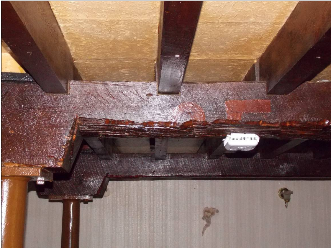
Figure 36: Carpenter's marks over the southern column of the central beam, looking east.
