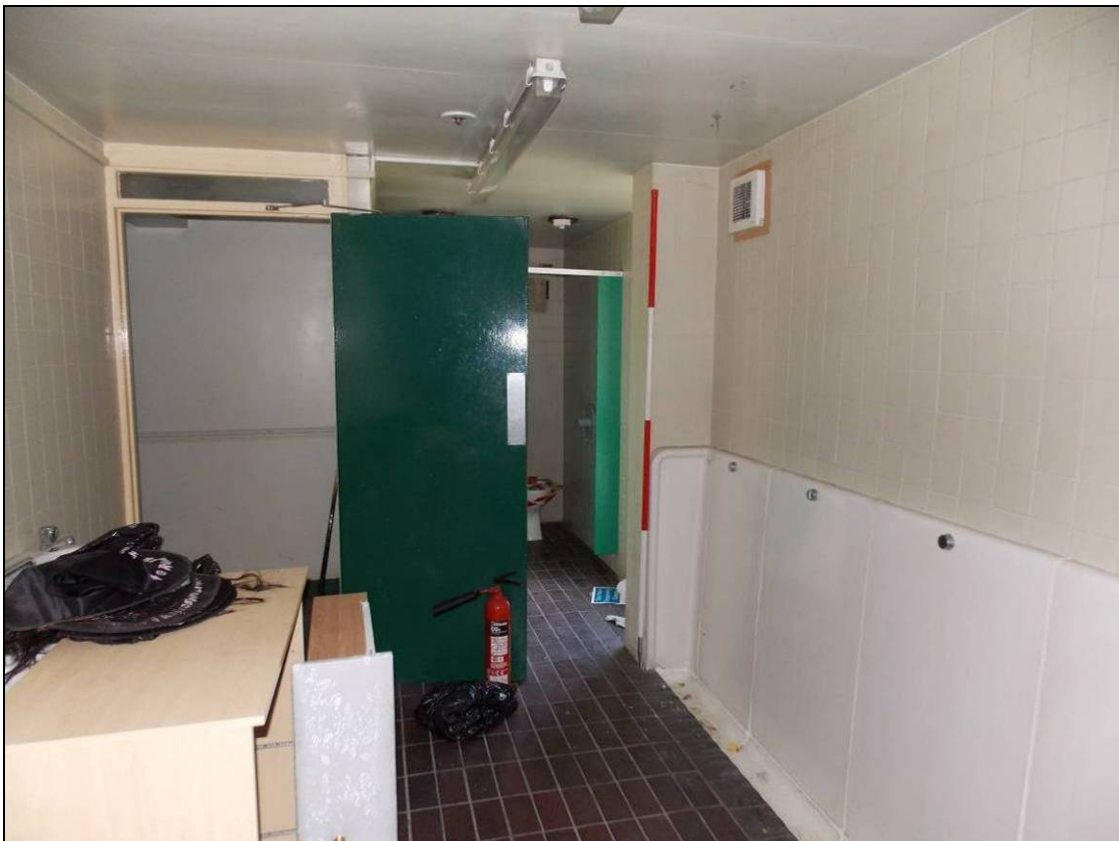
Figure 173: Gents lavatory within the first floor of Building D, looking west (scale 2m).
