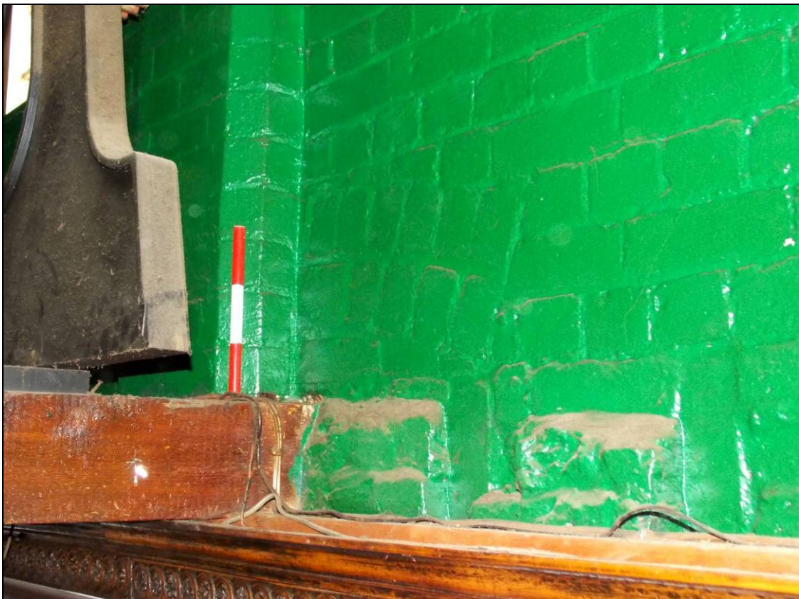
Figure 128: Segmental arched head partially obscured by later pilaster, looking north-east (scale 300mm).
