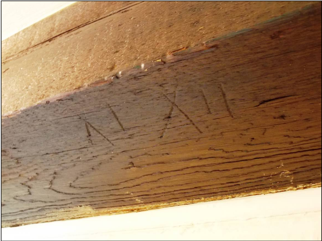
Figure 61: Carpenter's marks within the central tie-beam and adjacent to the southern through bolt.
