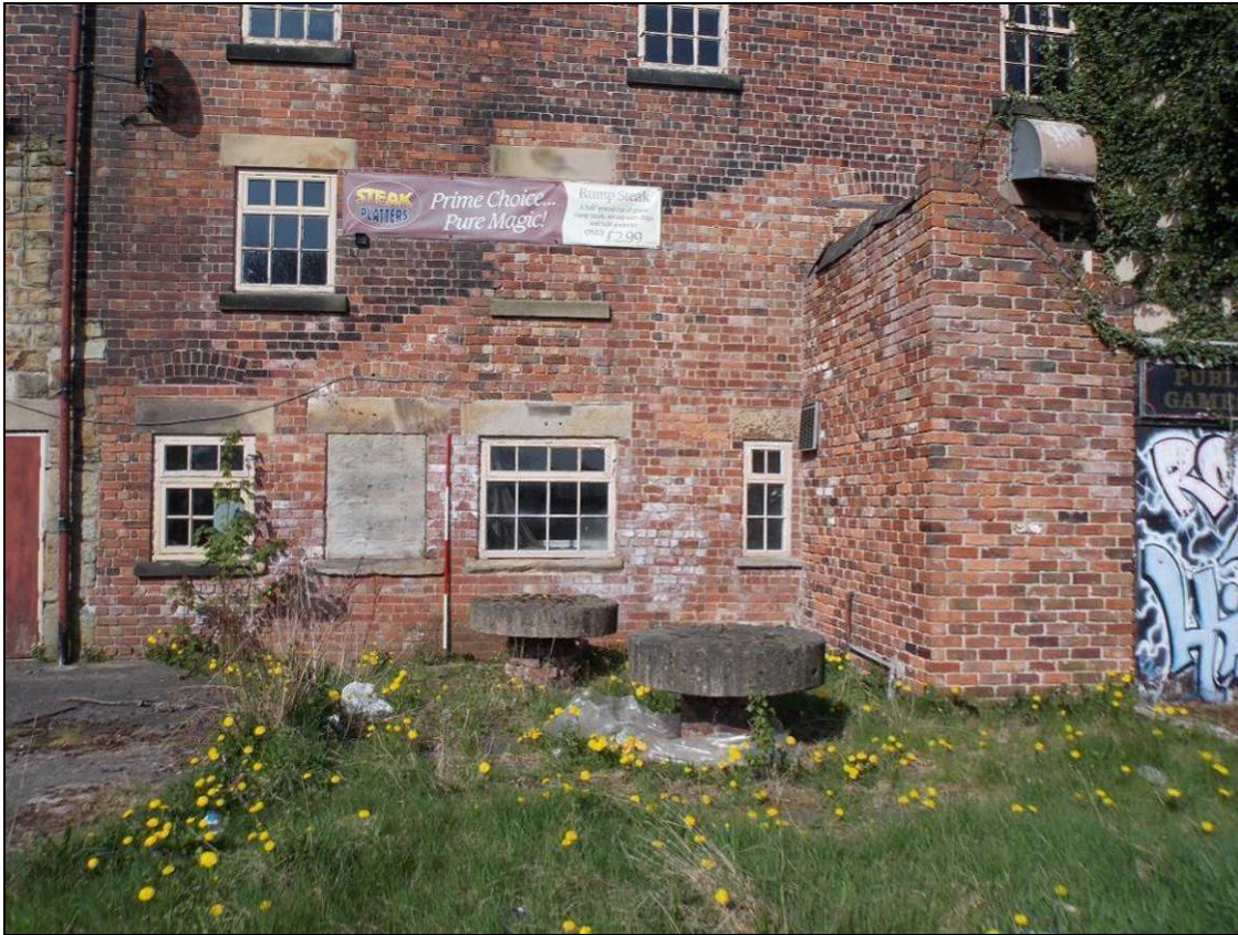
Figure 83: Scar of former pitched extension and remnants of earlier openings (scale 2m).
