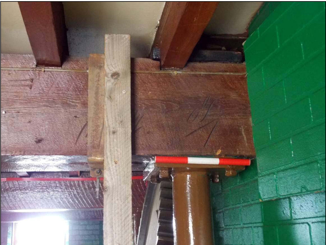
Figure 123: Carpenter's marks within the western beam and above the southernmost column (scale 300mm).
