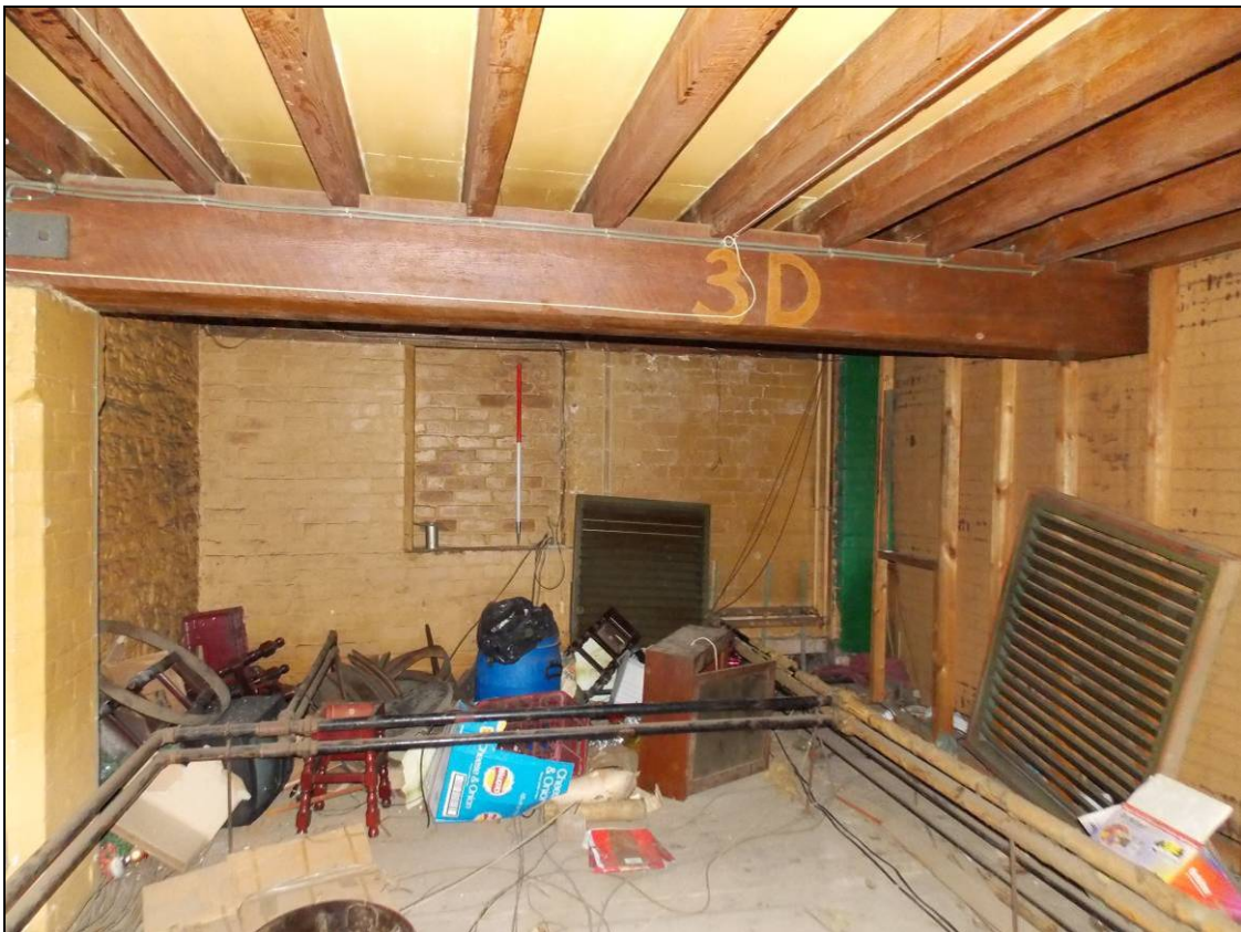
Figure 115: Southern bay of the first floor with blocked-up window opening within the west wall (scale 1m).
