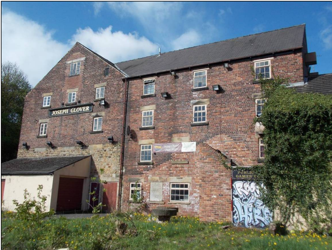
Figure 82: East elevation of Building B (right) abutting the gabled wall of Building A (left) (scale 2m).
