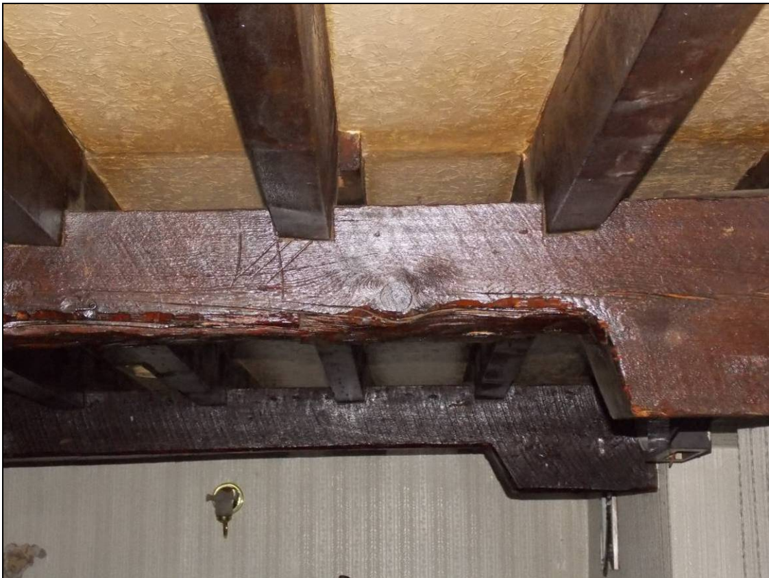
Figure 37: Carpenter's mark within the southern section of the central beam, looking east.
