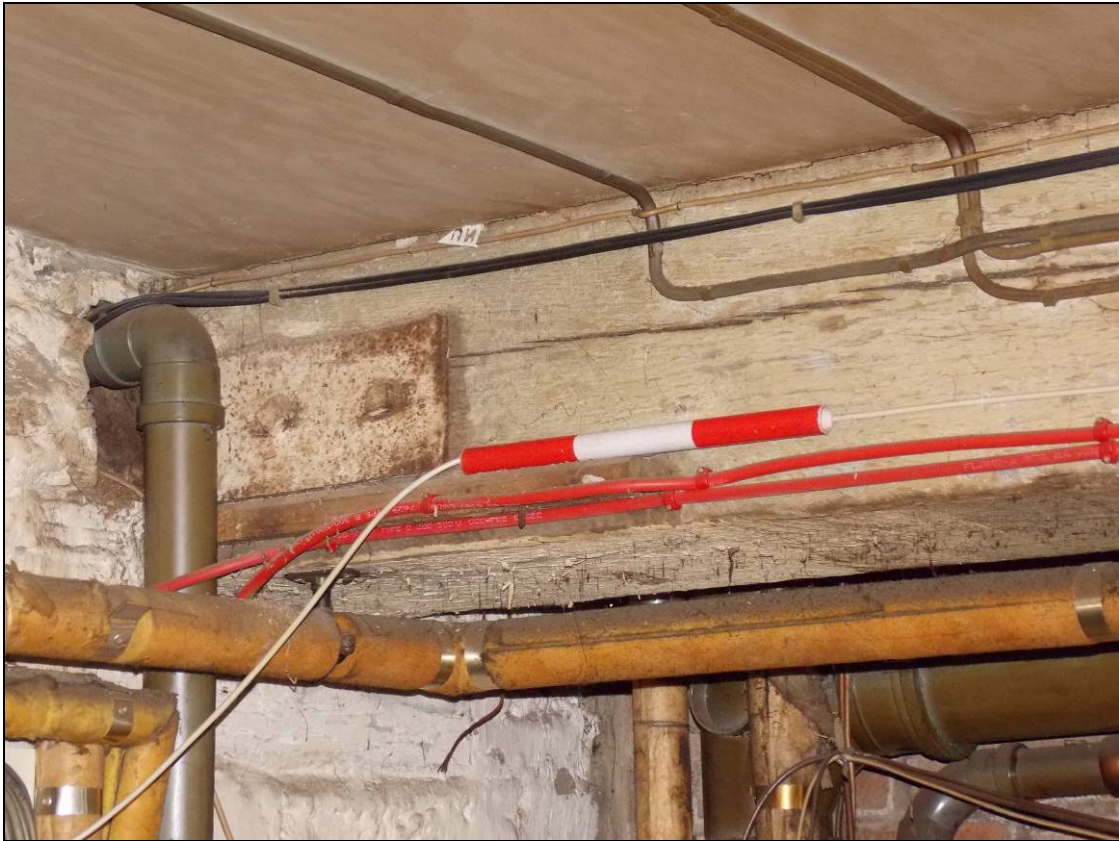
Figure 48: Plate attaching longitudinal beams of Buildings A and B, looking north-east (scale 300mm).
