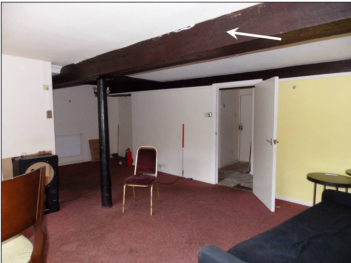
Figure 69: Room S7 with tie beam containing carpenter's marks (arrow), looking north-east (scale 1m).
