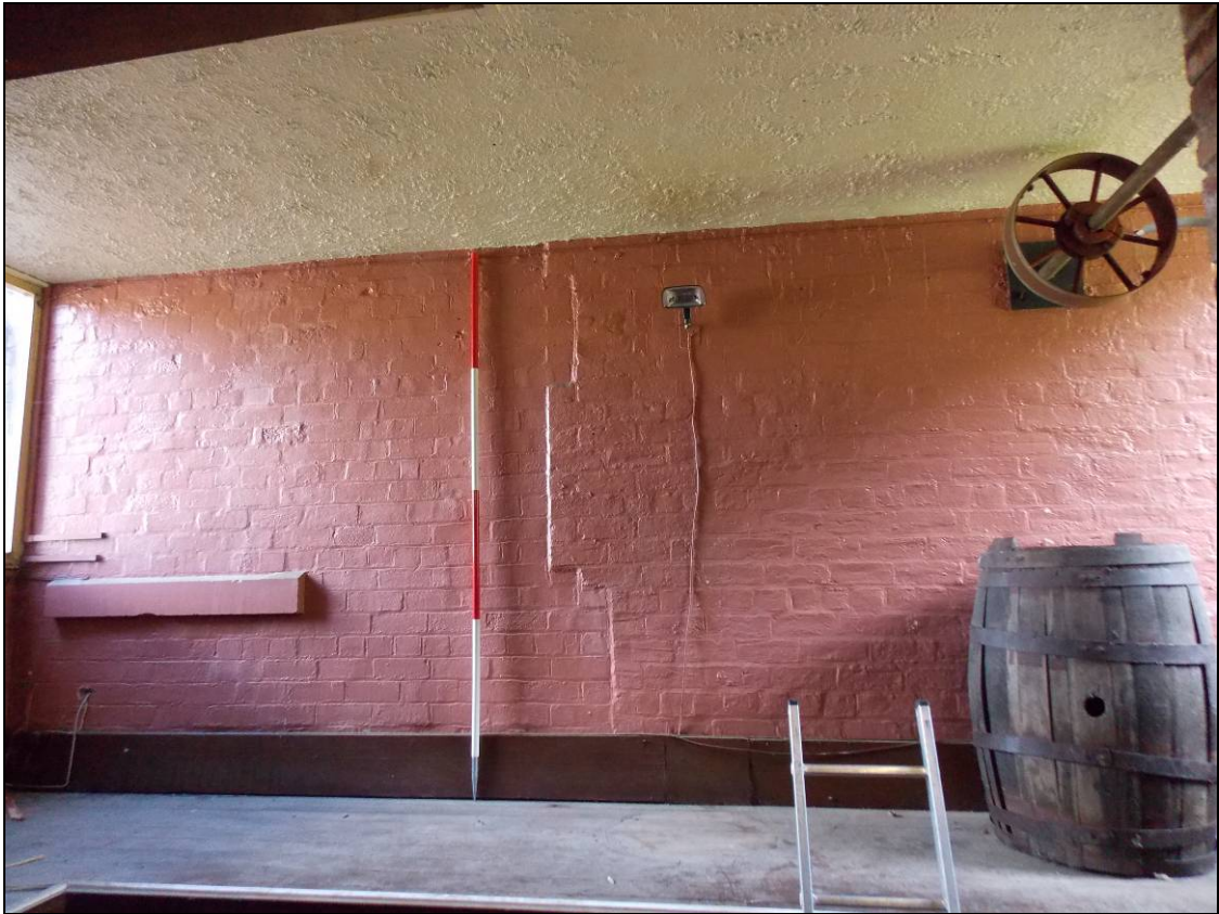
Figure 89: Blocked-up window opening and decorative drive belt within the first floor of Building B (scale 2m).
