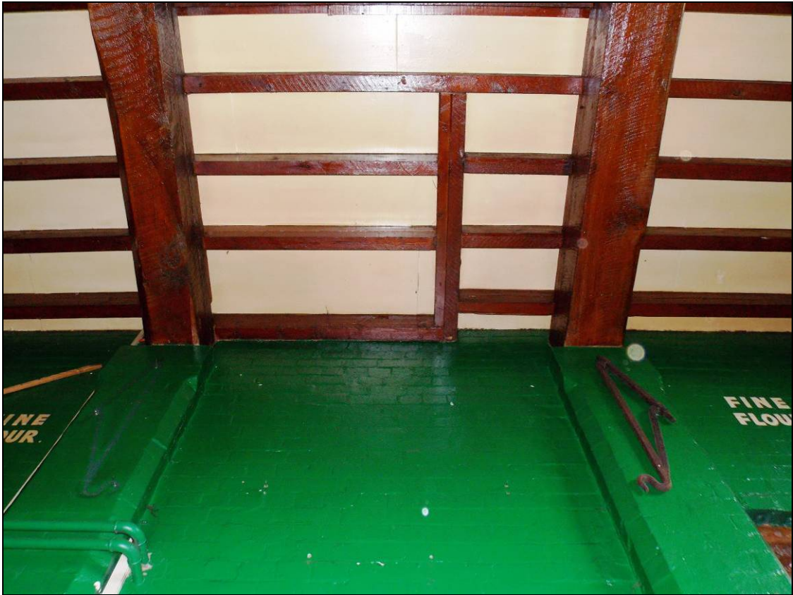
Figure 133: Trimmer beam within the northern end of the central bay, looking north.
