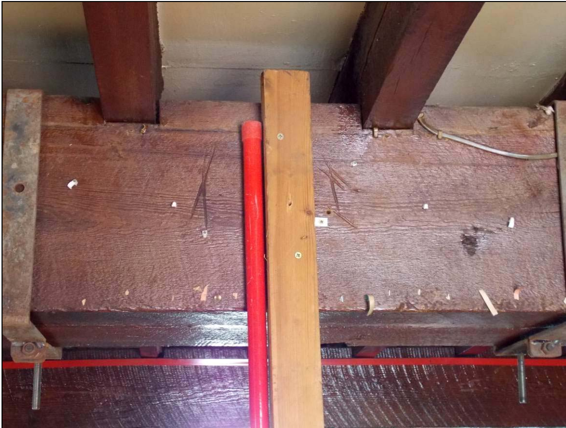
Figure 124: Carpenter's marks within the western beam between the central and southernmost columns.
