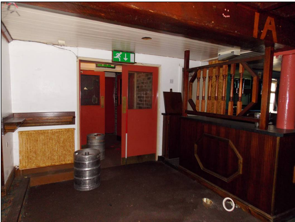
Figure 95: Main doorway to the basement within the west wall, looking west (scale 1m).
