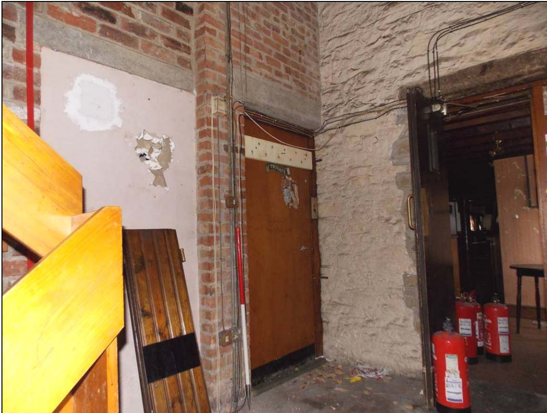
Figure 40: Lift (left) and inserted doorway (right) to the adjacent Building B, looking north (scale 1m).
