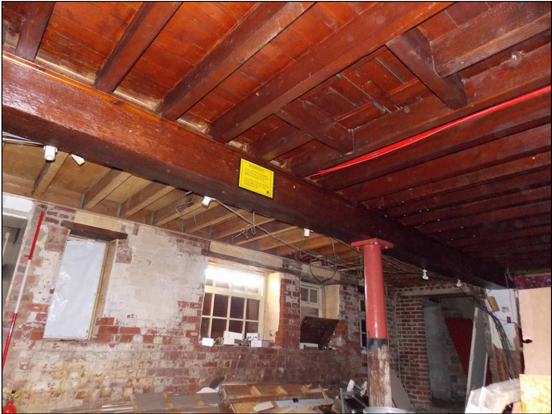
Figure 100: Basement with ceiling hatch adjacent to the bar (dismantled following soft-stripping).
