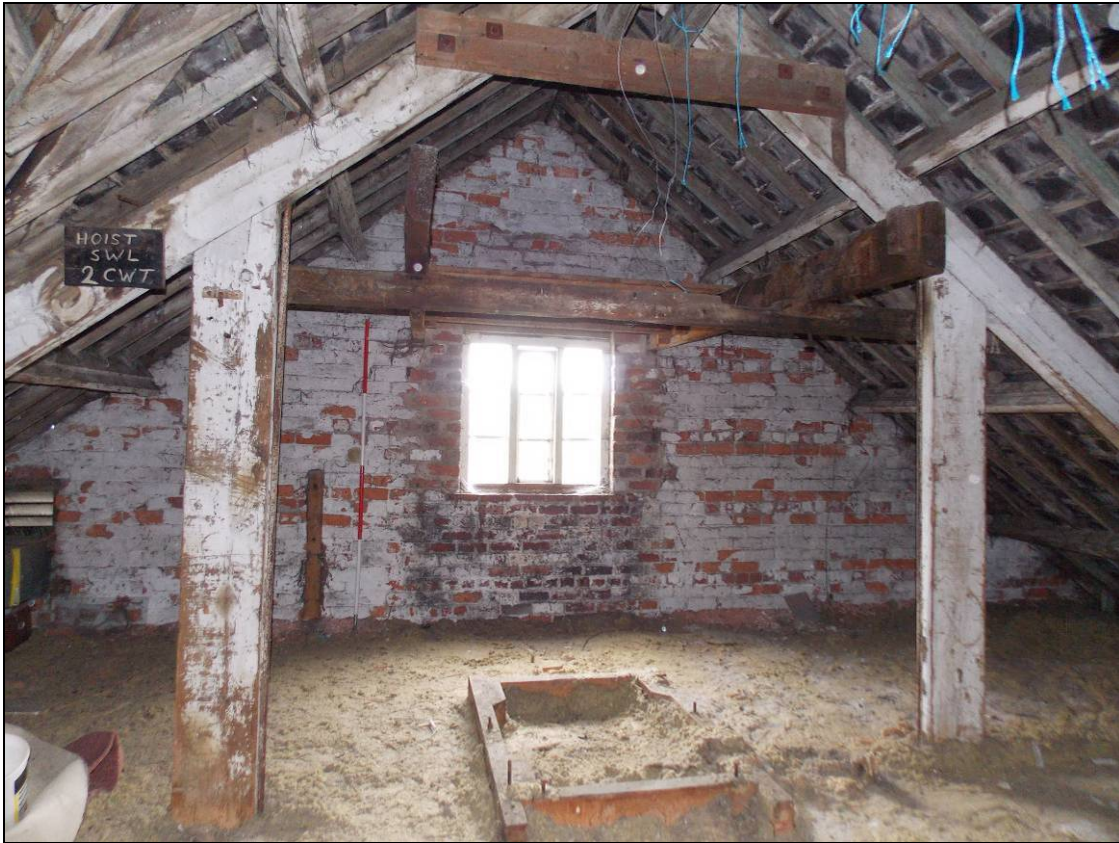
Figure 77: Eastern truss I with upper collar for central pulley wheel's joists (scale 2m).
