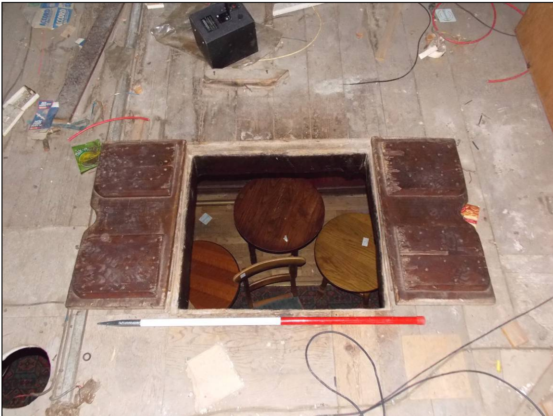
Figure 44: Hatch with doors open down to the ground floor, looking north (scale 1m).
