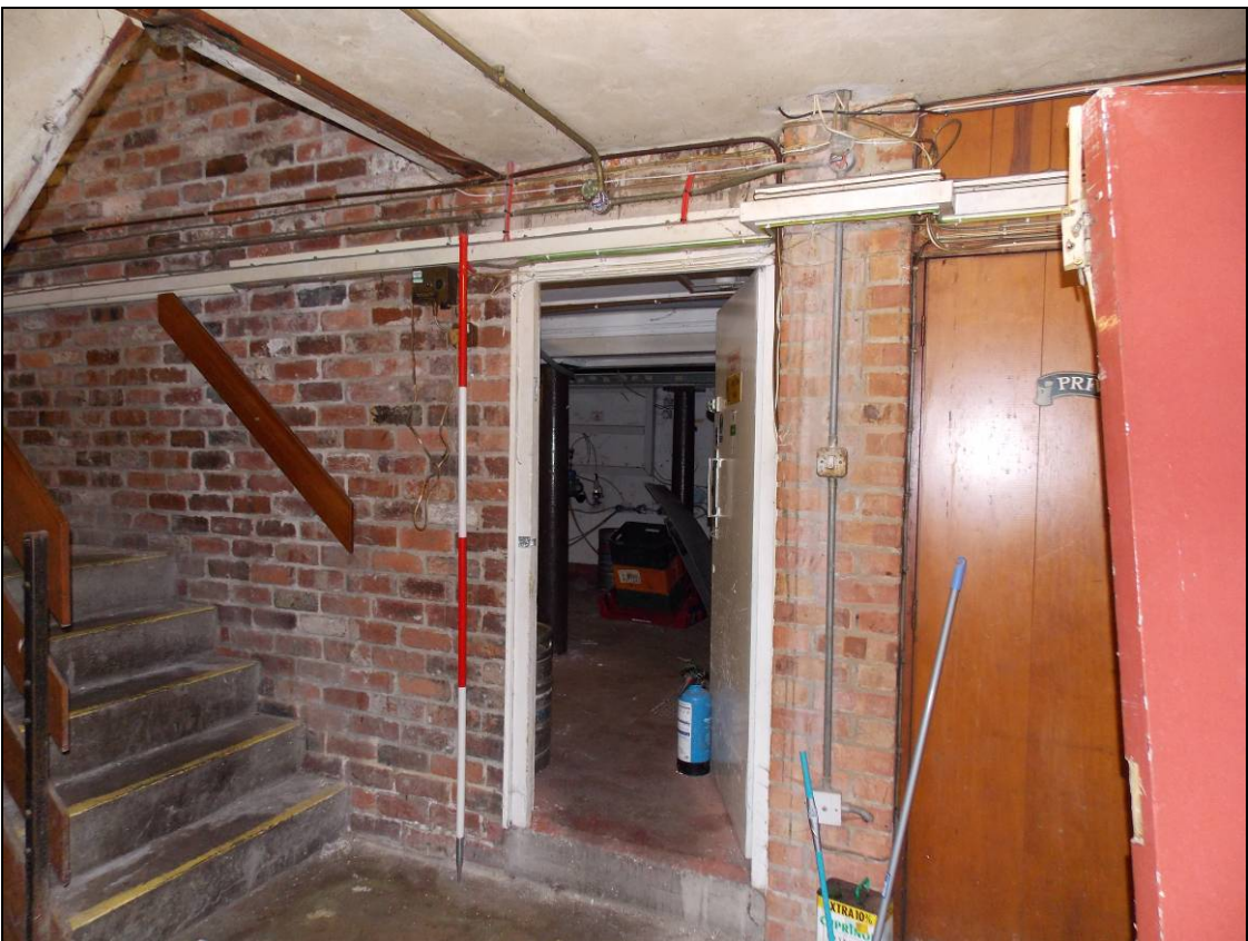
Figure 21: Doorway to the beer cellar (left) and lift (right), looking west (scale 2m).
