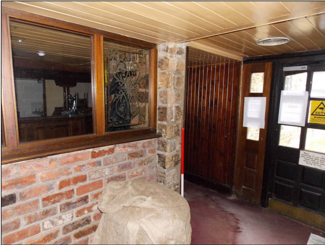
Figure 13: Northern section of the ground floor of the west elevation, looking south-east (scale 1m).
