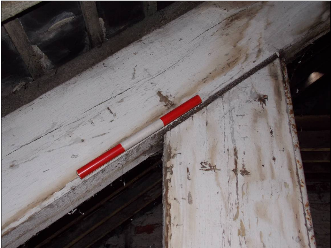
Figure 75: Detail of carpenter's assembly marks within the western truss III, looking west (scale 300mm).
