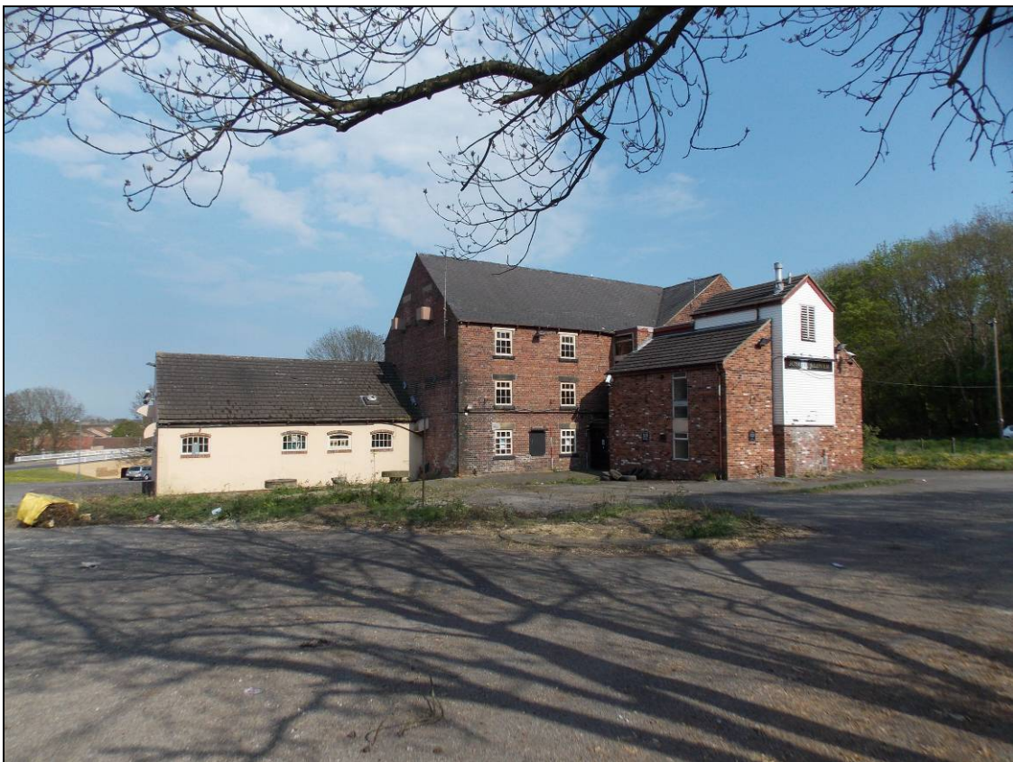
Figure 86: West elevation of Building B abutted by Buildings C (left) and D (right) (scale 2m).
