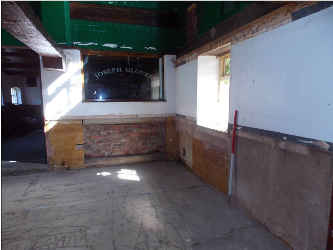
Figure 109: Former opening within the north wall revealed during the soft-stripping watching brief (scale 1m).
