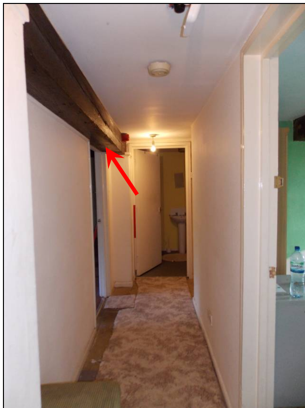
Figure 62: S3 with central beam containing carpenter's marks adjacent to the northern bolt (arrow) (scale 1m).
