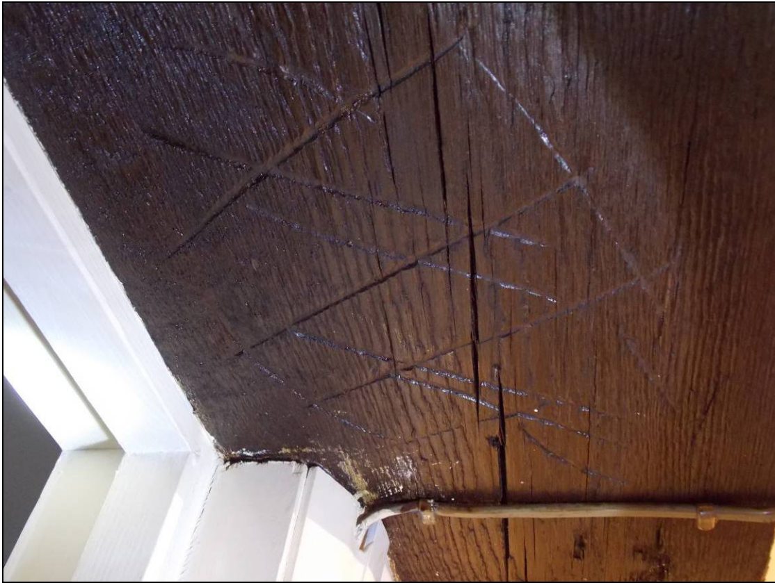
Figure 63: Carpenter's marks within the central tie-beam and adjacent to the northern through bolt.
