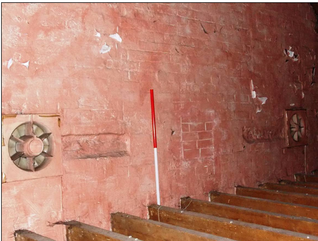
Figure 145: North gabled wall containing window openings blocked with bricks, looking north-east (scale 1m).
