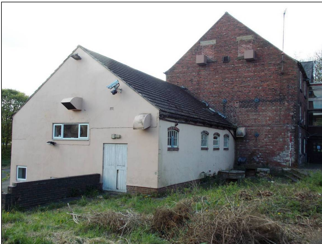
Figure 148: North and west elevations of Building C abutting Building B to the left (scale 2m).
