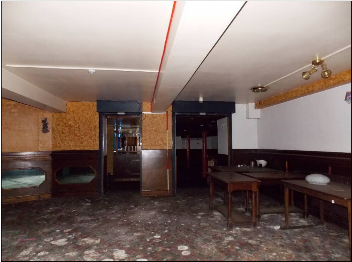
Figure 153: Snooker room within the basement of Building C, looking south (scale 2m).
