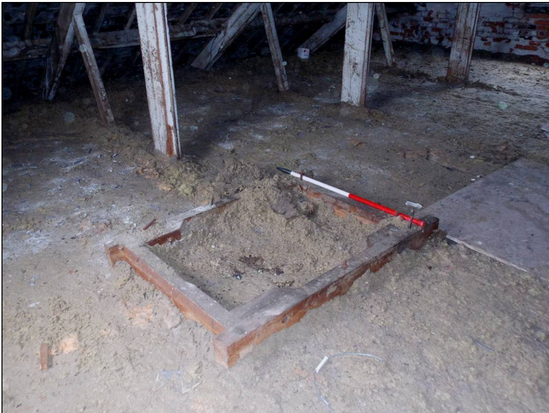
Figure 78: Frame of former hatch beneath the central pulley wheel, looking south-west (scale 1m).
