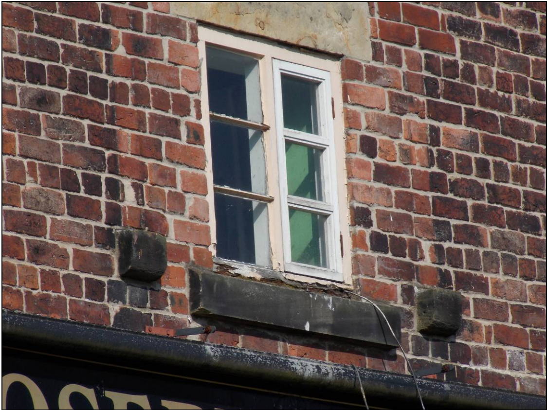
Figure 9: Detail of corbels flanking the central window sill of the second floor.
