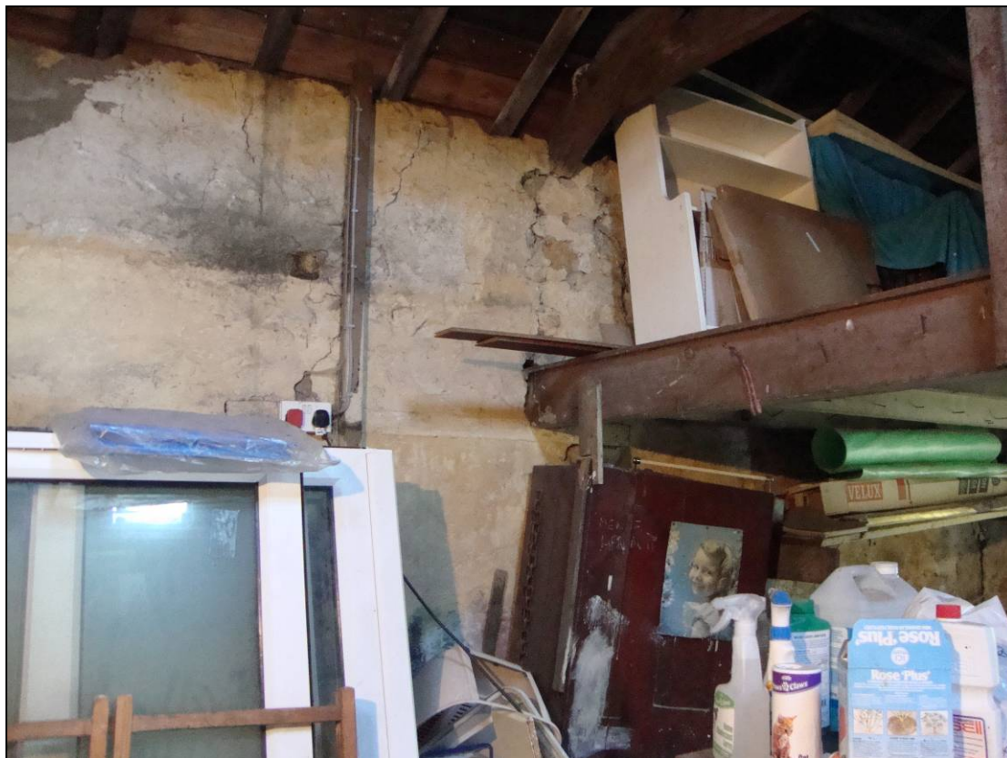
Figure 5. Internal view of the former farm building showing inserted mezzanine floor and structural defects in main wall.
