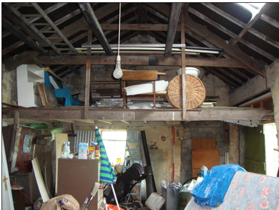
Figure 10: South wall of Room A1, Building A, including inserted mezzanine floor and blocked door opening. (scale=2m).
