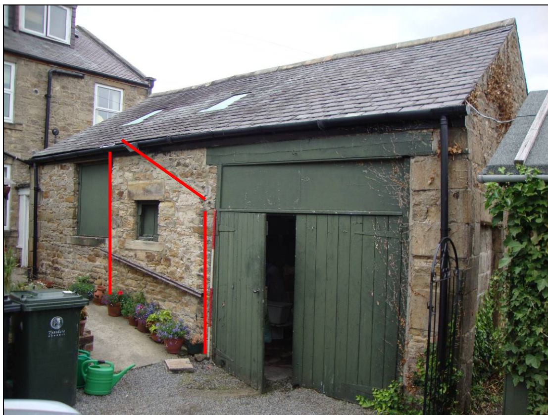
Figure 5: West elevation of Building A, showing position of join to later brick building, now removed, as indicated by red lines (scale=2m).
