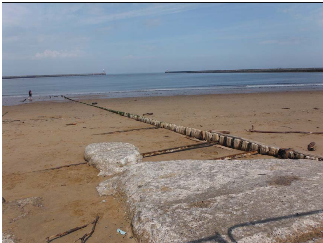
Figure 6. South-east view of seaplane ramp, showing close up view of overlain concrete
