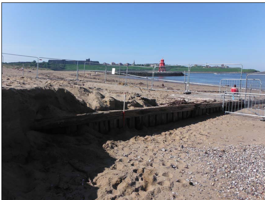
Figure 7. Northern view of seaplane ramp, highlighting vertical wooden beams overlain with horizontal beams. Scale = 1m.
