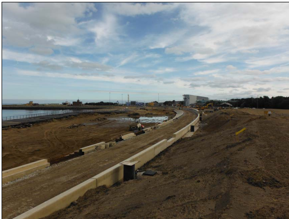
Figure 15. Southern view of site, showing old sea wall on the left and construction of new sea wall in centre of shot.
