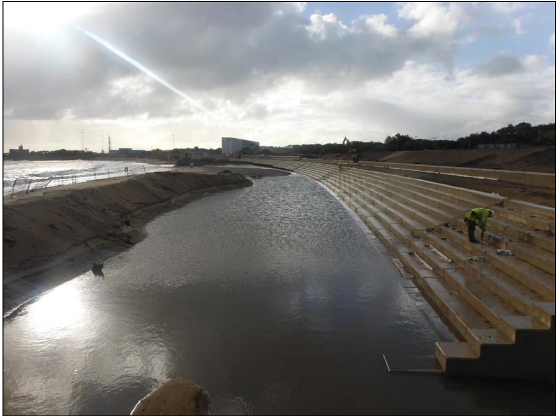
Figure 17. Southern view of site, showing old sea wall removed (on left) and new sea wall (on right).
