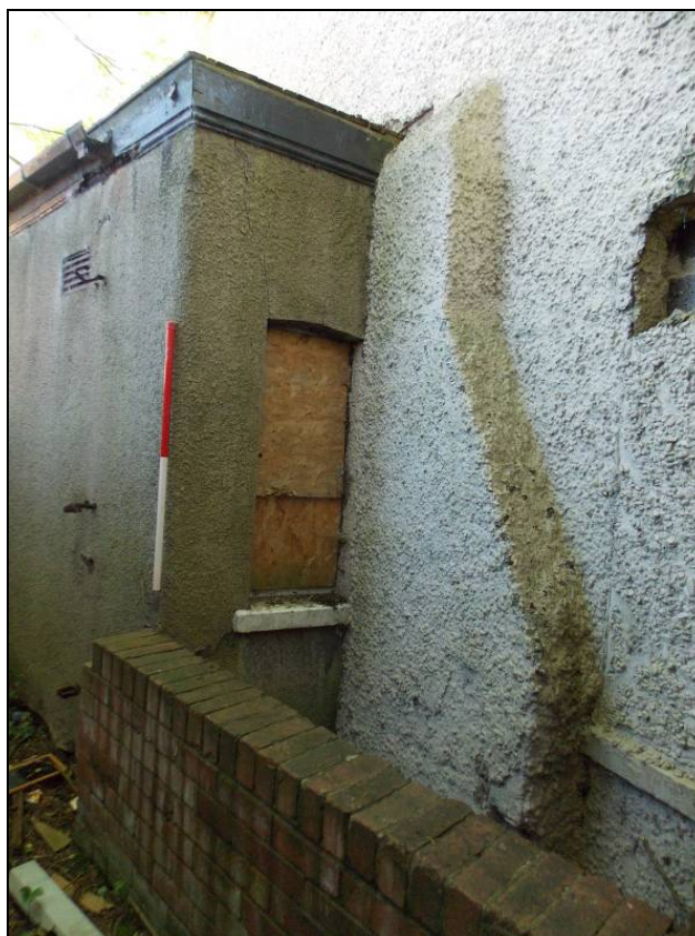
Plate 6: North elevation with truncated chimney stack and additional extension, looking east (scale 1m)
