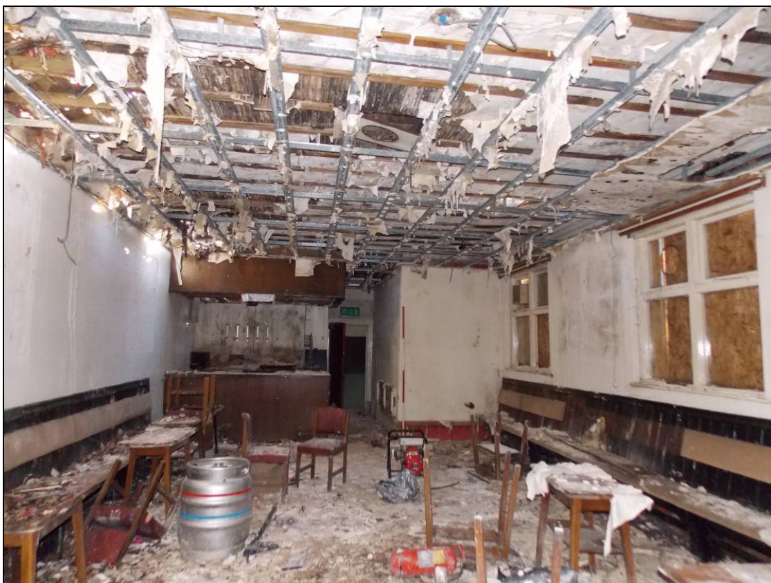
Plate 22: General view of the first floor of the cross-wing, looking east (scale 2m)
