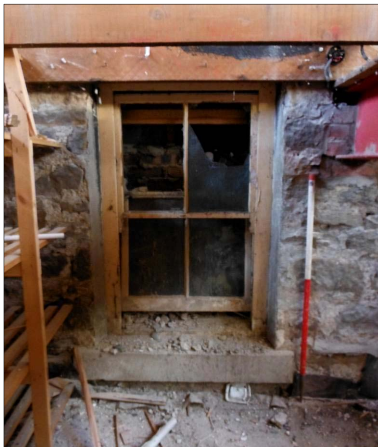
Figure 21: Inserted blocked sash window on the northwest elevation of Building C, preserved within the basement of Building F (scale=1m).
