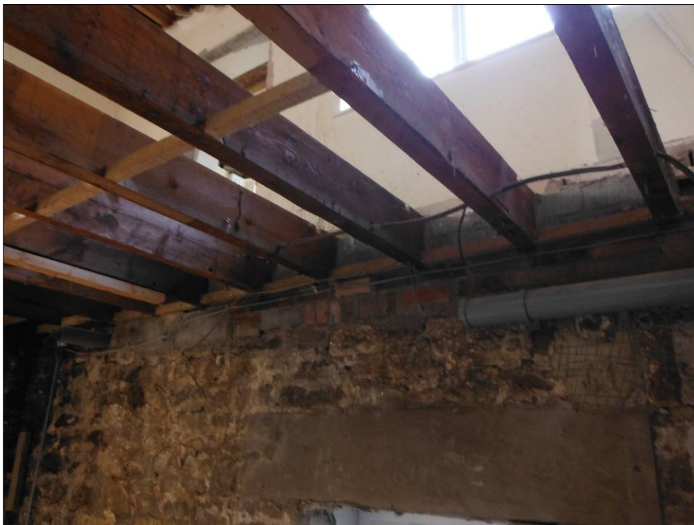
Figure 39: Insertion of the floor and addition of the first floor along the southwest wall of Room C4.
