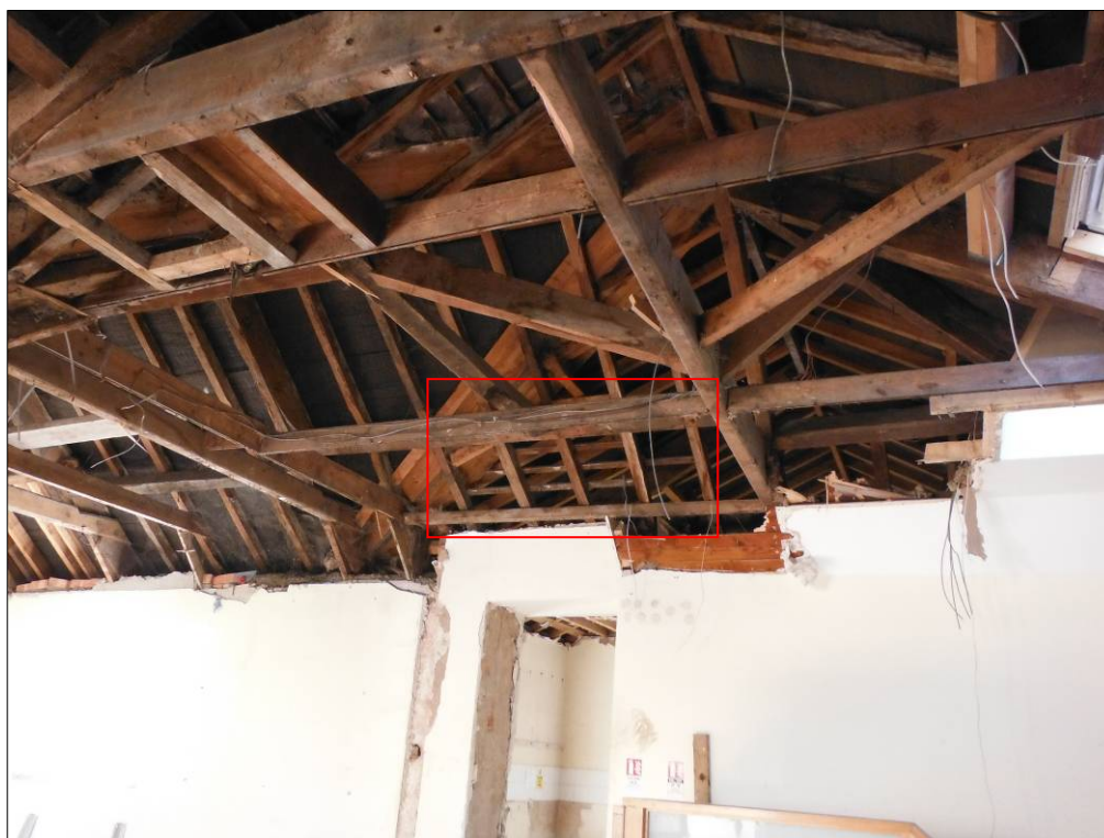
Figure 49: Detail of the roof structure at the first floor over the southwest end of Room C2, showing evidence of the original battens (highlighted in red) to fix the original roof covering, prior to the addition of Room C4 to the west.
