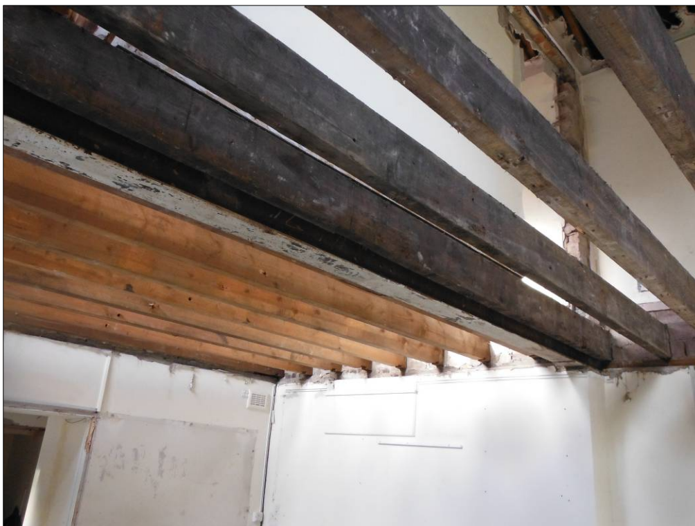
Figure 36: Change in floor structure marking a difference in phase within Room C3; note the inserted RSJ in the centre with the aged reused floor timbers of the eastern portion of the room to the right.
