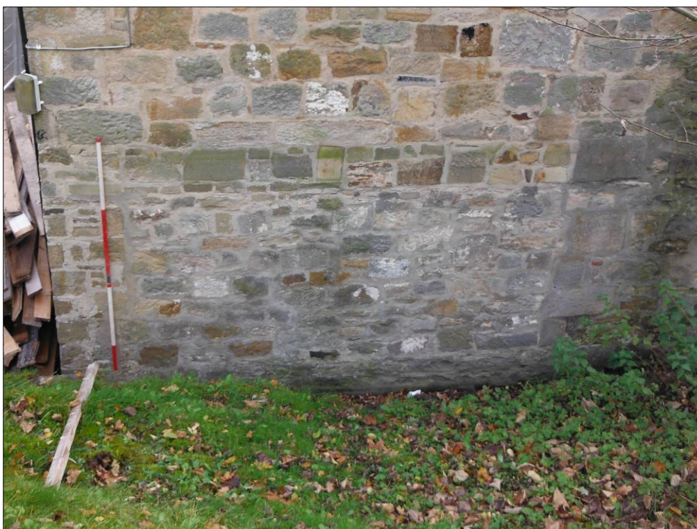
Figure 18: Detail of blocked opening at the eastern end of the northwest elevation of Building C (scale=2m).
