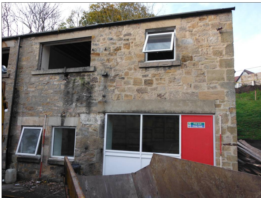
Figure 16: Easternmost section of the southeast elevation of Building C (scale=2 x 2m).
