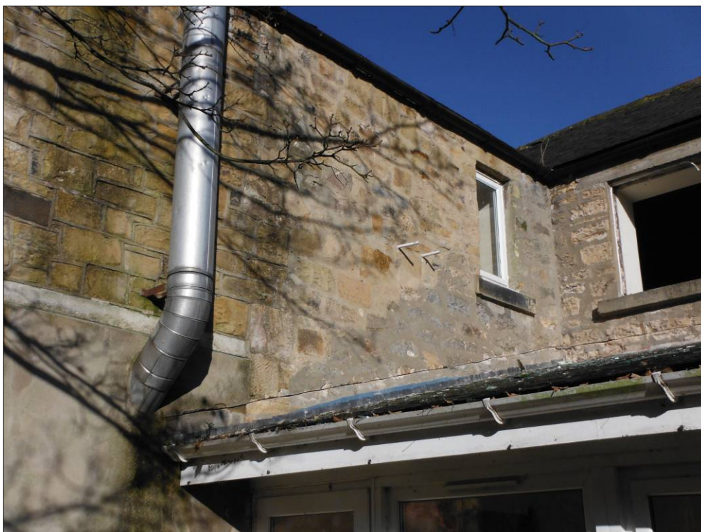
Figure 12: Detail of the ghost of a previous roof line on the southeast elevation of the western part of Building C.
