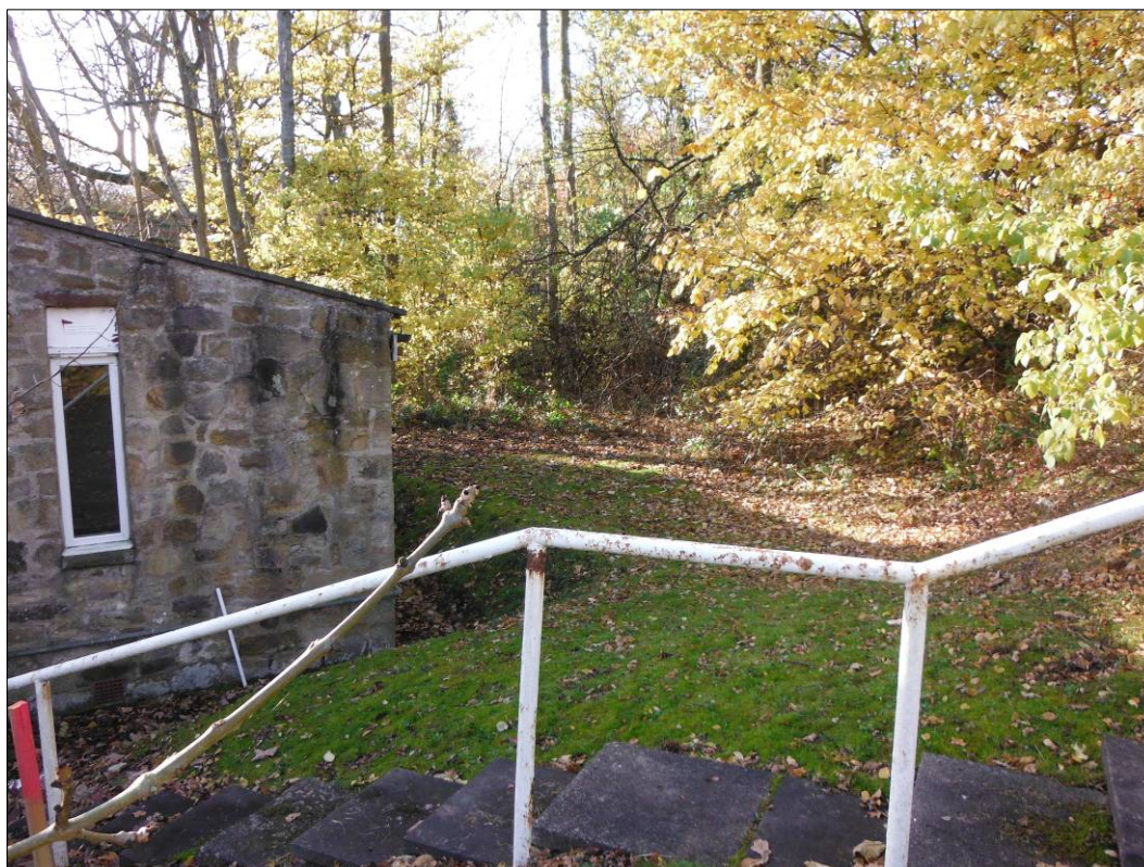
Figure 61: Area of the original mill pond, filled in and cut away to allow the modern extension of the building at this side.
