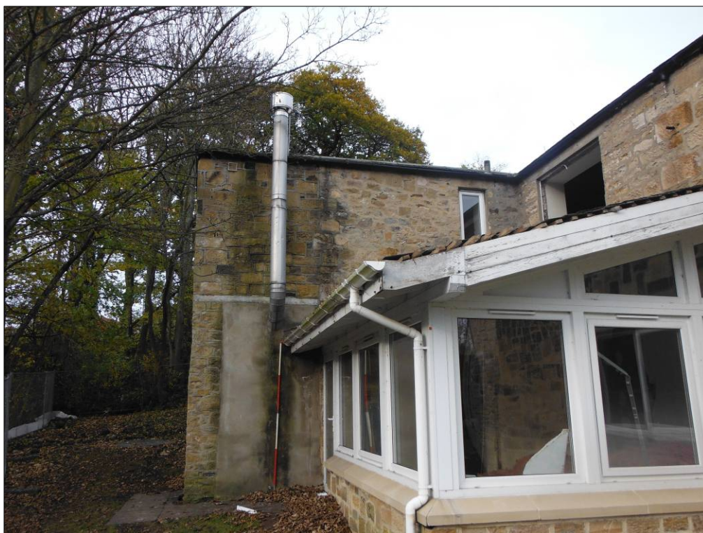
Figure 11: Southeast elevation of the western section of Building C (also showing Building E to the left of the photograph and Building D in the foreground) (scale=2m).
