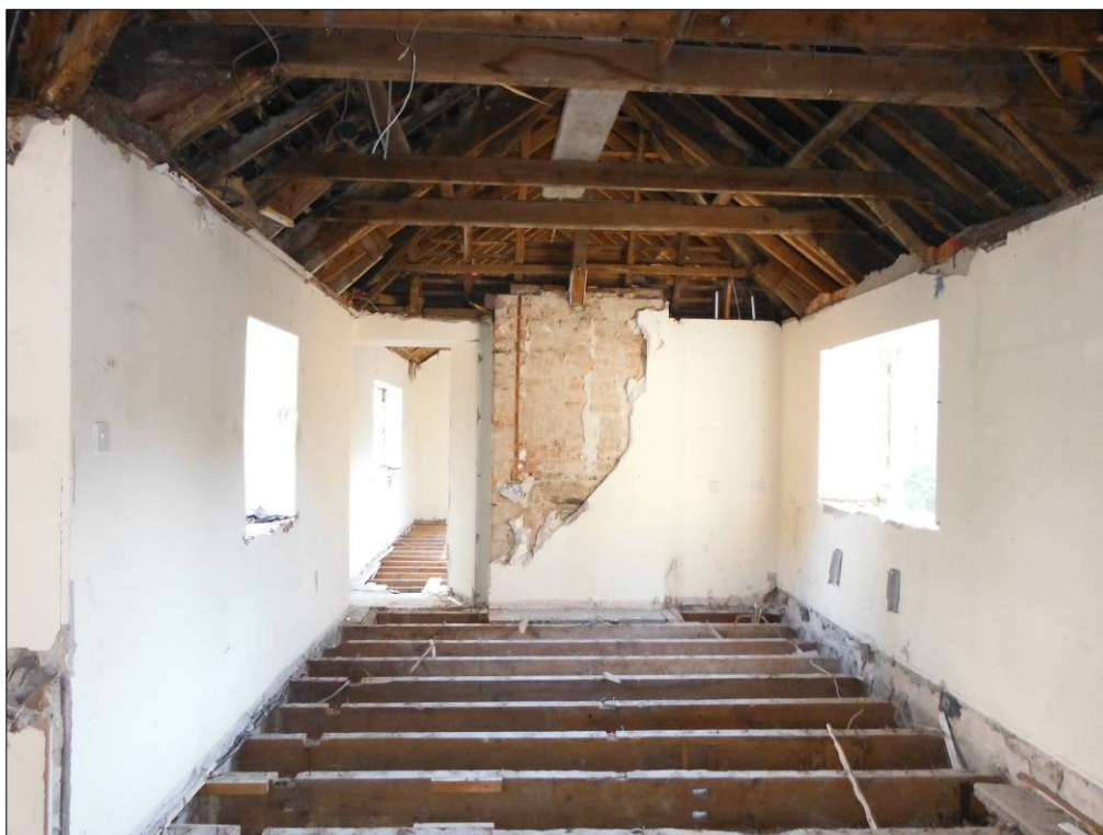
Figure 44: First floor over Room C1, showing inserted fireplace in a brick-built chimney breast in the southeast wall.
