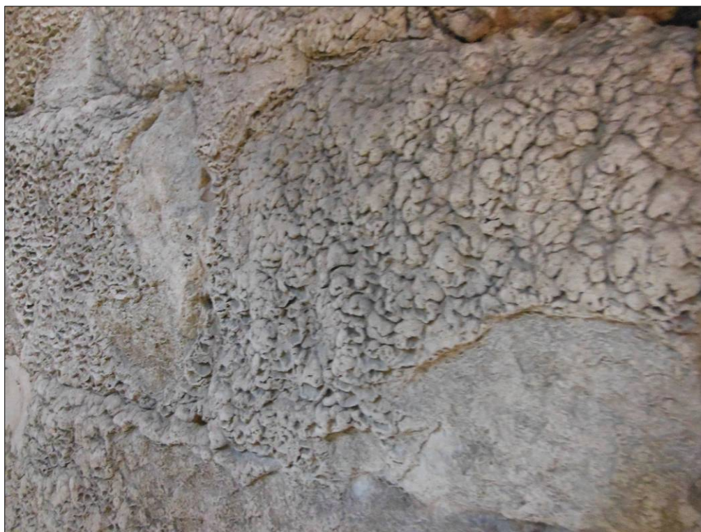
Figure 42: Calcification of the stone on the northeast wall possibly providing evidence of increased water action in this location.
