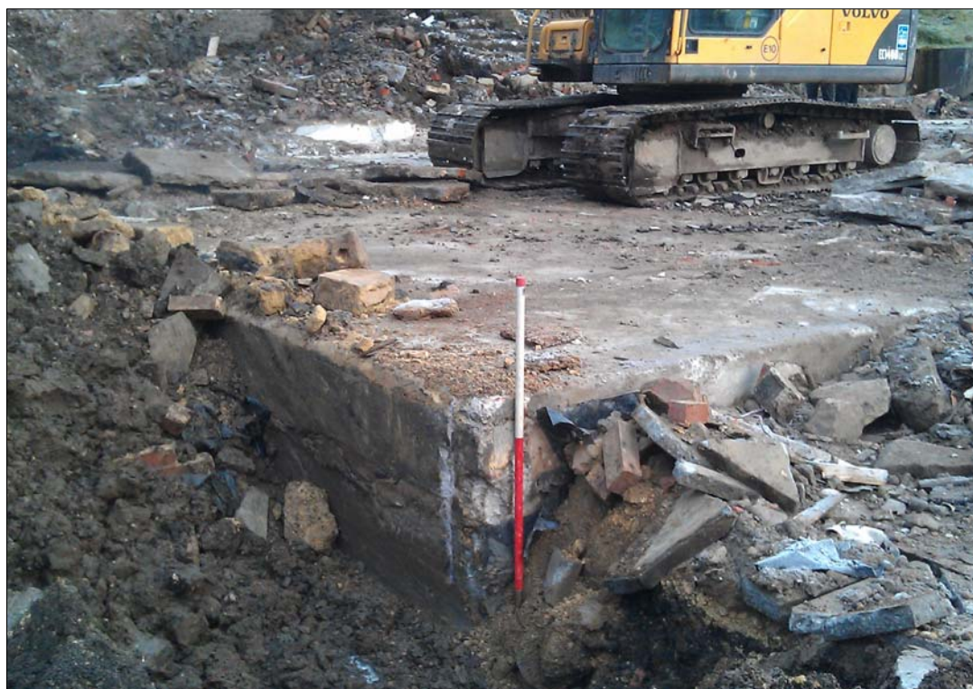
Figure 85: The concrete pad (003) forming the floor of Building C, Room C4 prior to removal
