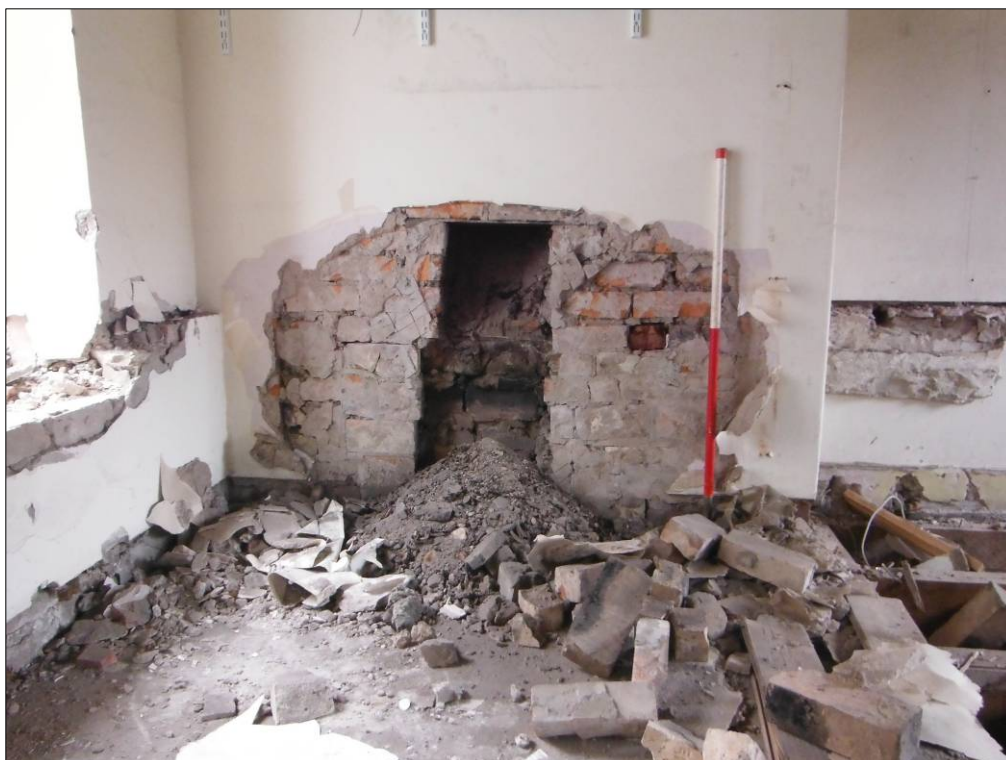
Figure 32: Northern end of the northwest wall at first floor level above Room C2, showing the flue provided in the brick skin applied to the interior of the sandstone wall (scale=1m).
