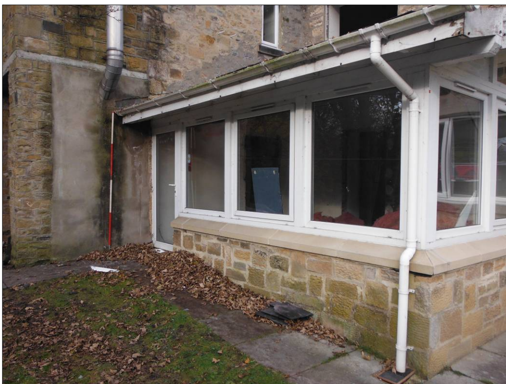
Figure 50: Southwest elevation of Building D, showing Buildings C and E in the background (scale=2m).
