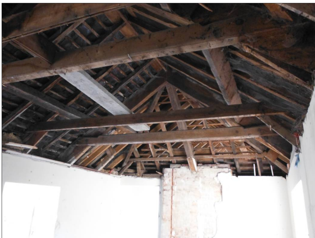
Figure 45: Detail of the roof structure at the first floor over Room C1, showing the original hipped end of the building prior to the addition of Building B to the south.
