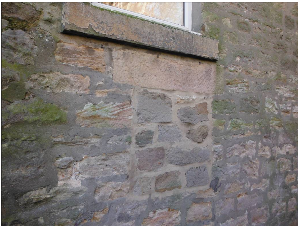
Figure 19: Detail of blocked opening in the ground floor of the middle portion of the northwest elevation of Building C.
