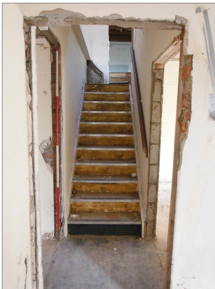
Figure 29: Modern staircase along the southwest wall of Room C2, also showing the brick-built partition of Rooms C1 and C2 in the foreground with the breeze-block partition of the staircase behind (scale=2m).
