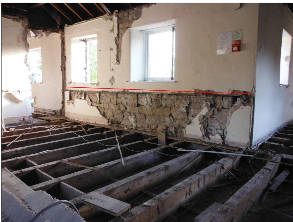
Figure 47: Southeast wall of the first floor over Room C2 showing the original floor level of this part of the building.
