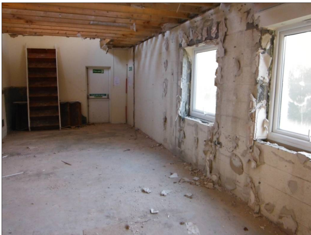
Figure 5: Interior of Building A, showing the southeast and southwest walls with remains of the staircase along the southeast end of the building (scale= 2m).
