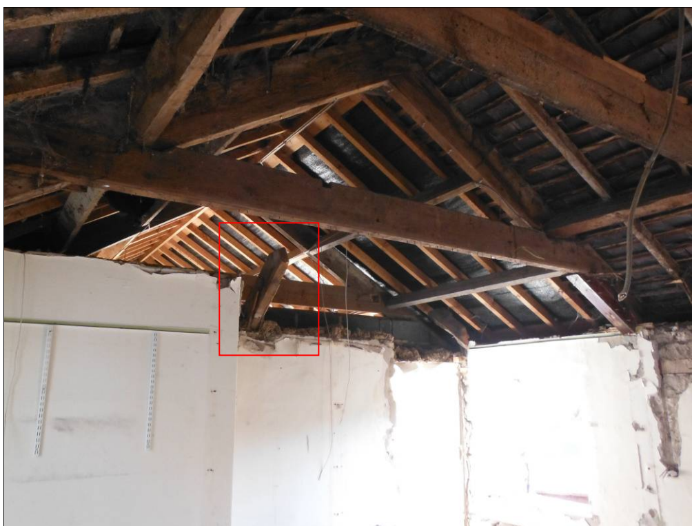
Figure 48: Detail of the roof structure at the first floor over Room C2, showing evidence of the original hipped end of the building (outlined in red) prior to the addition of extensions to the east.
