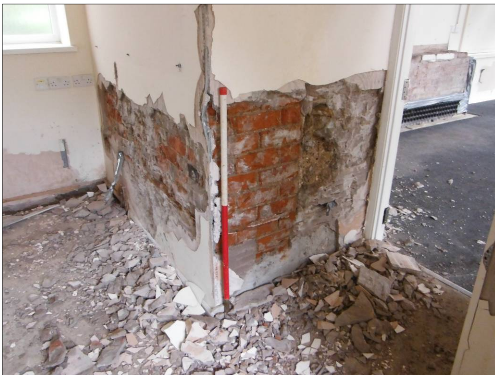
Figure 31: Northern end of the northwest wall of Room C2, showing the brick skin applied to the interior of the sandstone wall (scale=1m).
