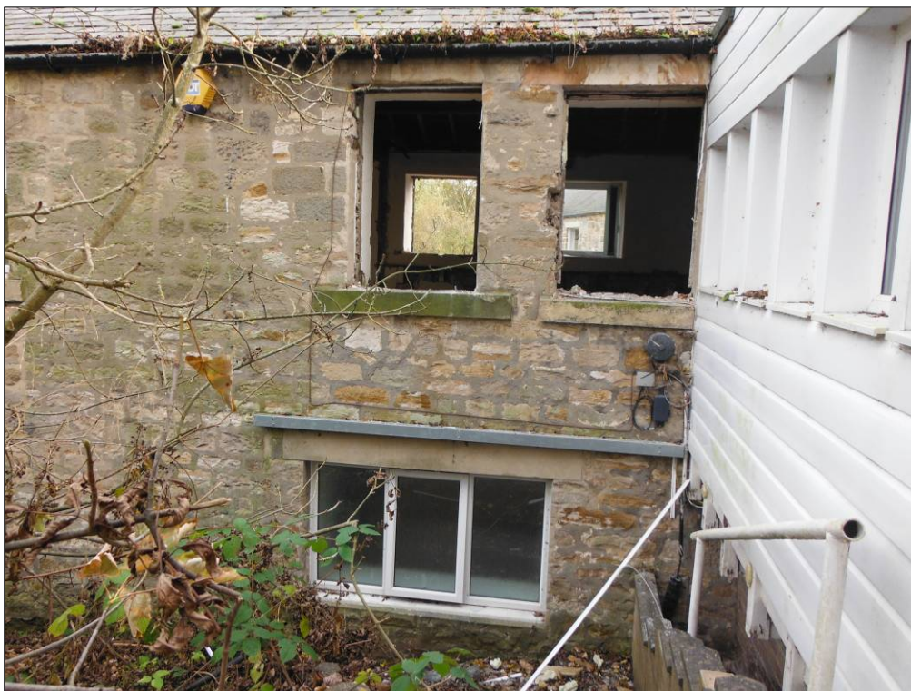
Figure 20: Western section of the northwest elevation of Building C before it is obscured by Building F.
