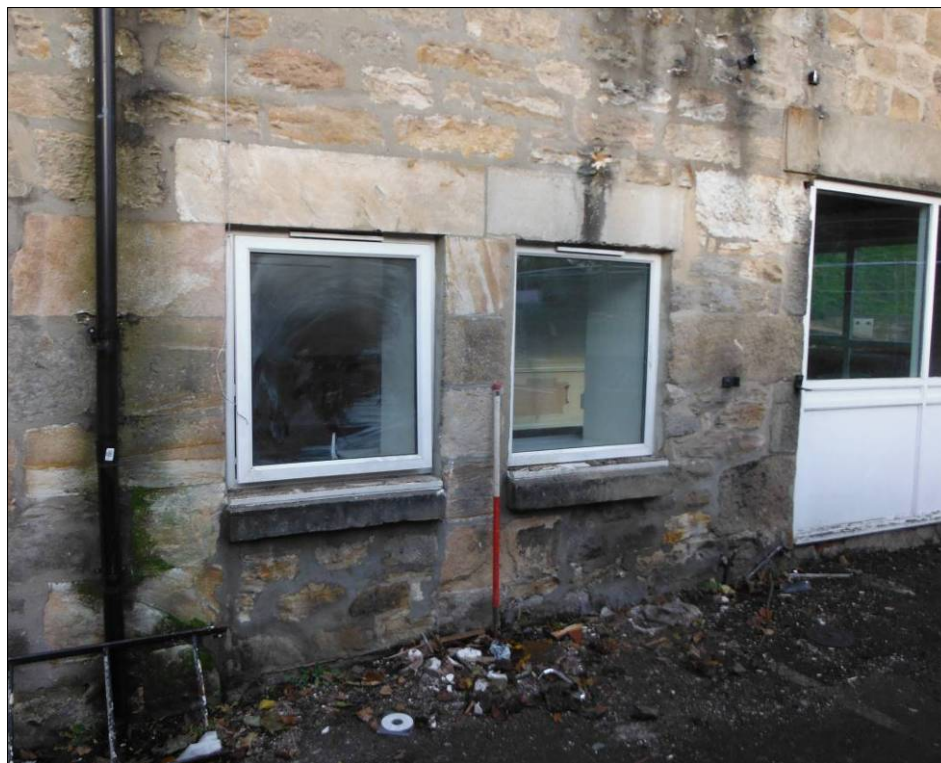
Figure 15: Detail of blocked original doorway on the middle section of the southeast elevation of Building C (scale=1m).
