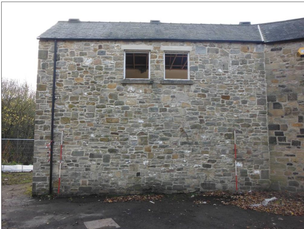
Figure 2: Northeast elevation of Building A showing vertical joint between Building A and B, on the right of the photograph (scale=2 x 2m).
