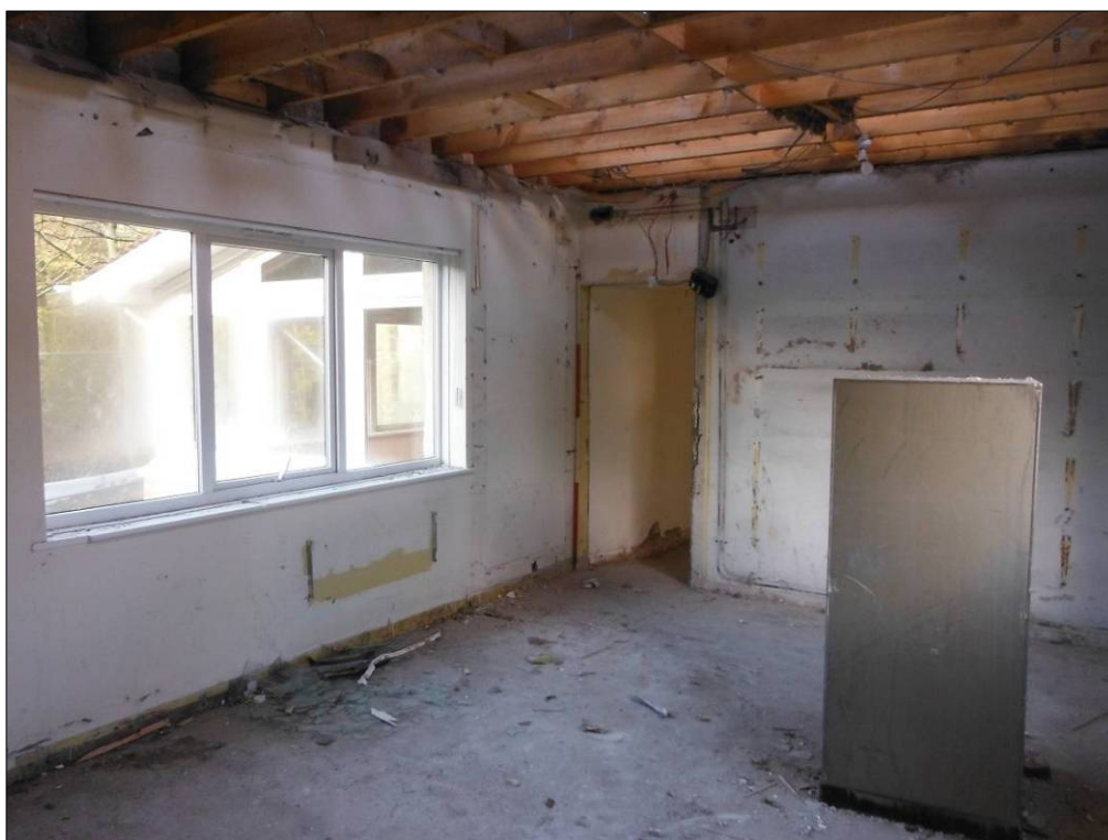
Figure 8: Interior of Building B, showing the southwest and northwest walls (scale= 2m).
