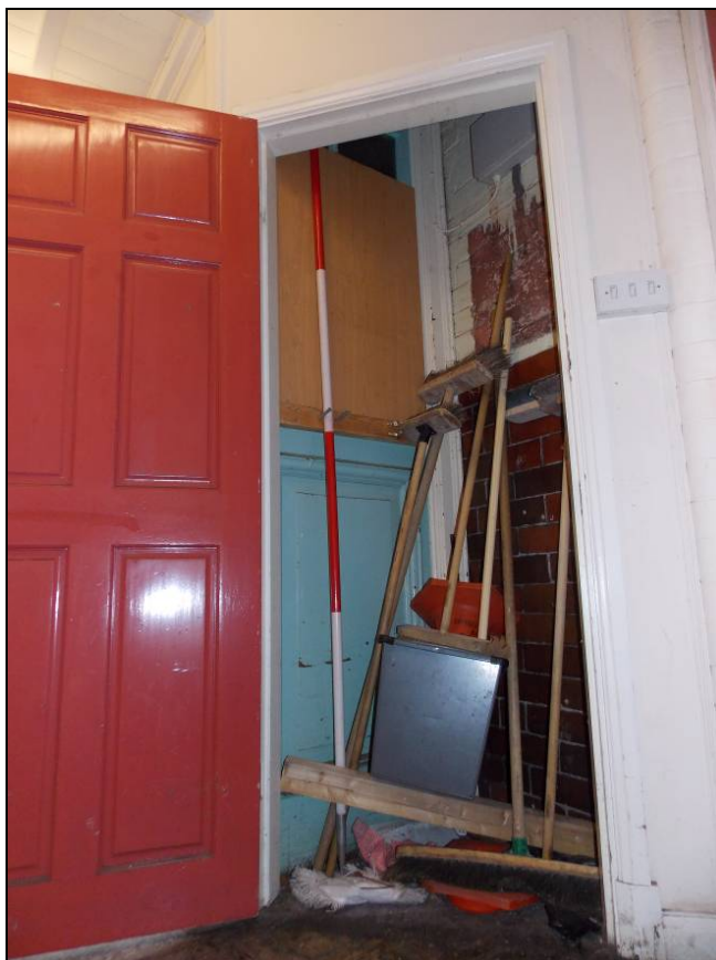
Plate 22: Storage cupboard concealing a former stud panel with boarded-up glazing lights (scale 2m).
