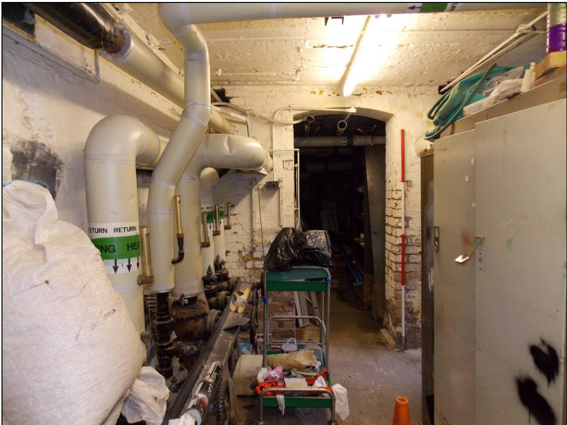
Plate 47: General view of the boiler room, looking west (scale 2m).
