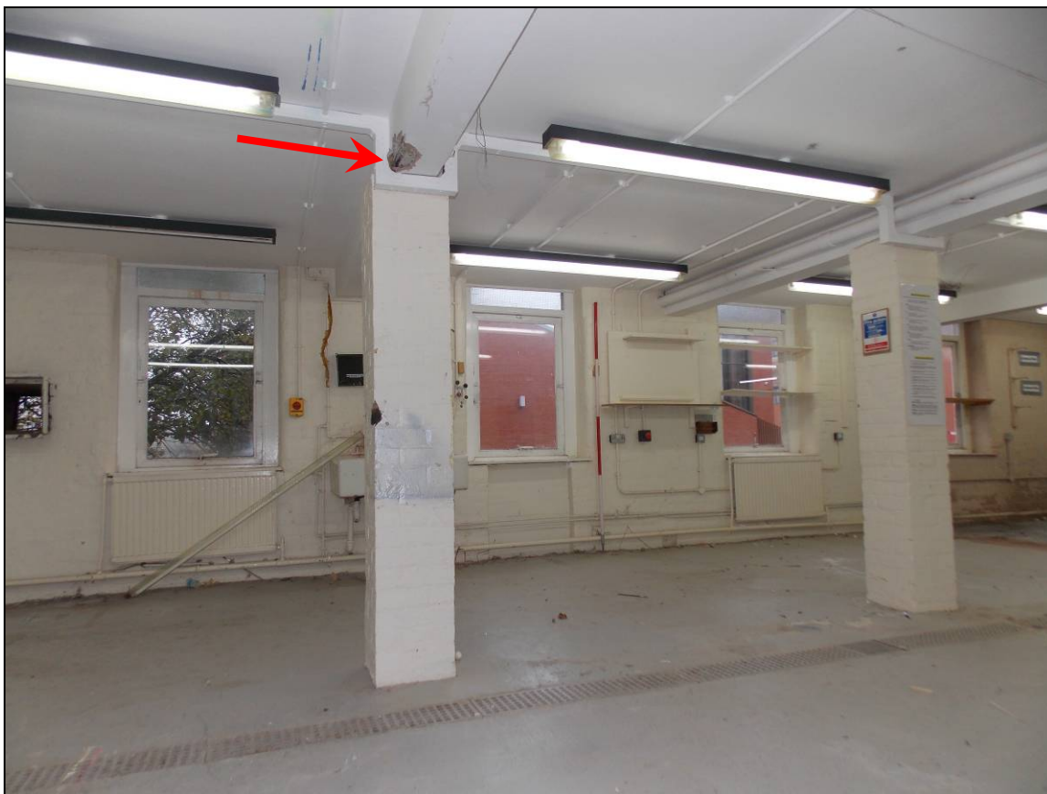
Plate 71: Timber ceiling beam concealed by later plasterboard (arrow), looking east (scale 2m).
