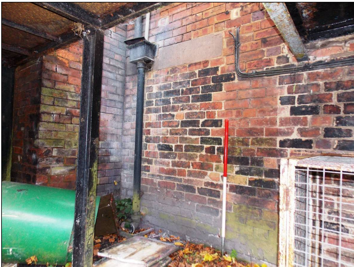
Plate 55: Blocked-up opening adjacent to the upright shaft block, looking north-east (scale 1m).
