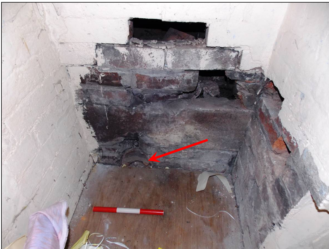
Plate 118: View of the block with remnants of a ceramic drain pipe (arrow), looking north (scale 300mm).
