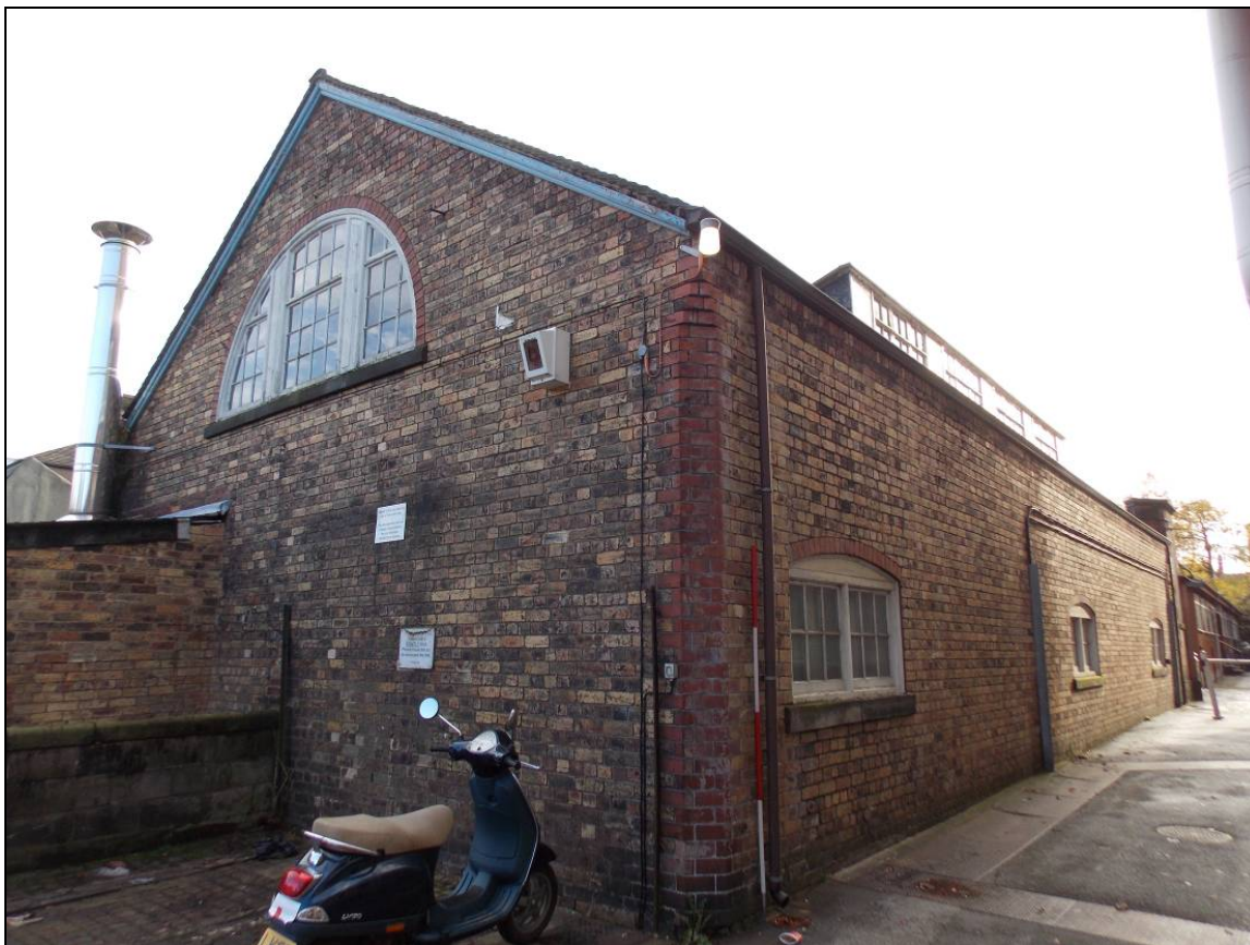
Plate 11: Northern end of the west elevation and gabled north wall, looking south-east (scale 2m).
