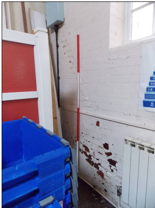
Plate 41: Scars of a former staircase within the southernmost end of the west wall, looking south (scale 2m).
