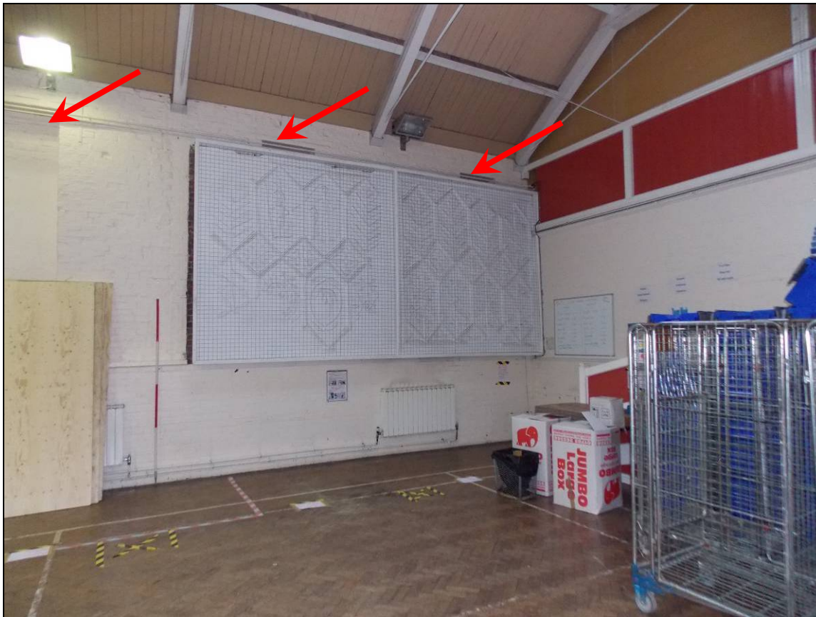
Plate 33: Blocked-up openings (arrows), two of which are behind the plaster ceiling (scale 2m).
