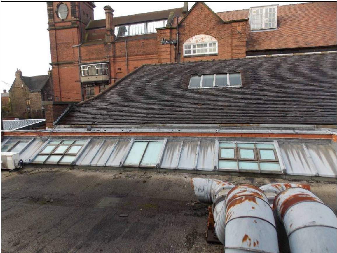
Plate 15: Southern side of the east elevation obscured by later abutments, looking west.
