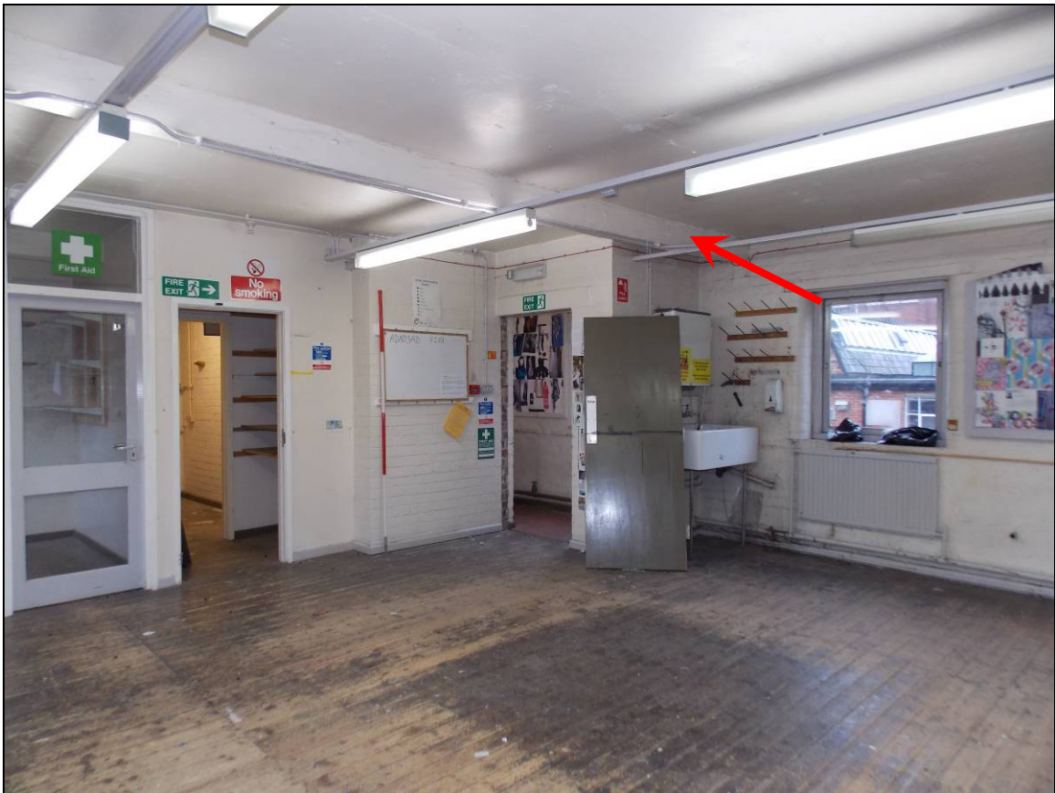
Plate 111: Exposed tie-beam (truss V) with carpenter's marks (arrow), looking south-west (scale 2m).
