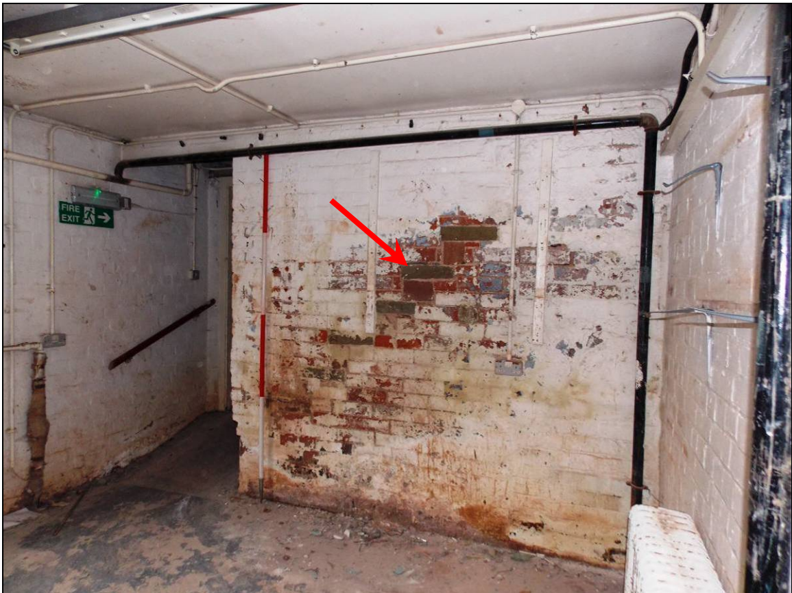
Plate 80: Partition wall of the original stairwell with discernable treads and raisers (arrow) (scale 2m).
