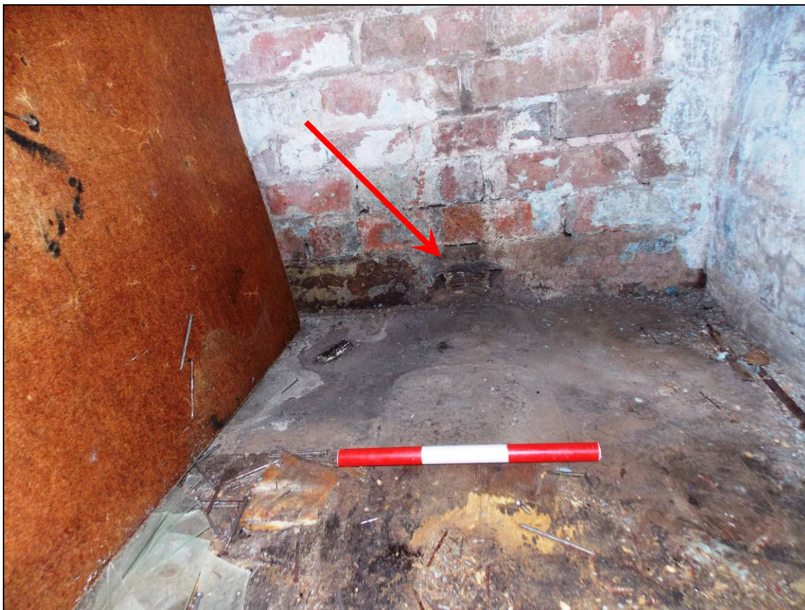
Plate 98: Scars of a former toilet and remnants of a ceramic drain pipe (arrow), looking north (scale 300mm).
