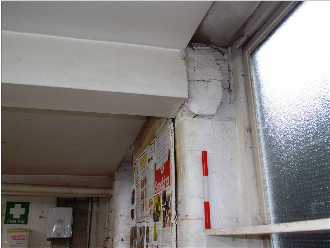
Plate 73: Detail of the west end of the fifth beam from the north, looking south (scale 300mm).
