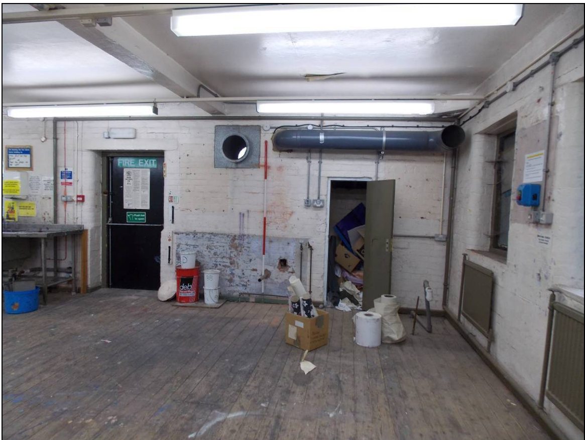
Plate 117: Doorway to the shaft block and inserted fire exit door, looking west (scale 2m).
