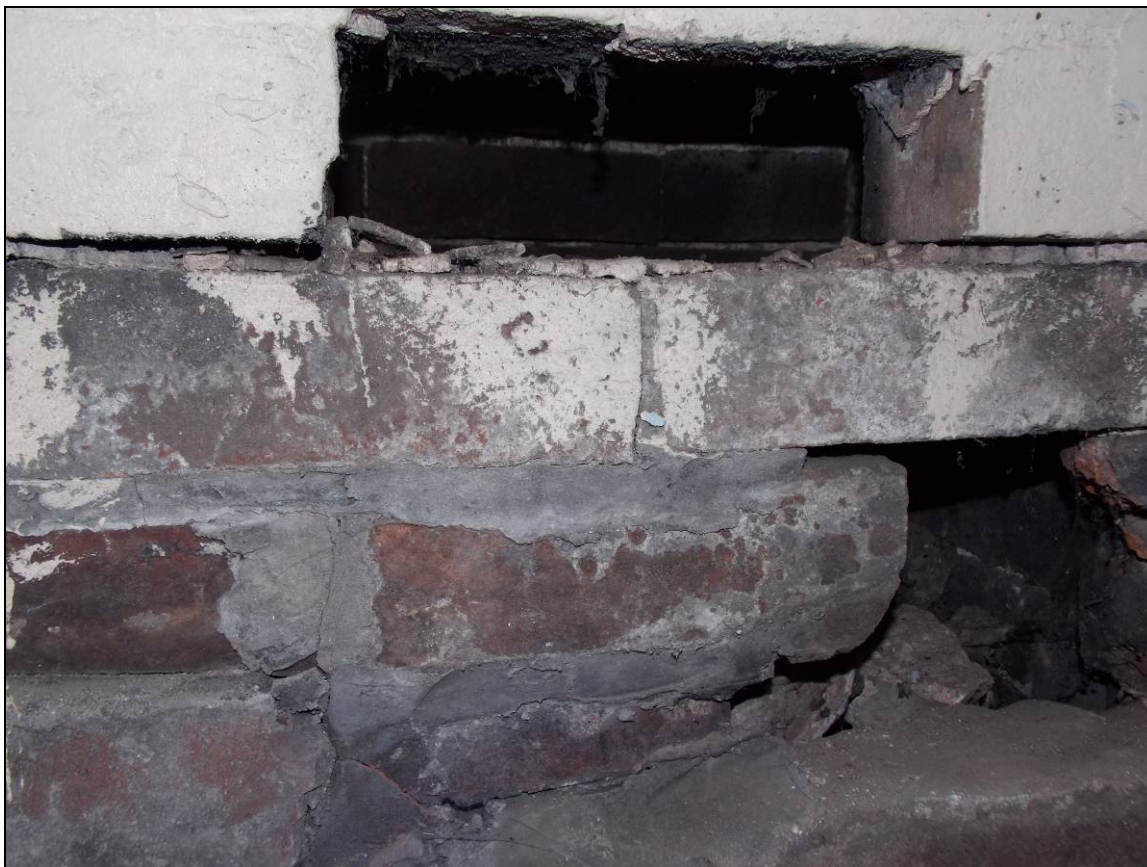
Plate 119: Detail of later brick repair and cavity behind the inserted northern wall.
