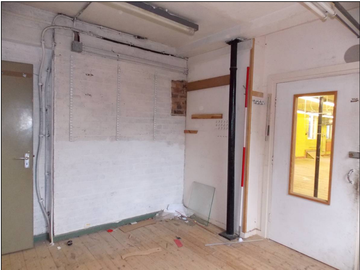
Plate 100: Office room with a cast-iron column behind the stud partition, looking north-west (scale 2m).
