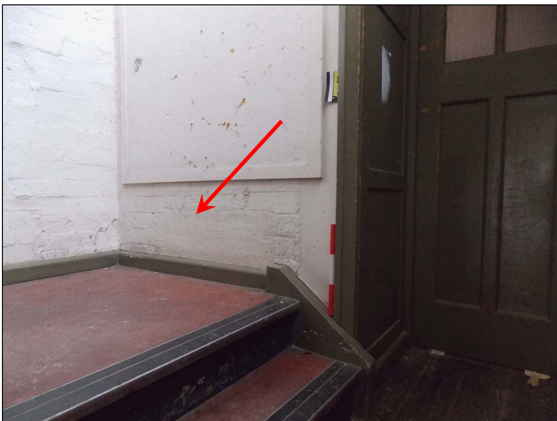
Plate 104: Lintel of former fire place within the south wall (arrow), looking south-east (scale 300mm).
