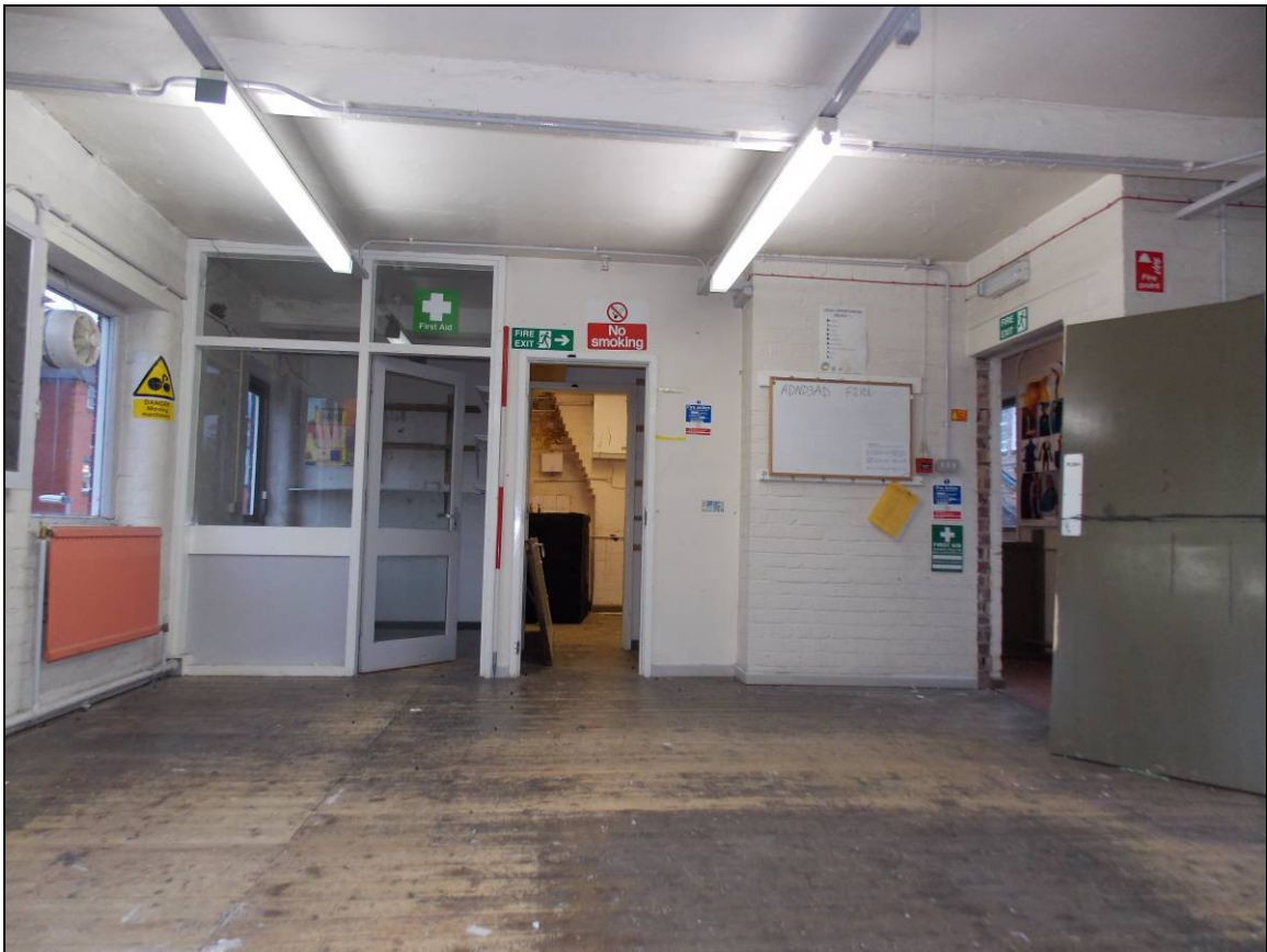
Plate 121: Partition wall with glazed studded section for the south-eastern room, looking south (scale 2m).
