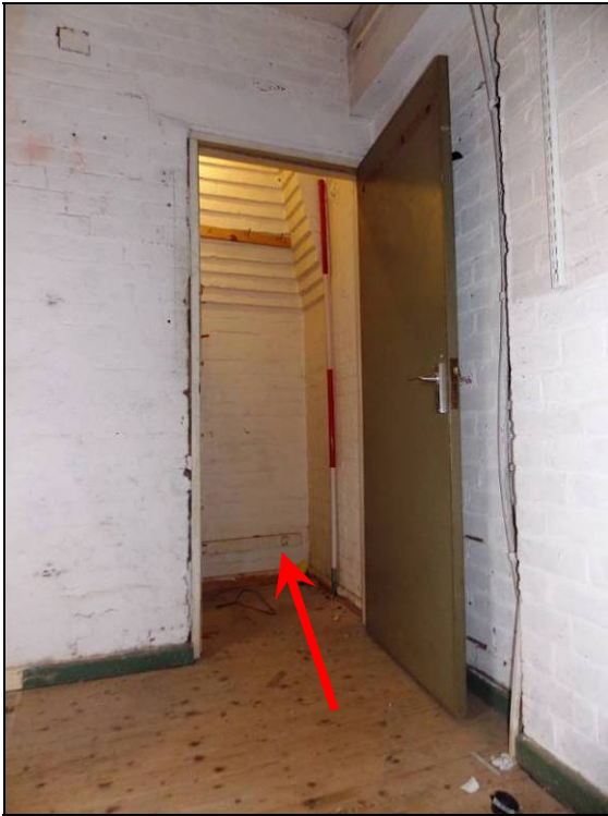
Plate 101: Doorway to original stairwell with chimney breast and tie plate (arrow) attached to it (scale 2m).
