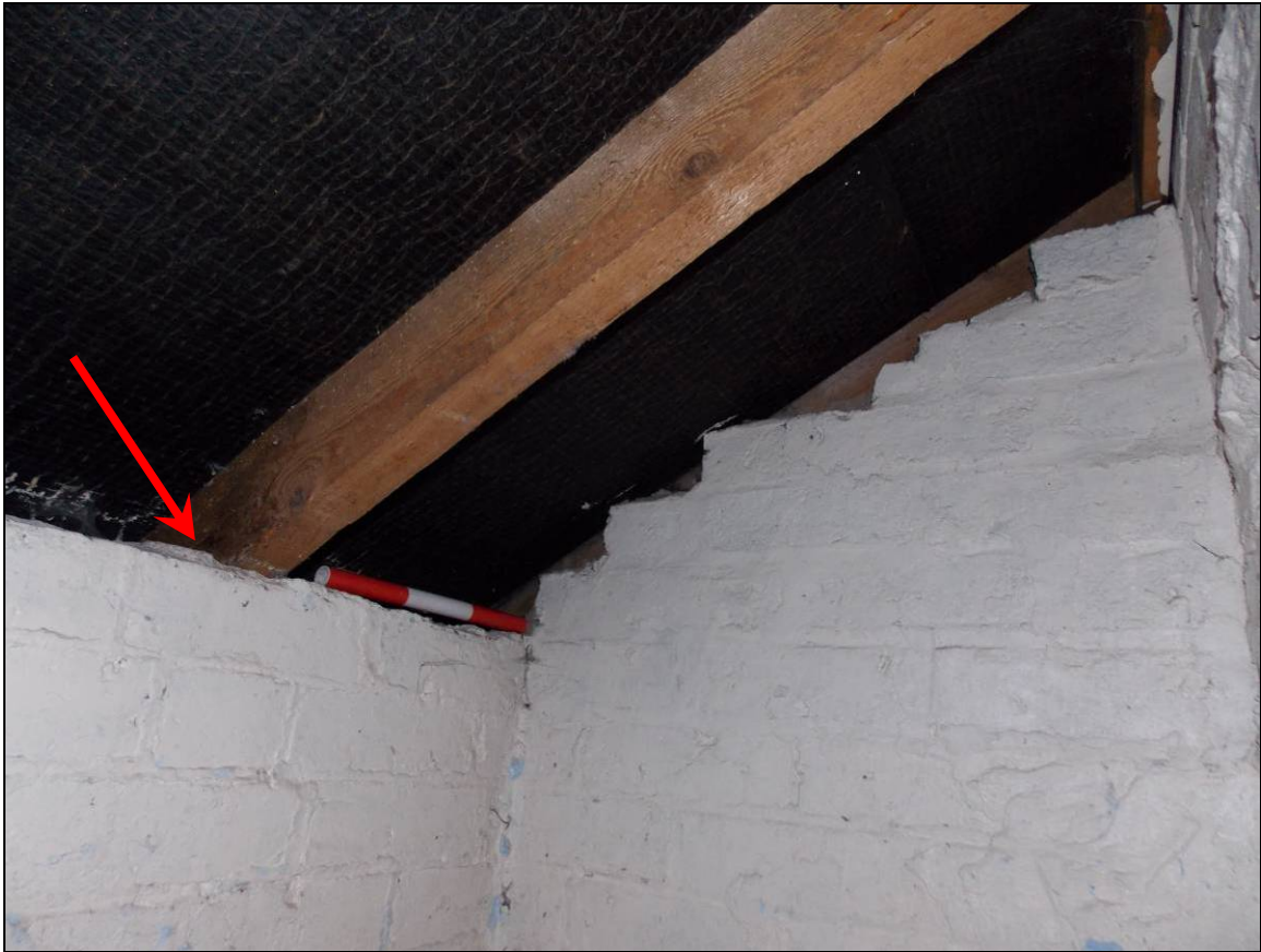
Plate 120: Mortar bedding (arrow) of removed courses over the west wall (scale 300mm).
