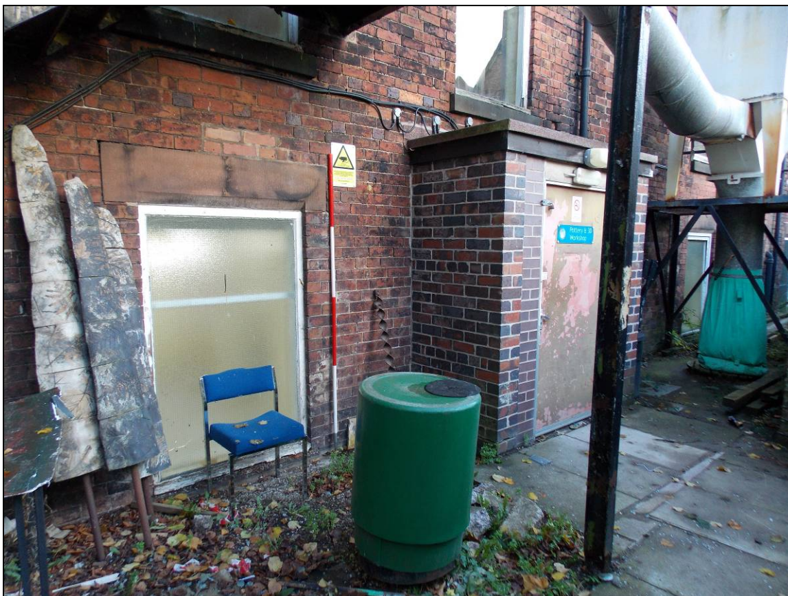
Plate 54: Detail of ground floor's entrance within a later extension, looking east (scale 2m).
