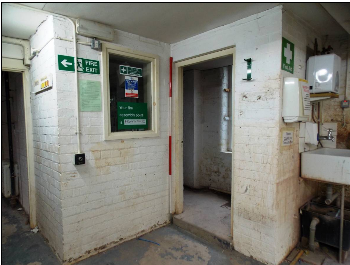
Plate 77: Inserted partition within the south-western corner of the ground floor, looking south-west (scale 2m).
