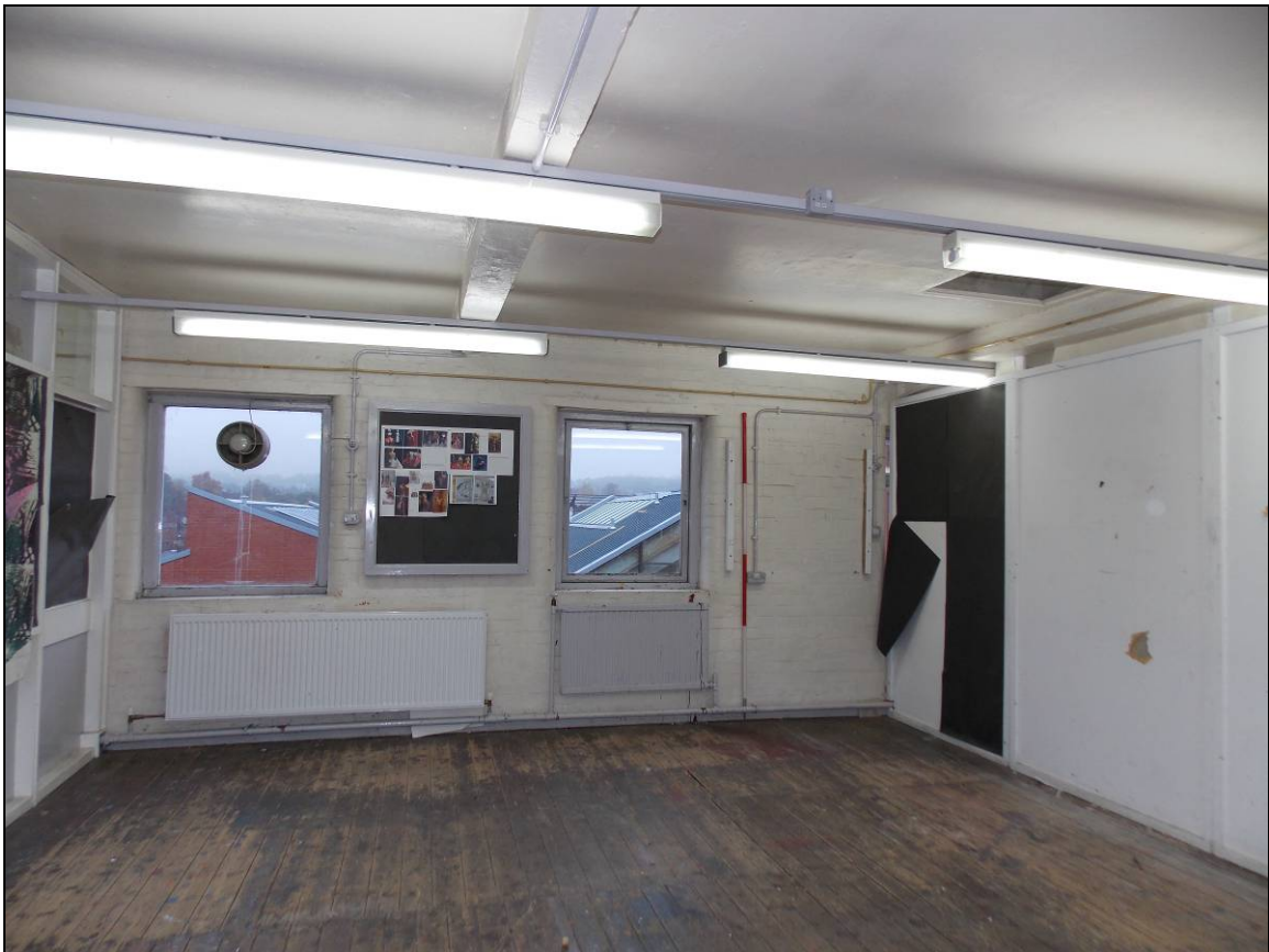
Plate 113: Ceiling hatch adjacent to exposed tie-beam (truss IIII), looking east (scale 2m).
