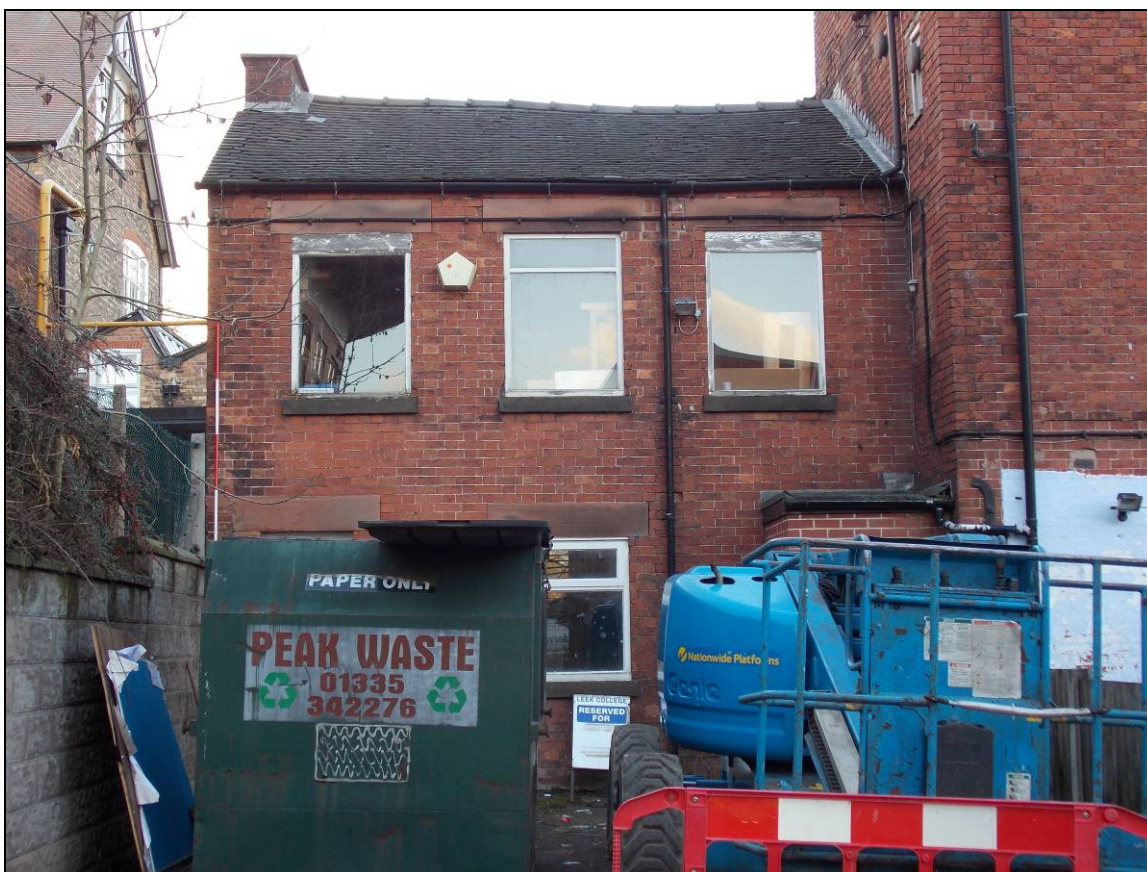
Plate 64: General view of the west elevation of the southern extension (scale 2m).
