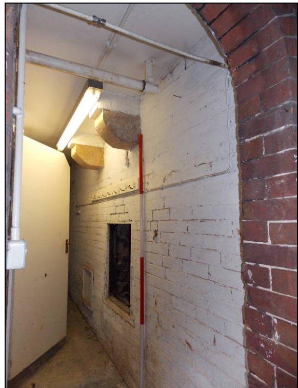
Plate 86: Flue vent, inserted under-stairs cupboard and corbels supporting a brick stack (scale 2m).
