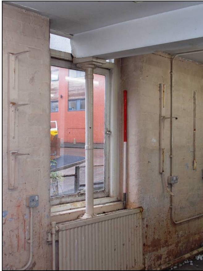
Plate 75: Detail of column within the central window opening of the east wall, looking south-east (scale 1m).
