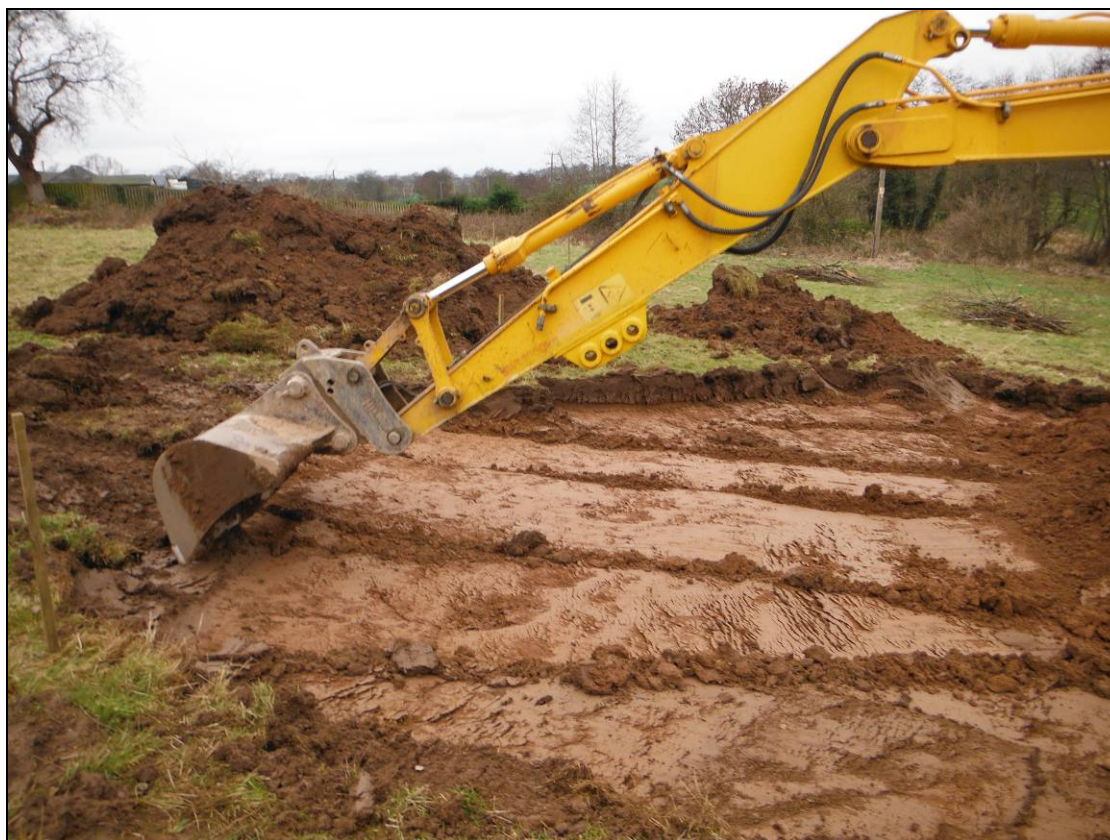
Figure 25. Working shot of the excavation of Pond 2, showing the upper surface of the subsoil. Facing north-west.
