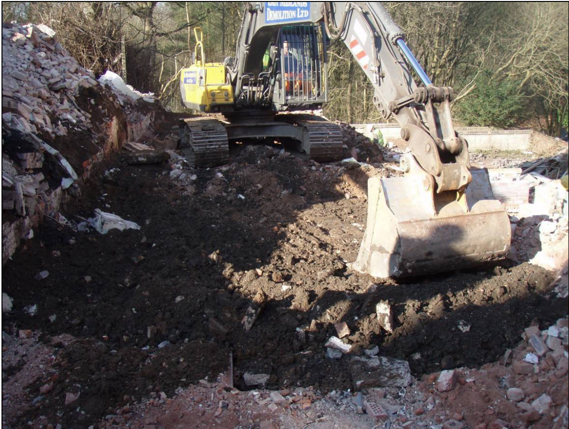
Figure 5: Made ground layer beneath the concrete floor of the Mill, looking north.
