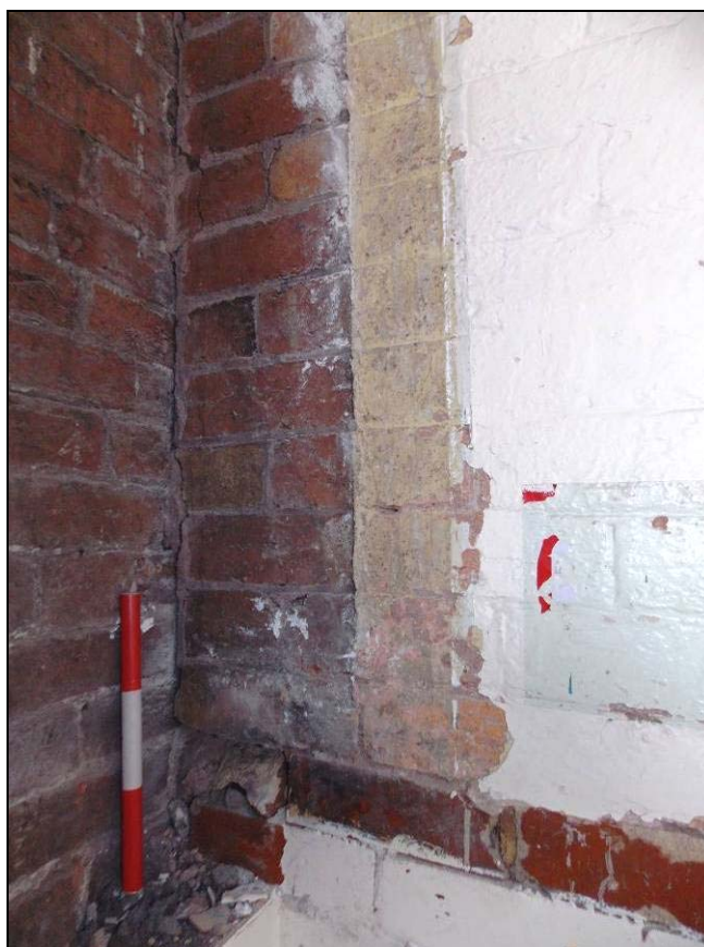
Figure 50: Detail of construction break/joint between the east and south walls (scale 300mm).
