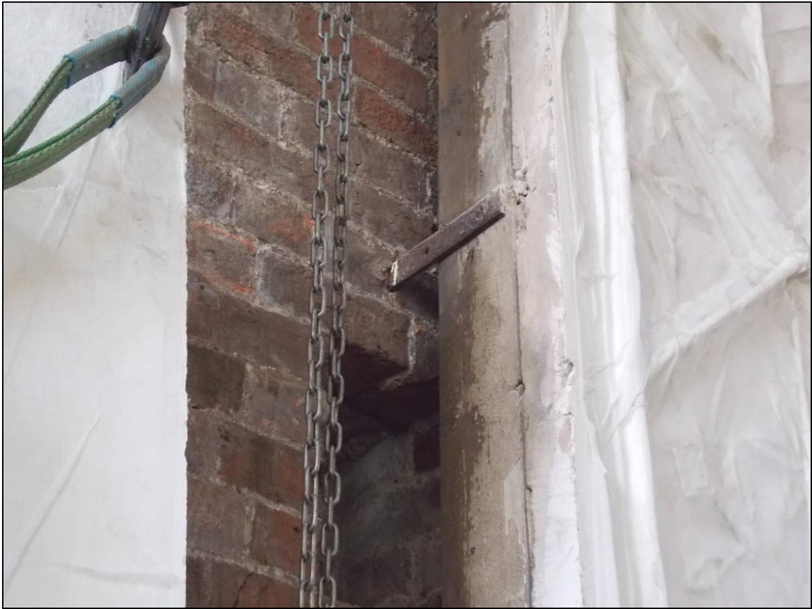
Figure 20: Detail of iron strap supporting the frame of Panel 2.
