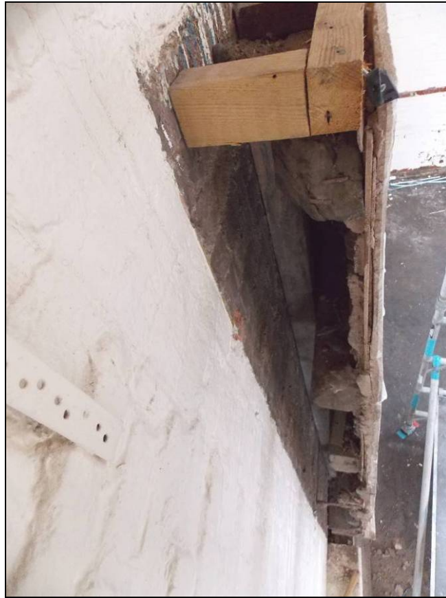
Figure 18: Lateral edge of the plaster ceiling mounted on the east wall, looking south.
