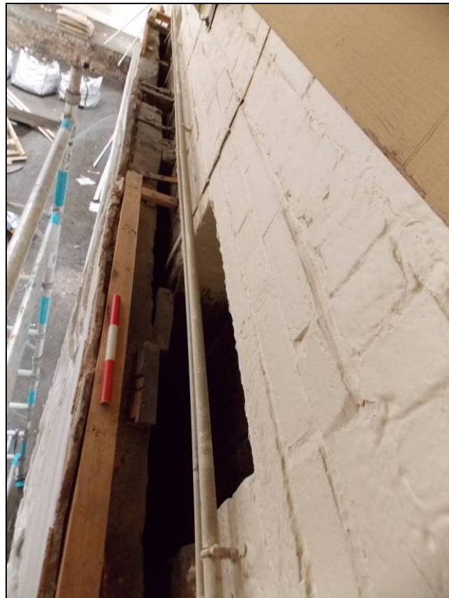
Figure 17: Upper edge of the plaster ceiling mounted on the east wall (scale 300mm).
