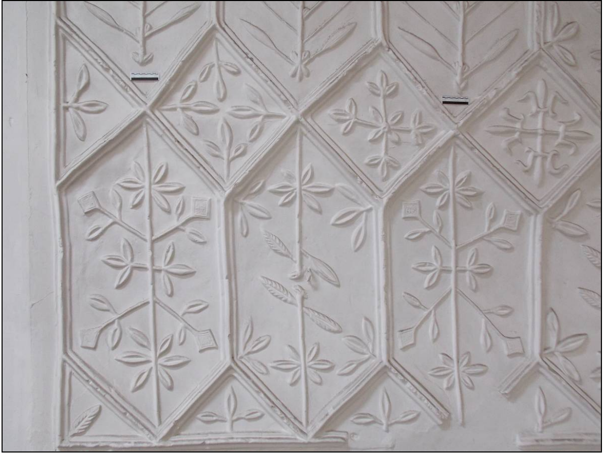
Figure 40: Lower left section of Panel 2 (scale 2 x 100mm).
