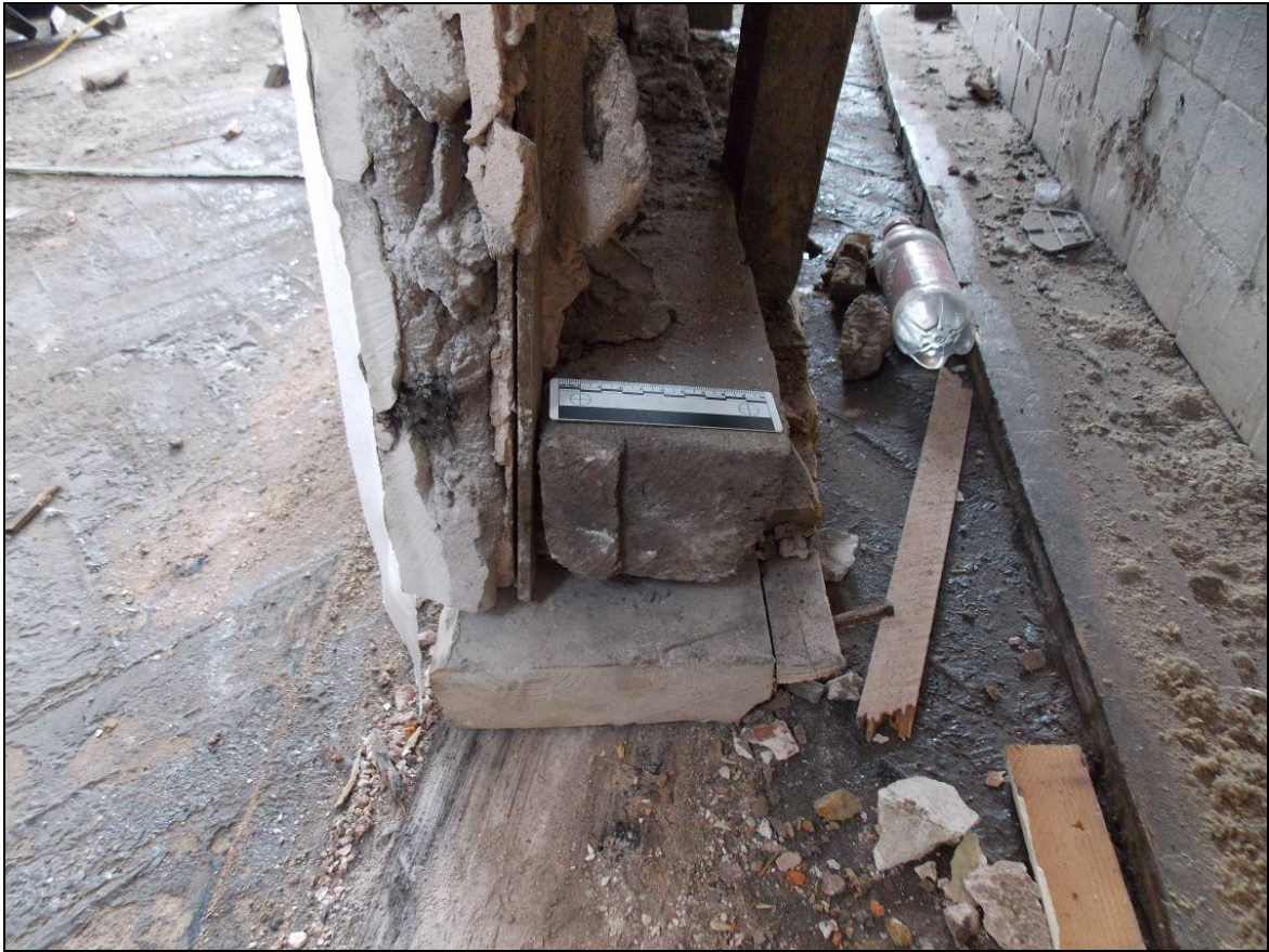
Figure 30: Ceiling joist with sawn-off tenon (scale 100mm).
