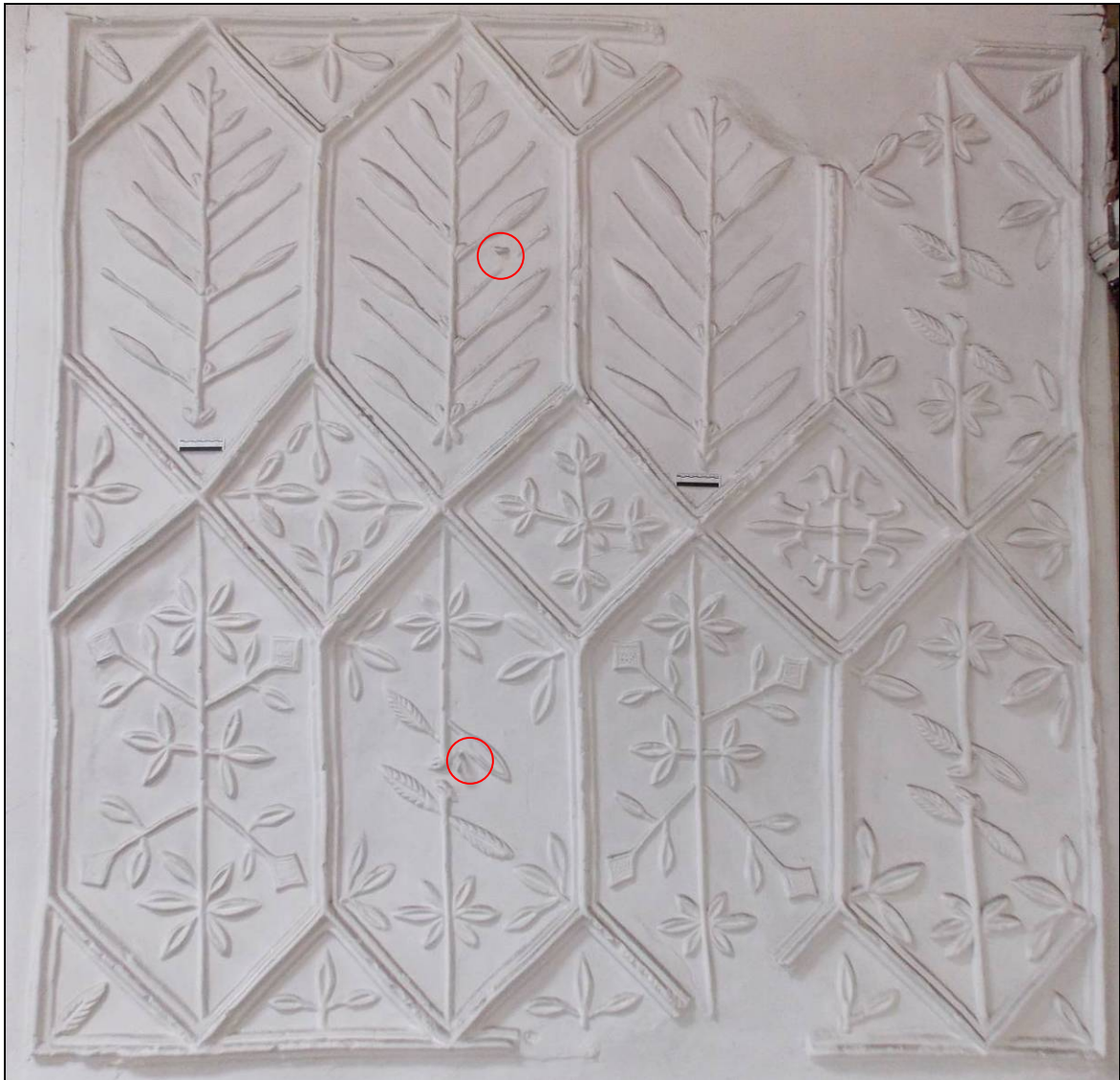
Figure 37: General view of Panel 2 with two hooks denoted by red circles (scale 2 x 100mm).
