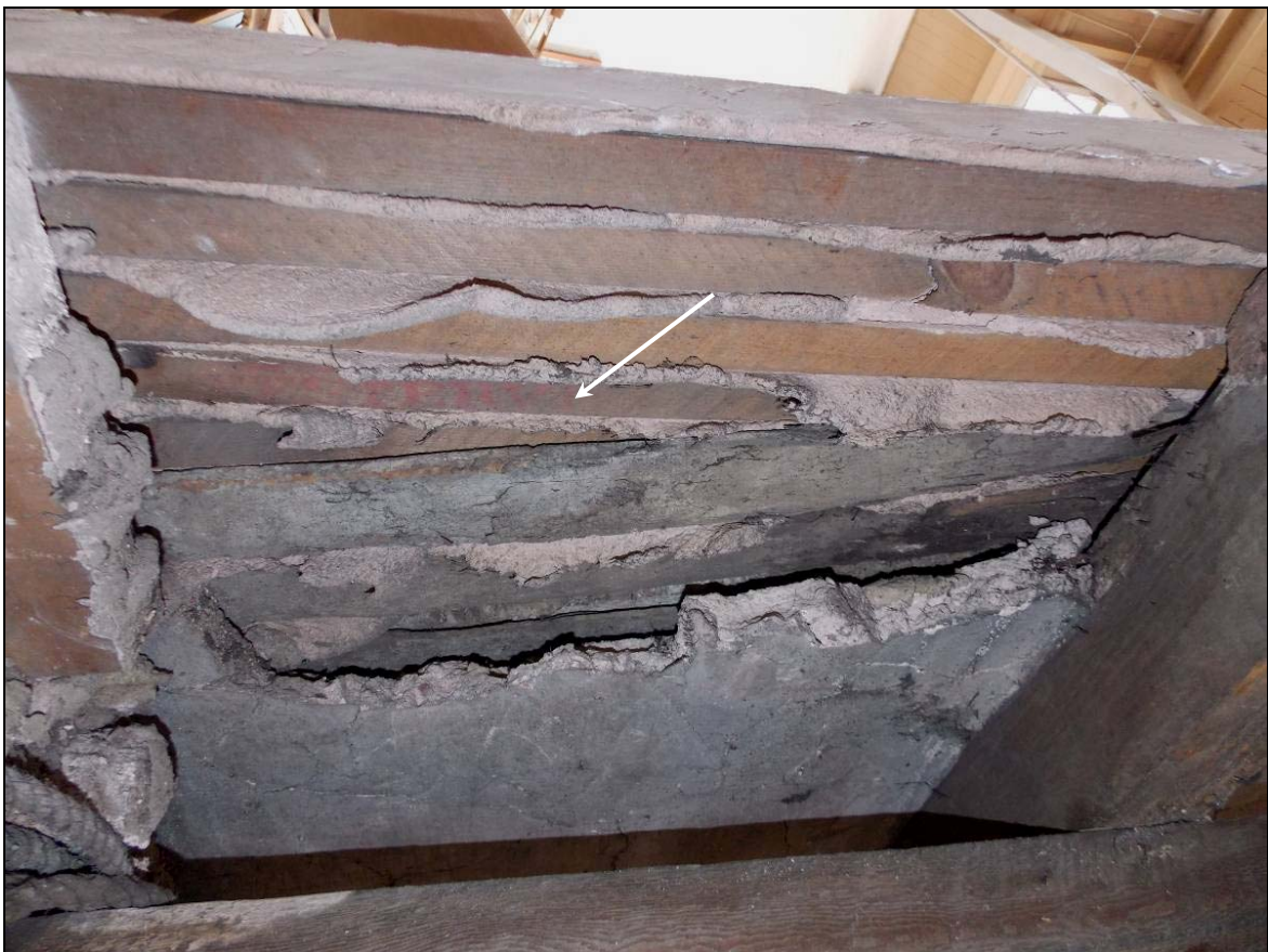
Figure 33: Detail of replaced lath with printed writing (arrow).
