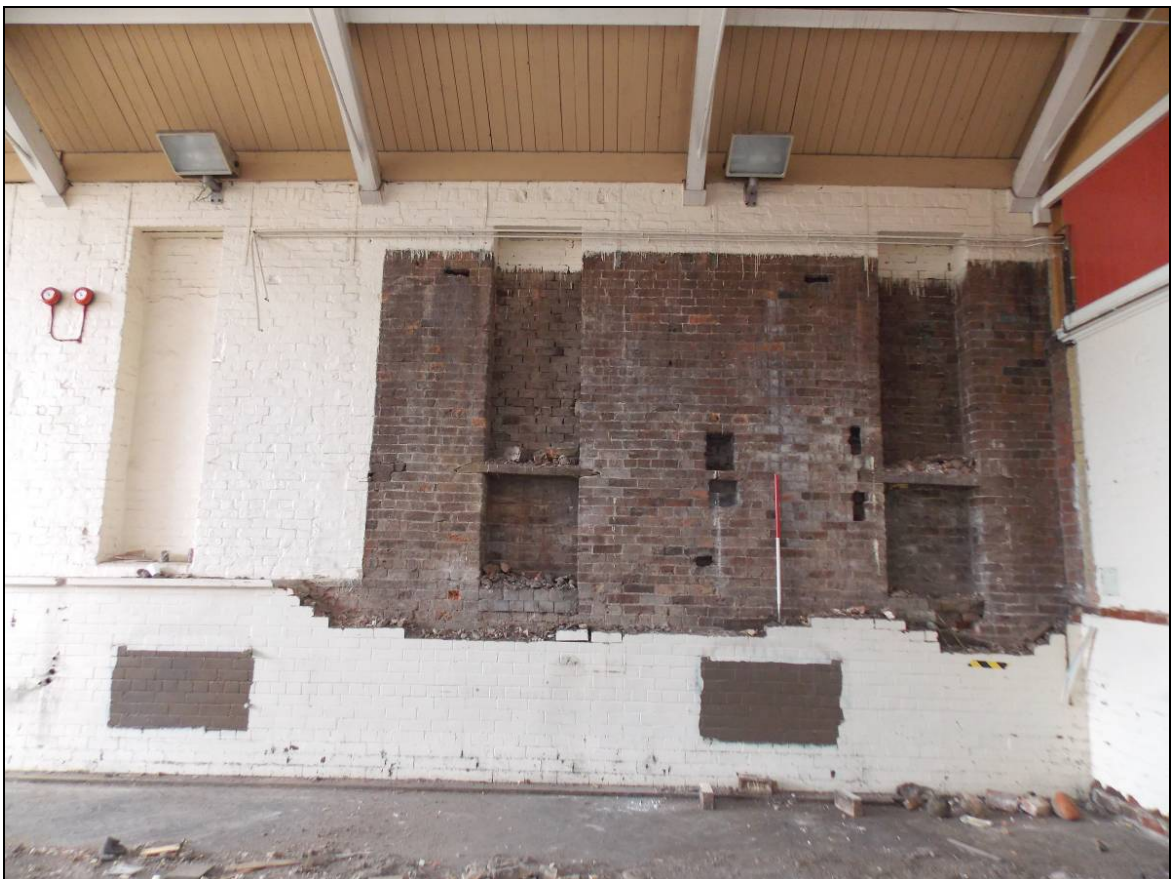
Figure 49: Southern end of the east wall following the dismantlement of the ceiling (scale 1m).
