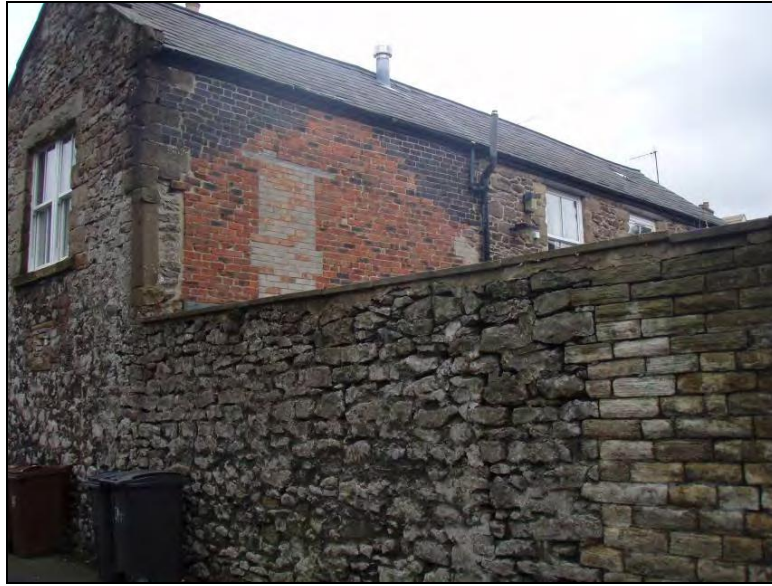
Figure 15. Wall (116), taken from Torr Street, before demolition. The wall clearly runs in a continuous line until it meets with the existing stable building. Facing north-east.
