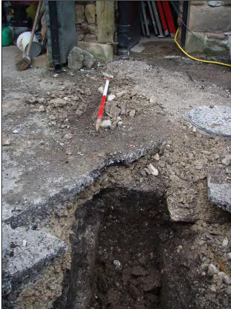
Figure 7. Wall (106) shown in alignment with the existing stable block wall. Facing north. Scale = 1m.
