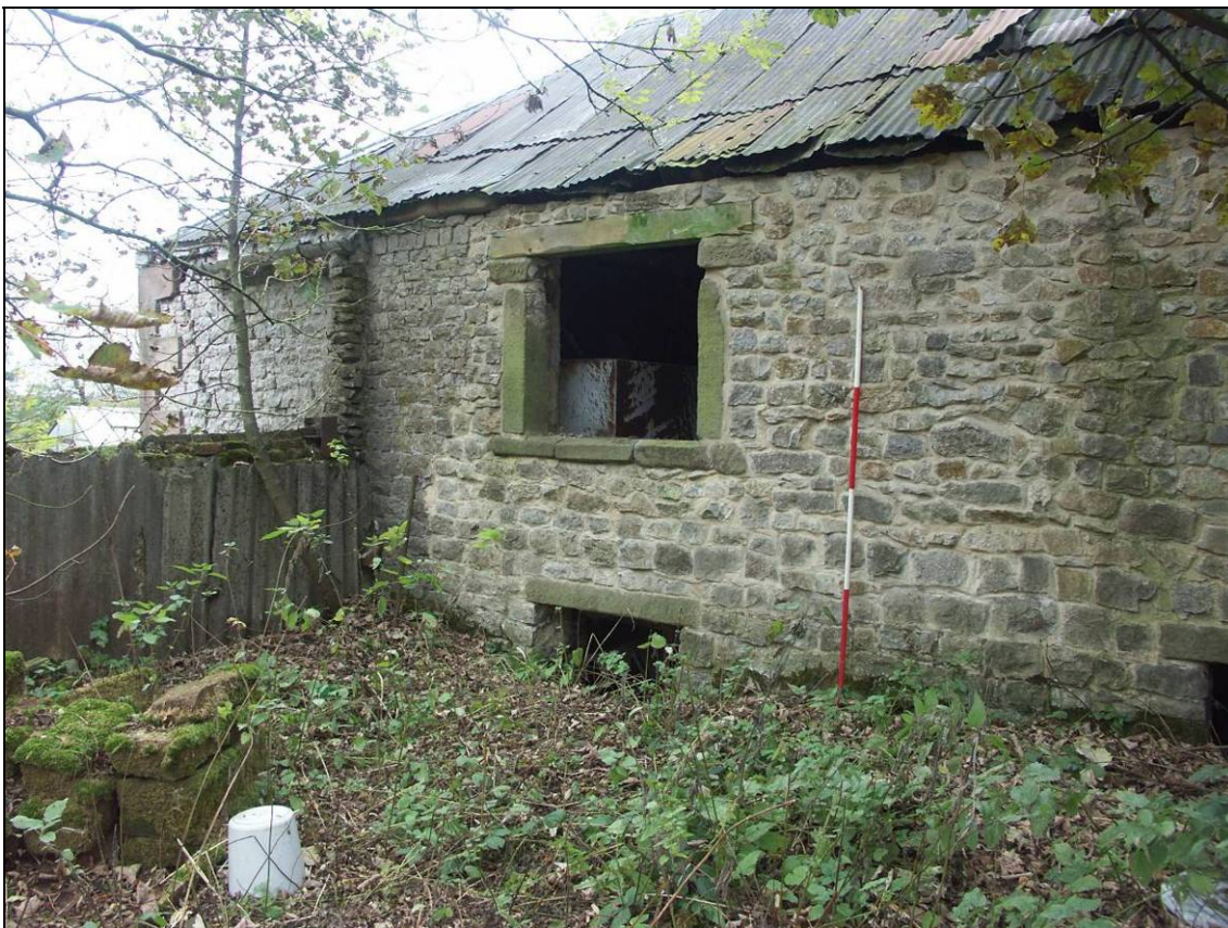
Figure 4: Detail of rebuilt area within the east elevation of the eastern wing (Block 3)
