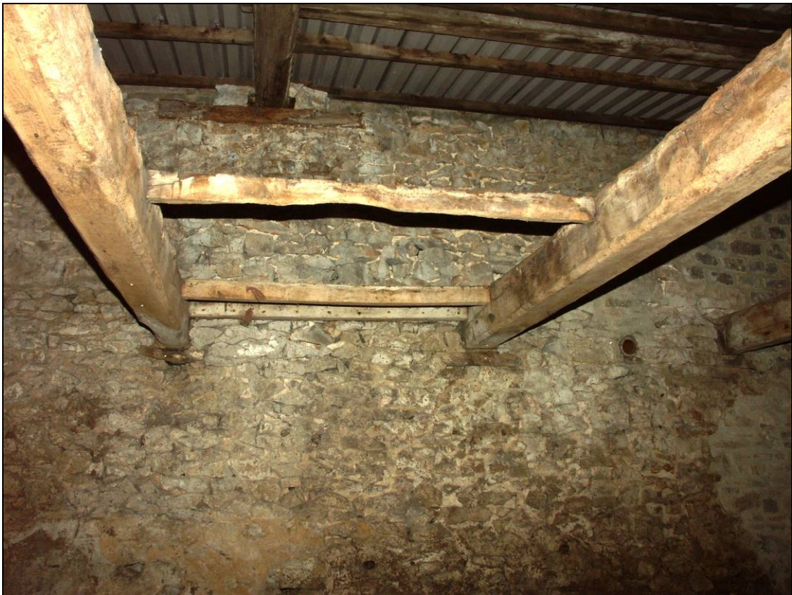
Figure 8: Bridging beams supported by timber pads within the northern section of Block 1
