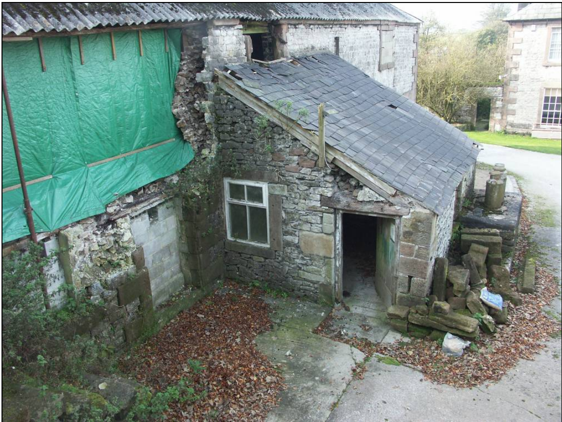
Figure 14: Small lean-to (Block 6) abutting the north elevation of the southern wing (Block 4)
