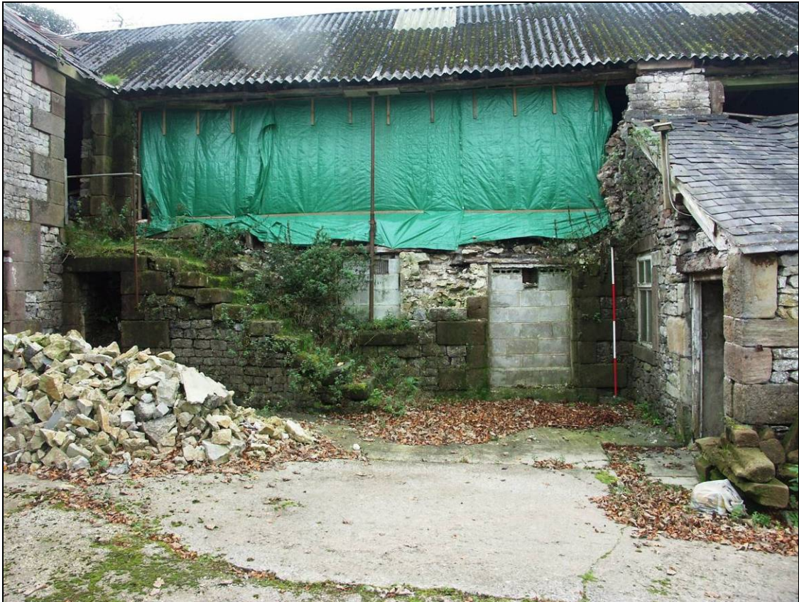
Figure 13: Detail of collapsed wall within the north elevation of the southern wing (Block 4)
