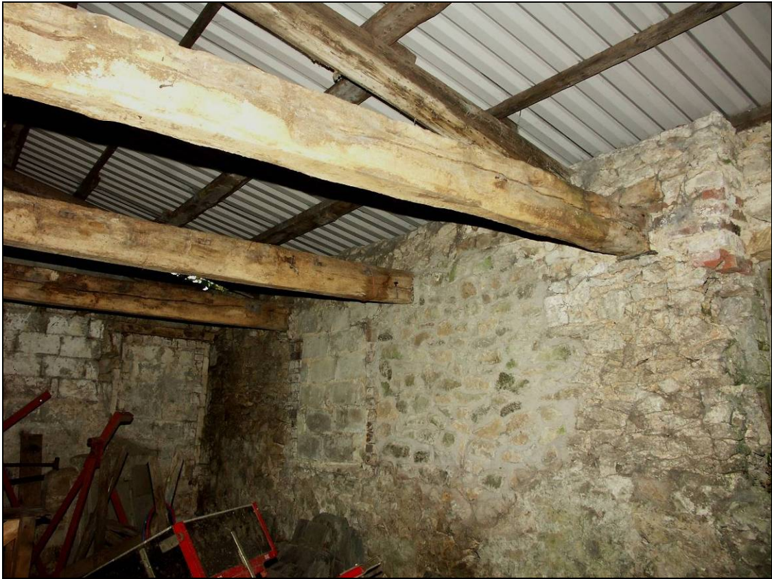
Figure 9: Opposite side of the bridging beams without support pads (Block 1)
