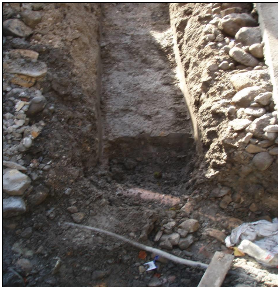
Fig 6. South facing view of trench. Ceramic pipe (004) evident at northern extent of trench.
