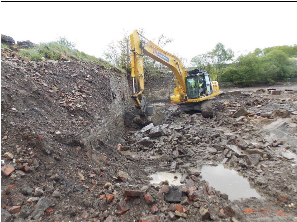
Figure 106: Excavation along the retaining wall of the small mill pond, looking south-west.
