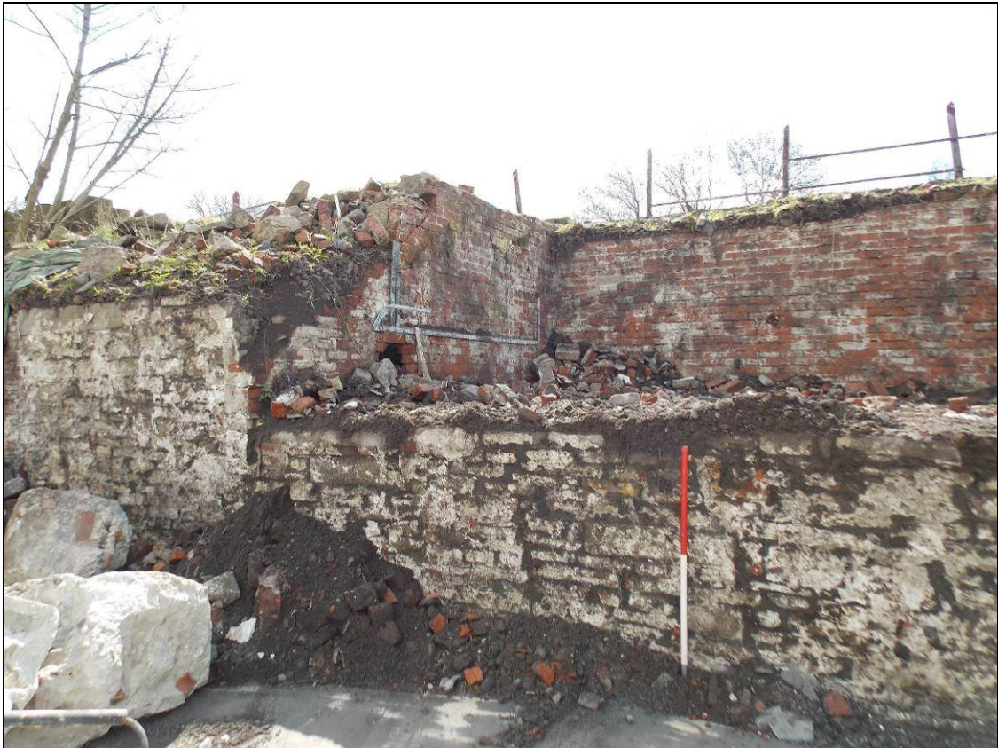
Figure 37: Easternmost area of the main wall and later brick-built extension, looking south-east (scale 1m).
