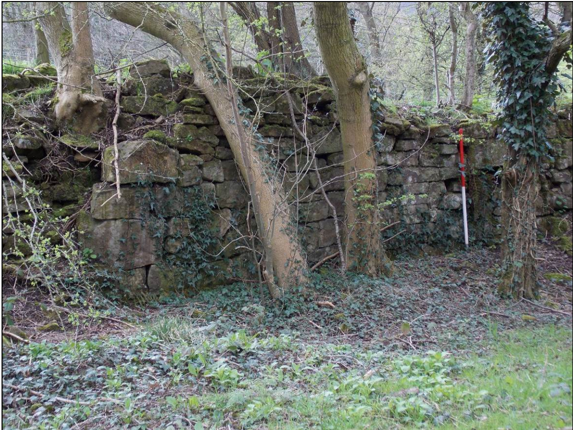
Figure 62: Detail of the southern wall of Structure M, looking south-west (scale 1m).
