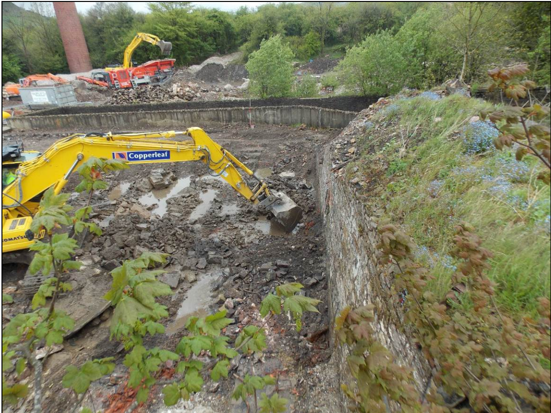
Figure 105: Excavation along the retaining wall of the small mill pond, looking north-east.
