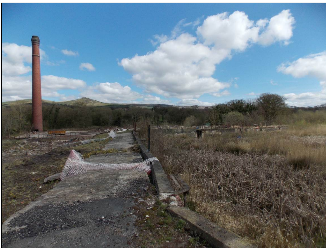
Figure 29: Large mill pond with retaining wall topped with concrete coping, looking north-east.
