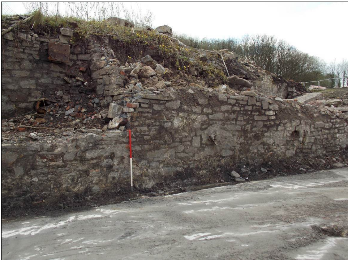
Figure 42: Western area of the main wall of Structure H, looking south-west (scale 1m).
