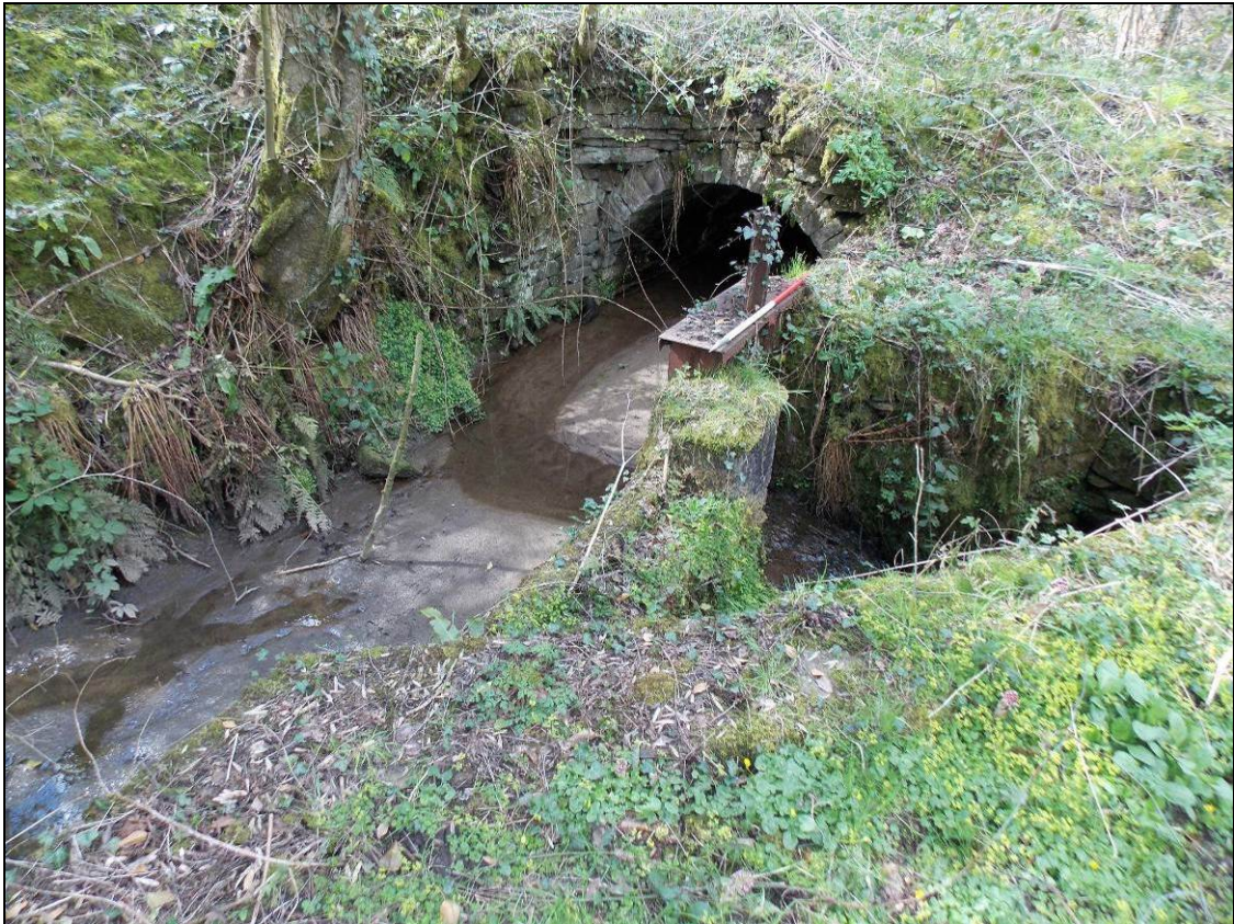
Figure 57: General view of the sluice, sluice gate and bridge, looking west (scale 1m).
