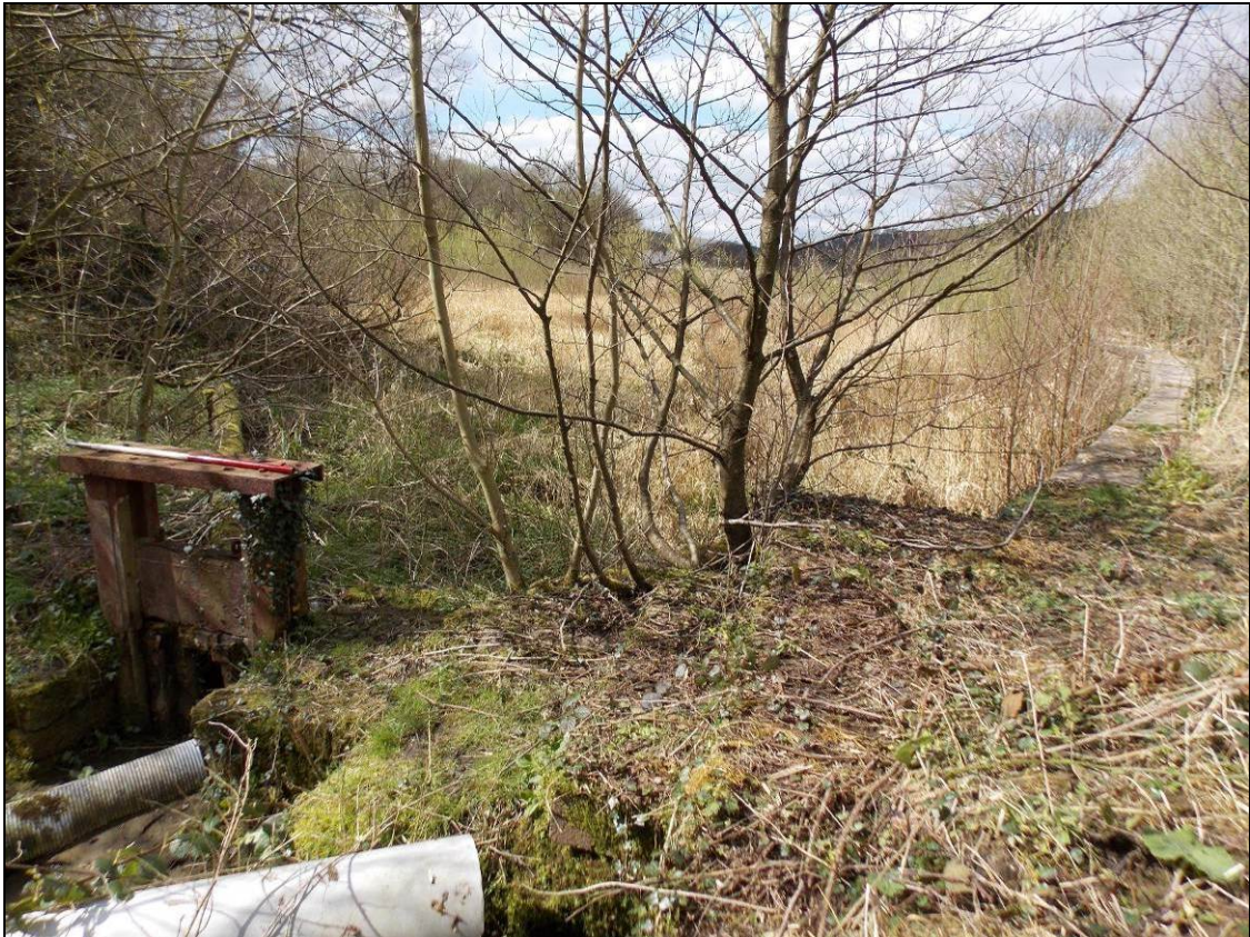
Figure 56: Sluice gate within the north-eastern corner of the large mill pond, looking north-west (scale 1m).
