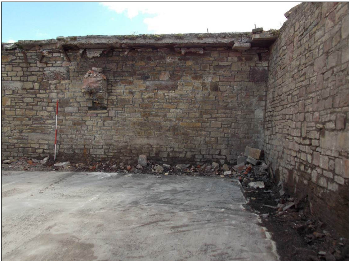
Figure 23: Southern side of the eastern wall of Structure E, looking south-east (scale 2m).
