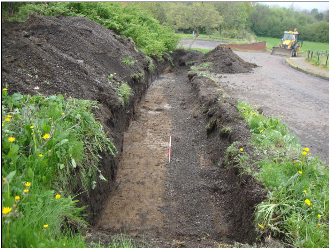
Figure 5: The trench showing the modern drainage pipe at the base of the trench to the right. Looking north, scale = 1m.
