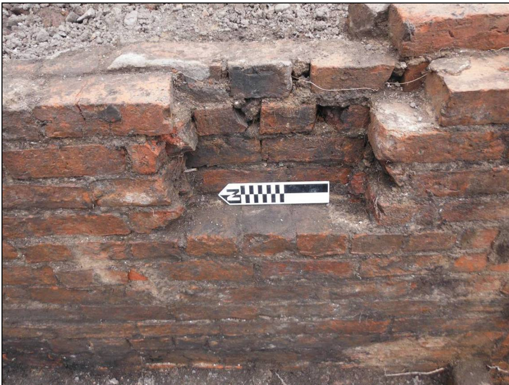
Figure 16. Possible purpose-built inset built into wall (220) to be used as a shelf, Trench 2. Scale = 0.25m.
