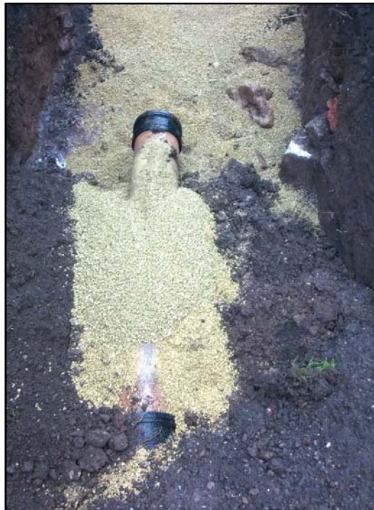
Figure. 7- Preservation of early modern ditch cut [104] using bedding gravel prior to installation of modern service piping
