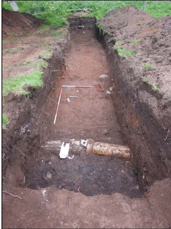
Figure.3 – NW facing shot of trench displaying service trench F.108 in the foreground and ditch F. 106 in the background (Scale- 1 x 1m, 1 x 2m)
