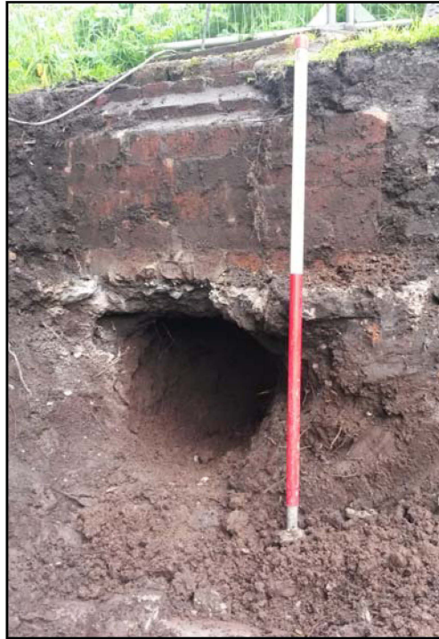
Figure. 8- Pipe access excavated through subsoil (002) below modern manhole at the northern extent of the trench (Scale- 1 x 1m)
