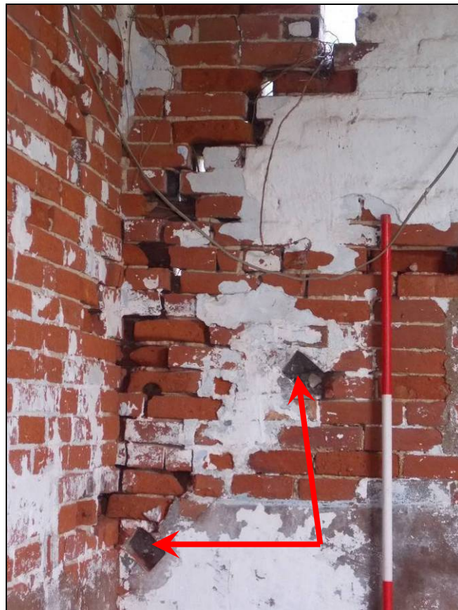
Plate 19: Detail of vacant sockets (arrows) of a former manger trough, looking east (scale 1m).
