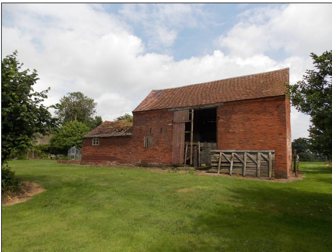
Plate 8: West elevation of Building A with extension (Building B) to the north, looking north-east.
