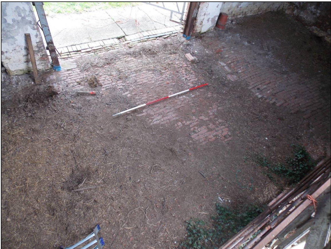
Plate 21: Brick floor within the central and southern bays, looking south-east (scale 2m).
