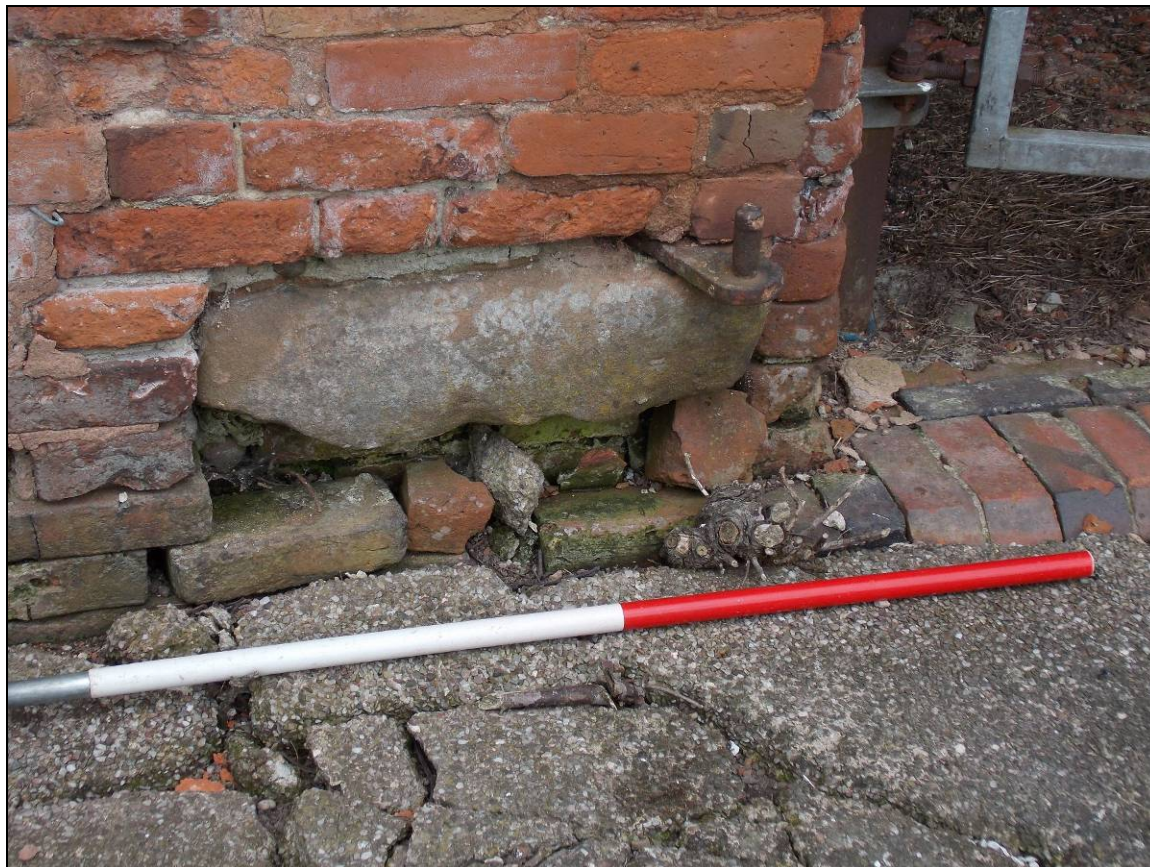
Plate 7: Detail of sandstone block with iron plate and pintle of door hinge, looking west (scale 1m).
