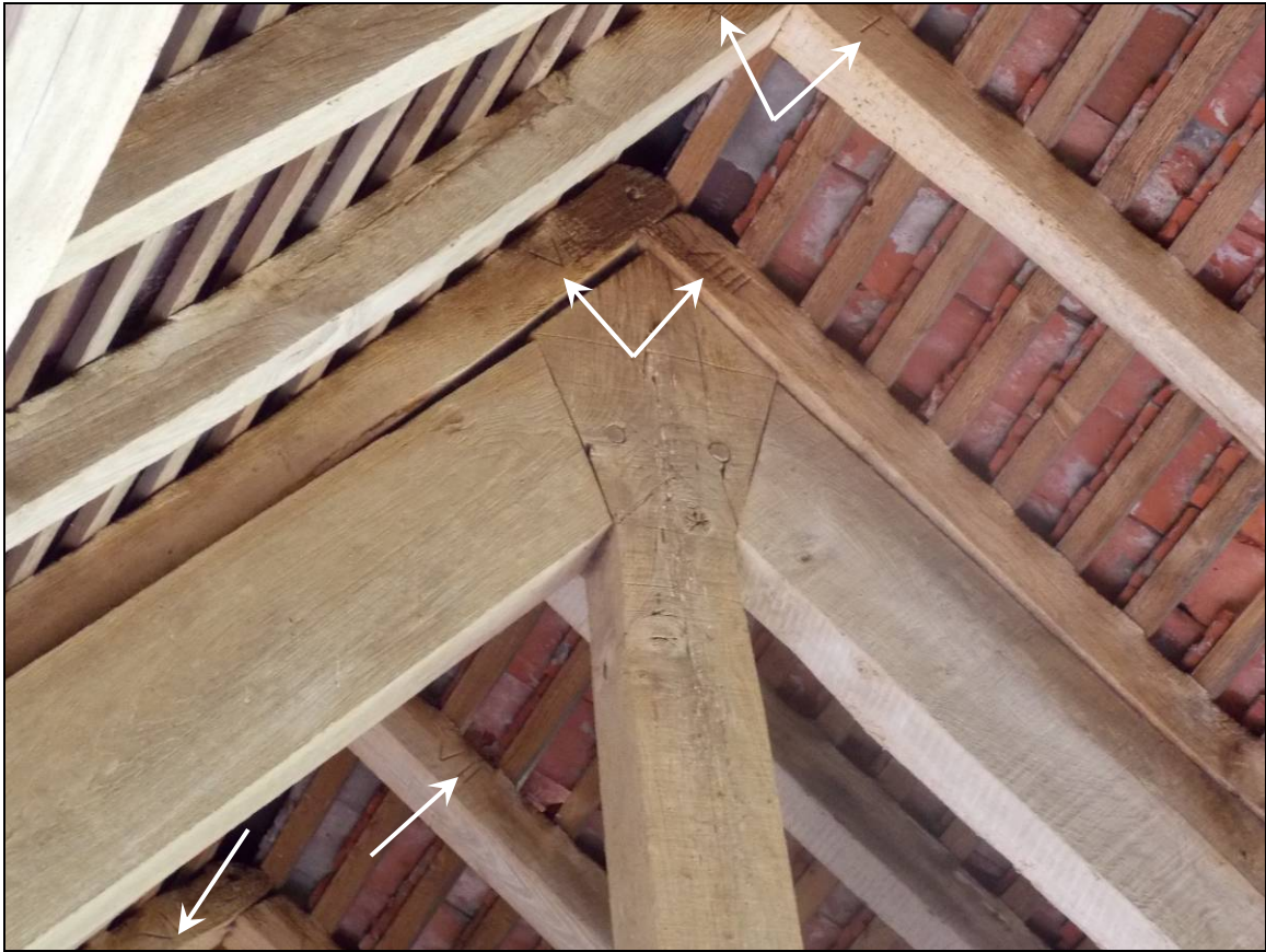
Plate 30: Upper section of truss I and carpenter's marks (arrows) within common rafters, looking south.
