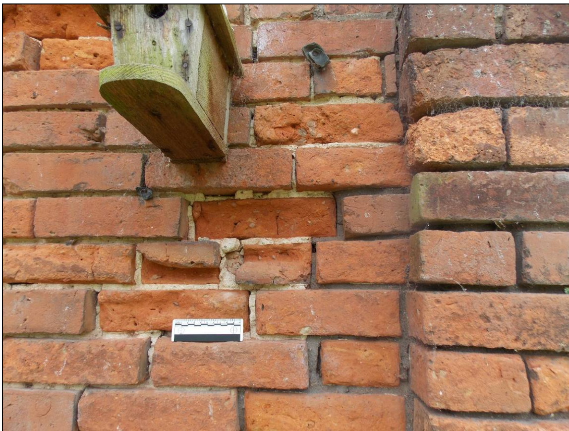
Plate 43: Detail of later brickwork repair with grey mortar bond, looking south (scale 10mm).
