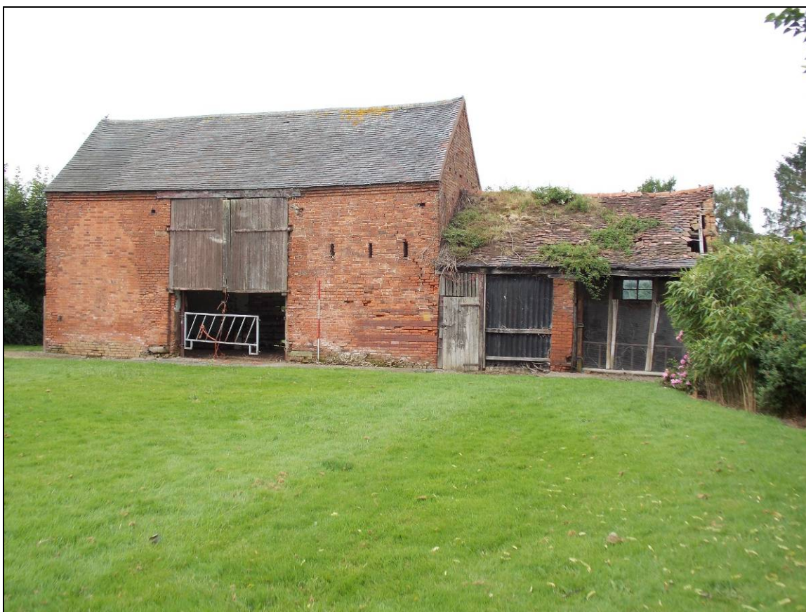
Plate 2: East elevation of Building A with open-fronted extension (Building B), looking west (scale 2m).
