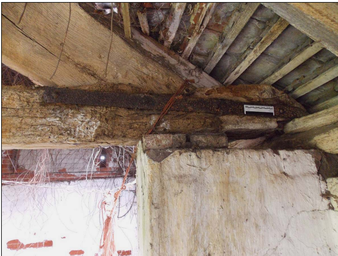
Plate 53: Western wrought-iron cramped tie, looking south (scale 100mm).
