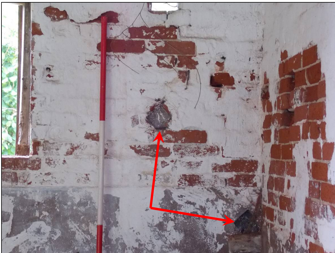
Plate 26: Detail of sockets (arrows) of a former manger trough, looking west (scale 1m).
