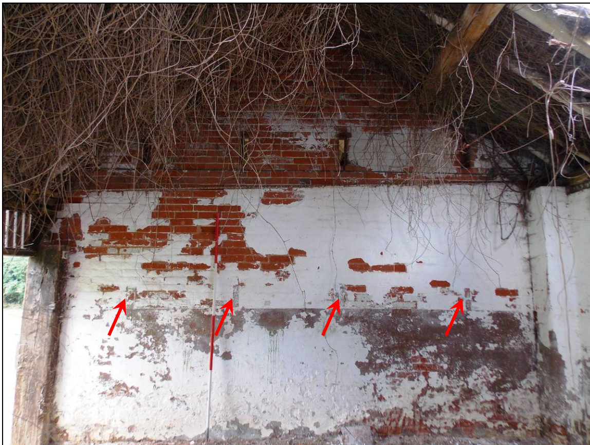
Plate 49: Internal south wall with blocked-up ventilation slits (arrows), looking south (scale 2m).
