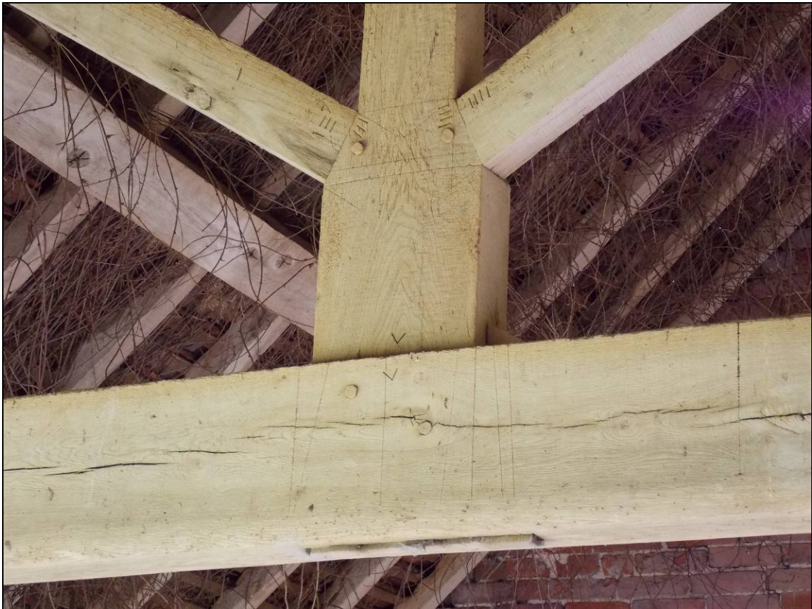
Plate 35: Truss II with several assembly carpenter's marks on the upper south face, looking north.
