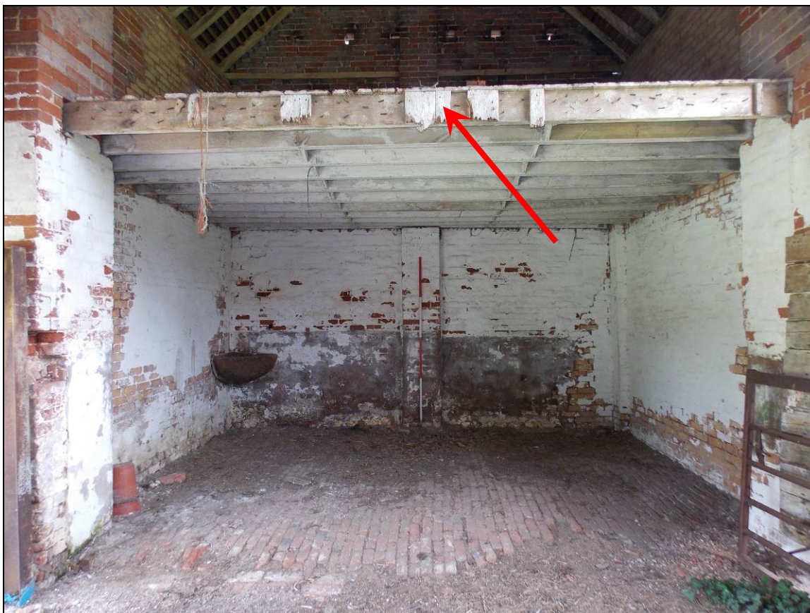
Plate 23: Upper storey with remnants of a former boarded screen (arrow), looking south (scale 2m).
