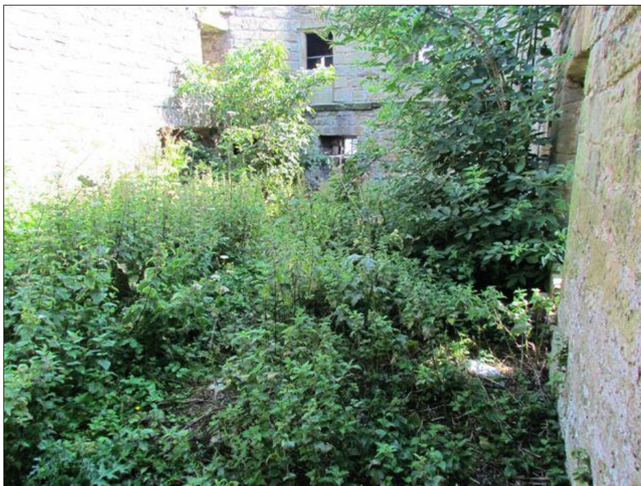
Figure 3: The appearance of the first-floor level of the tower prior to clearance works, looking west (Photograph Barry Mead).
