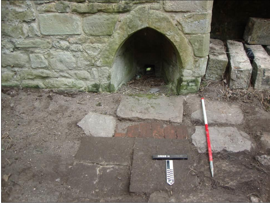
Figure 8: The brick and stone repair (004) adjacent to the slop hole in the south wall (scale = 1m).
