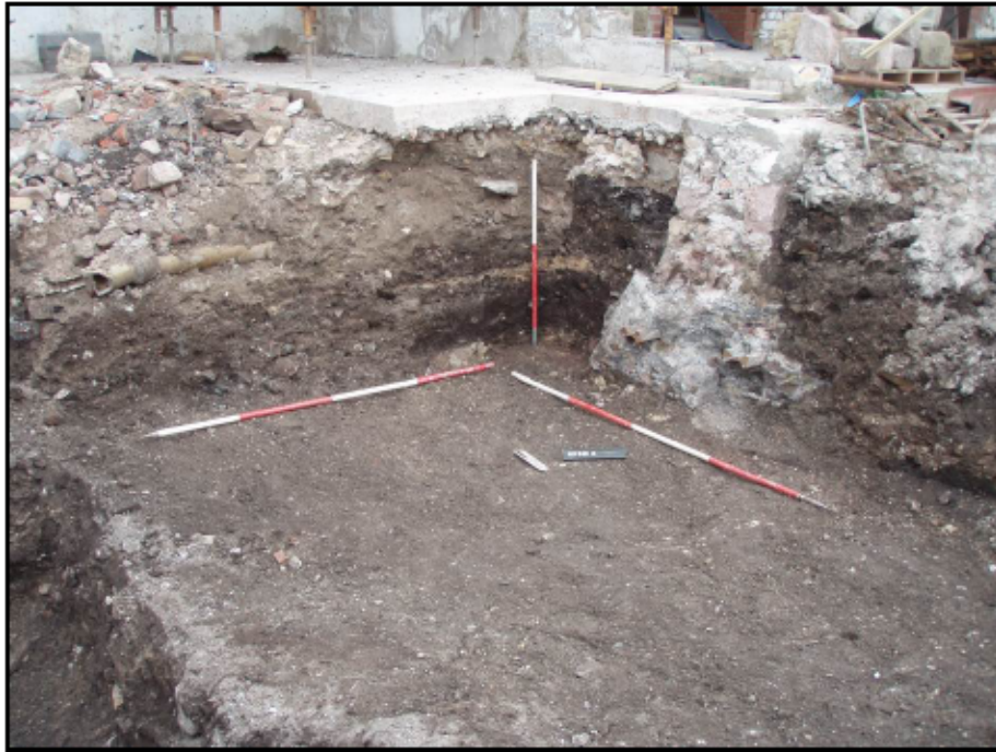
Figure 24 – South-west facing view displaying 20th century concrete foundation base (238), wall (215) and service trench F.225. See figures 39 (section points) and 40 (section).
