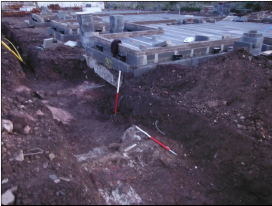
Figure 49 – North facing section of extended trench containing wall (241) and wall (249). (Scale = 2 x 1m).
