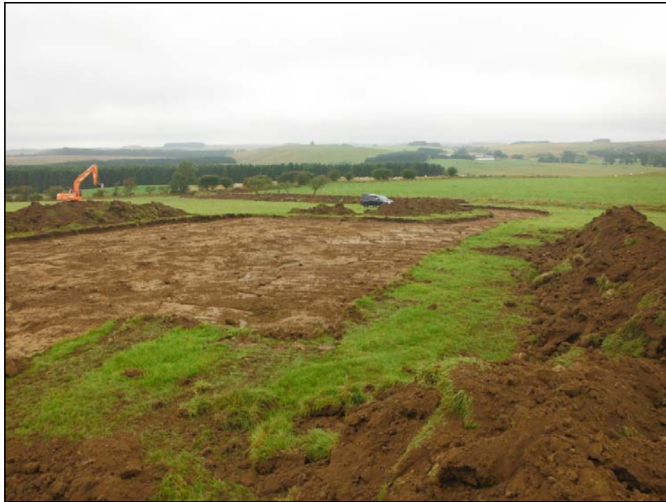
FIGURE 5: NORTH-WEST FACING POST-EXCAVATION SHOT OF SOUTH-EASTERN EXTENT OF WATCHING BRIEF AREA LOOKING TOWARDS DOVECOTE HILL
