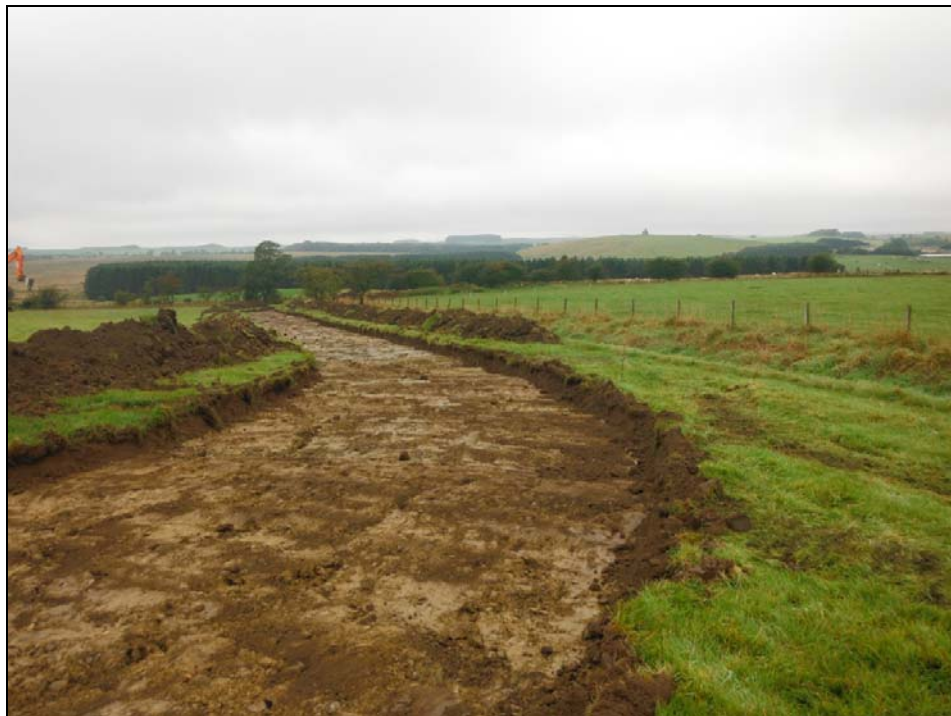
FIGURE 4: NORTH-WEST FACING POST-EXCAVATION SHOT OF EASTERN EXTENT OF WATCHING BRIEF AREA LOOKING TOWARDS DOVECOTE HILL
