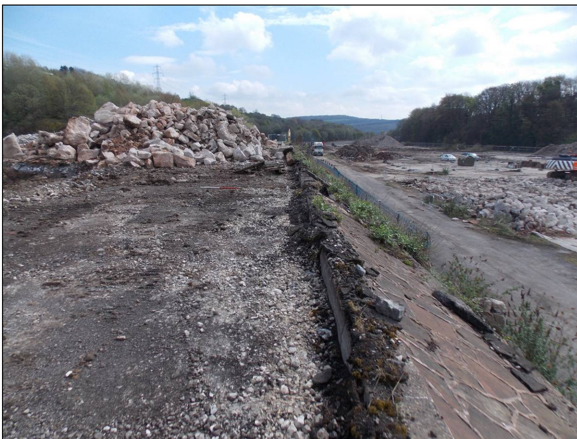
Figure 49: Sloping revetment along the southern edge of Area C, looking east (scale 1m).
