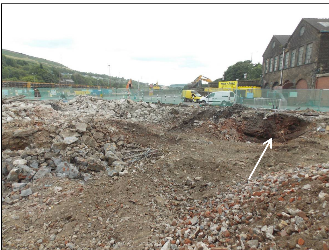
Figure 16: General view of Division A-4 with the remains of a chimney flue (arrow), looking east.
