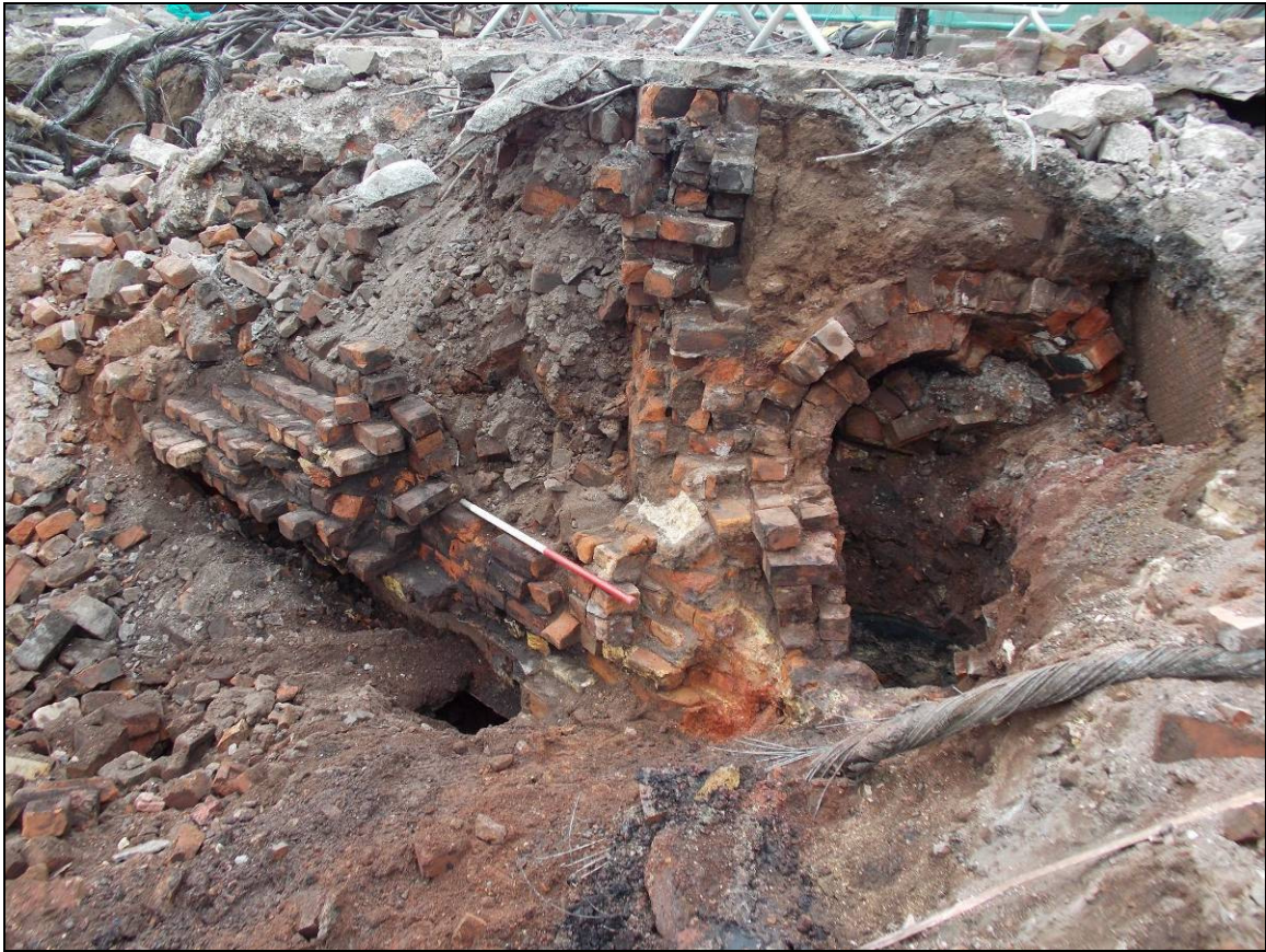
Figure 17: Chimney flue (113) abutted by a later brick-built structure (117), looking east (scale 1m).
