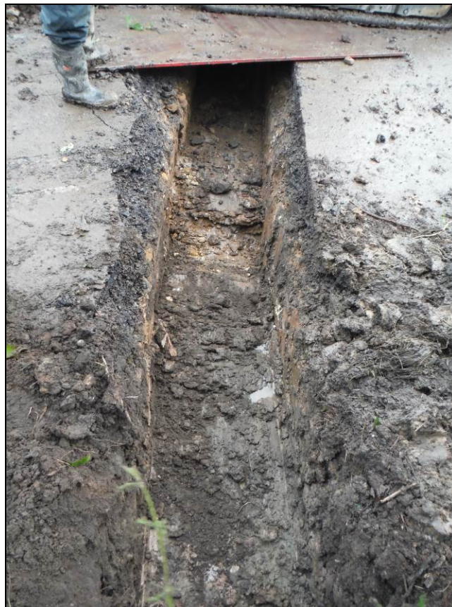
Figure 6. The pipe trench across the road showing tarmac, bedding and natural clay.
