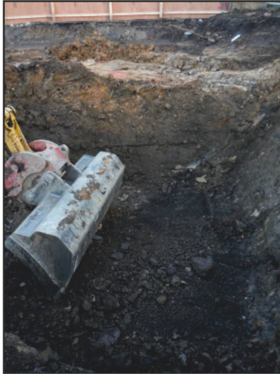
Figure 18: Phase 3, looking north, mechanical digger exposing dark grey clay deposits (413), (426) under re-deposited clay (414).
