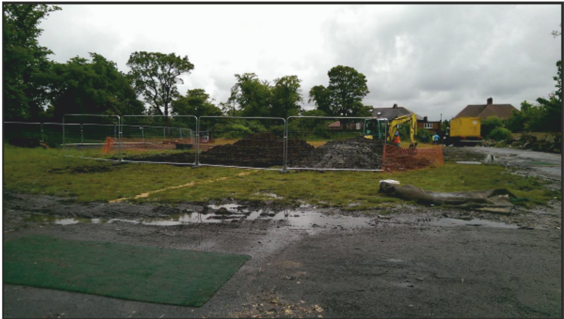
Figure 11: Phase 3 extent of site, looking south, illustrating road around perimeters and grassed area in centre.
