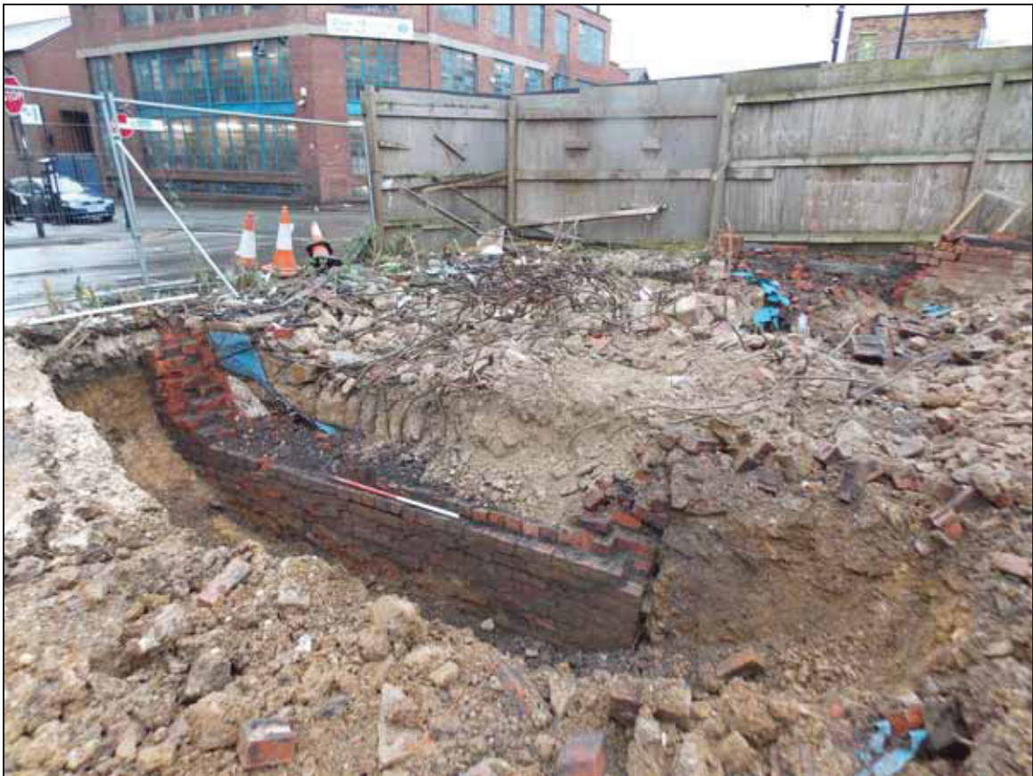
Figure 16: Brick-built cellar (111) within the southern corner of the site, looking south-west (scale 1m).
