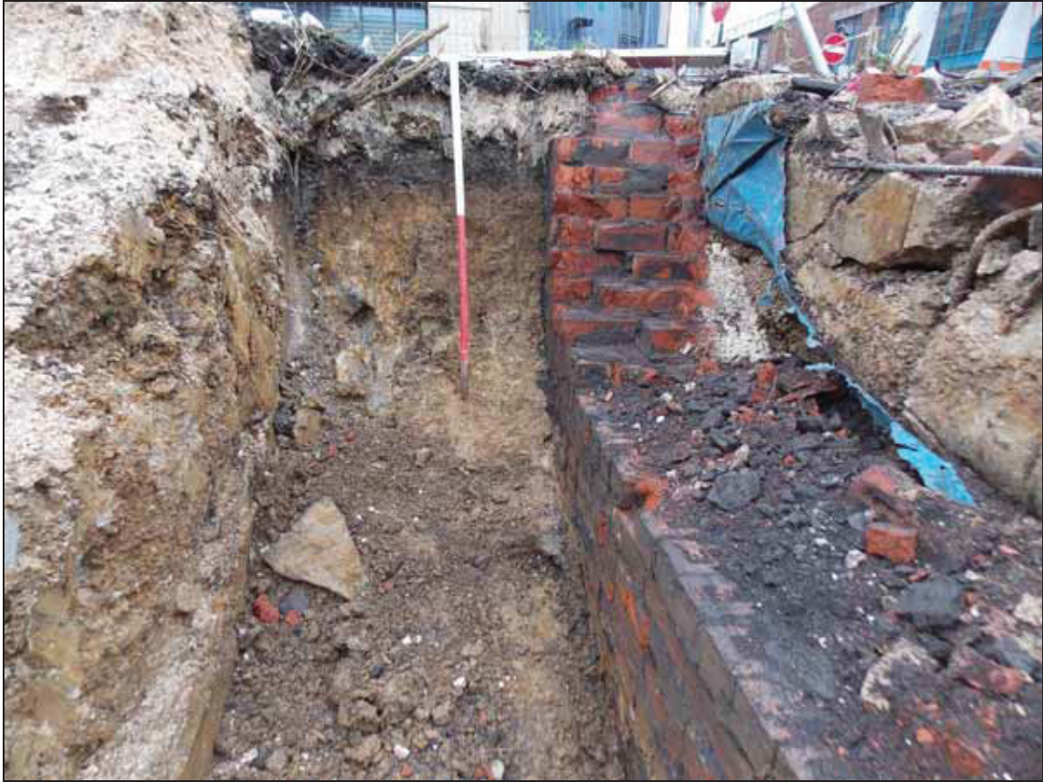
Figure 17: Sectional view of cellar (111) showing the construction cut [113], looking south-east (scale 1m).
