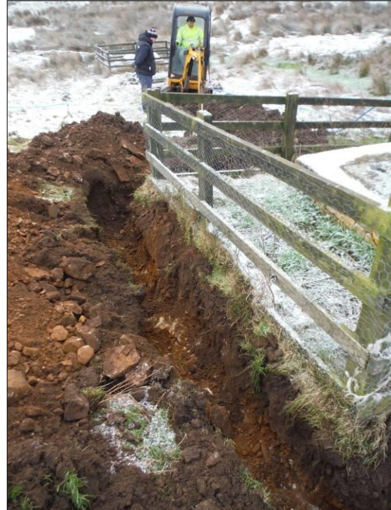
Figure 14: Trench 9 running around the east side of the existing man-hole, looking north-east (scale = 1m).
