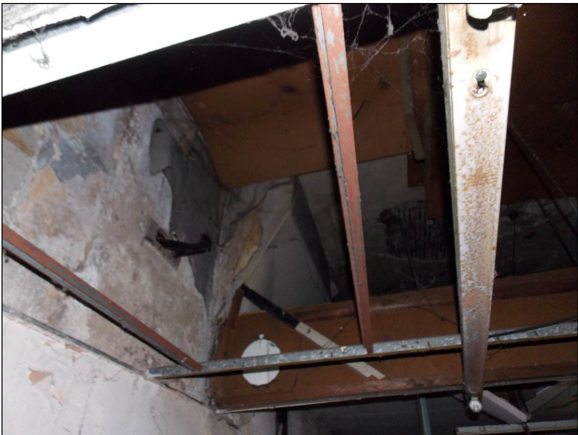
Plate 20: Truncated chimney breast within the north-western room of the ground floor, looking south-east.
