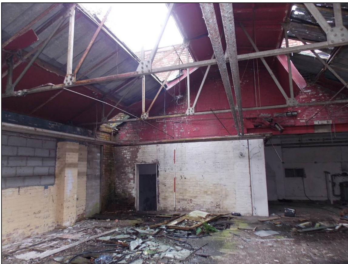
Plate 16: Part of the rear elevation viewed from inside a later extension, looking south-east (scale 2m).
