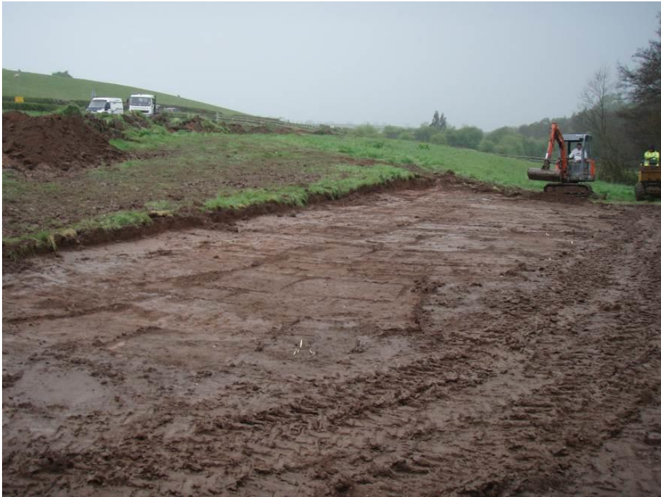
Figure 4. Area of Trench 2 where the topsoil was stripped, revealing the surface of the clay subsoil (102).
