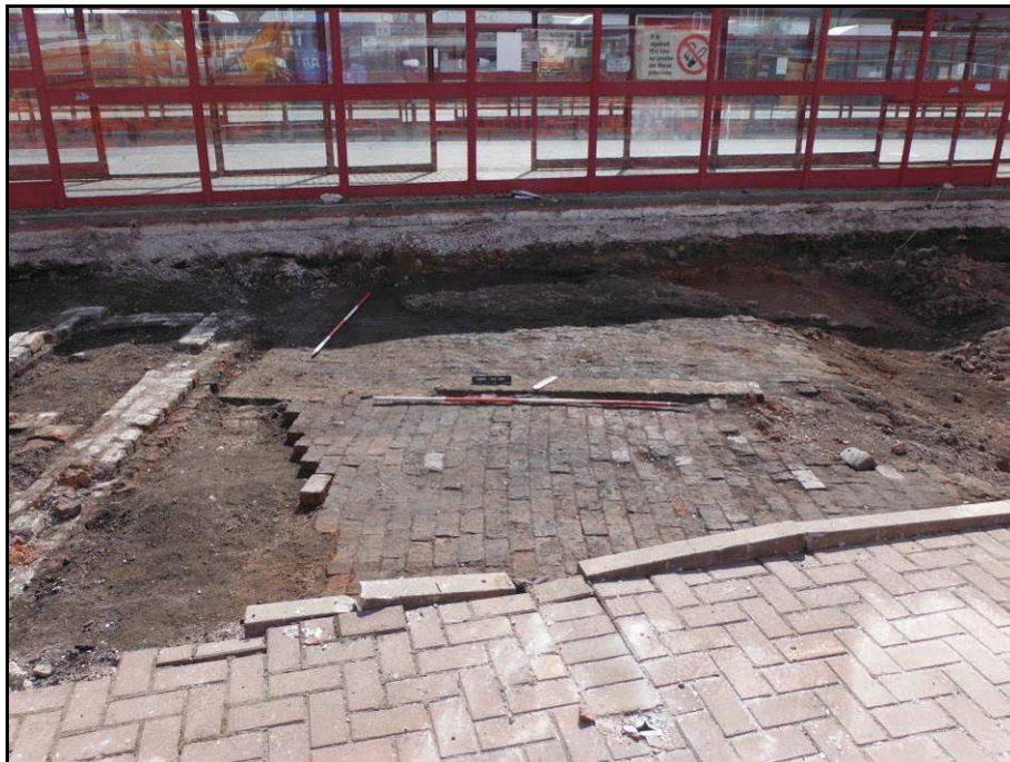
Figure 40- SW facing shot of surface (013), (015), partition wall (014) and walls (041)/(017) at the left hand side of the picture (Scale- 2 x 2m)
