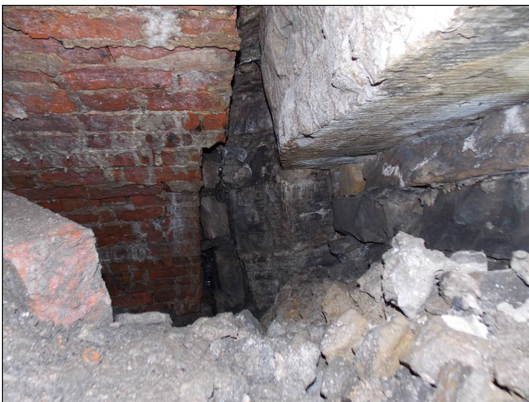
Figure 16: Detail of secondary infill between the brick vault and the external stone masonry of Catacomb.
