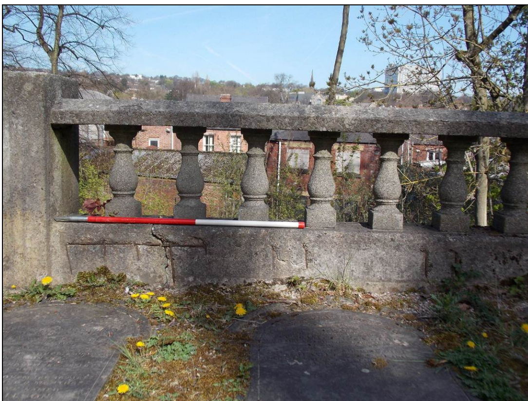
Figure 49: Plinth of balustrade showing exposed iron reinforcing cage.
