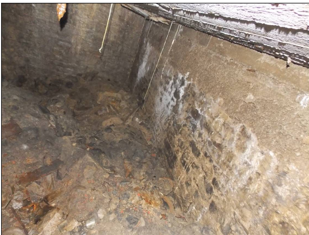
Figure 32: Internal view of Catacomb I with substantial deposited rubble.
