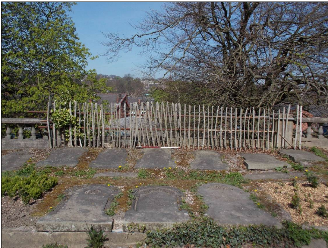
Figure 48: Section of the concrete parapet with missing balusters.
