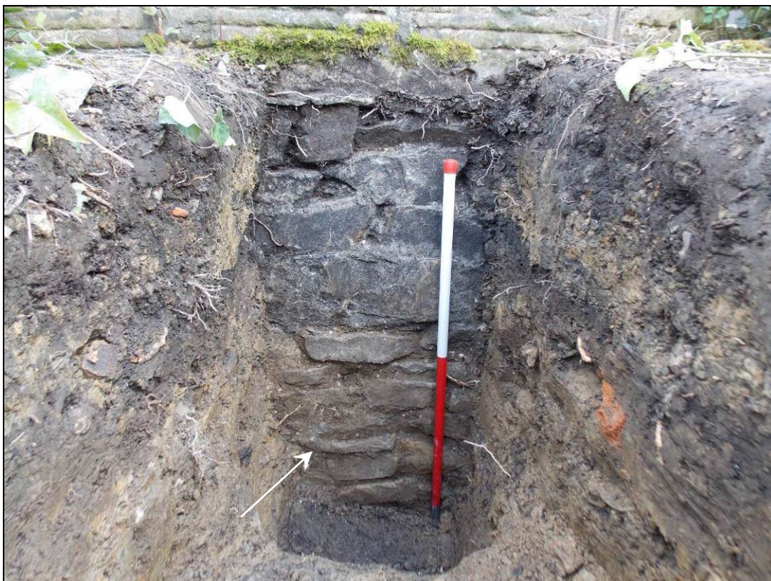
Figure 43: Test pit showing an earlier phase of construction beneath the foundation of the retaining wall.
