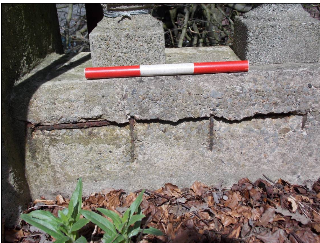
Figure 50: Detail of exposed reinforced cage and fracture.
