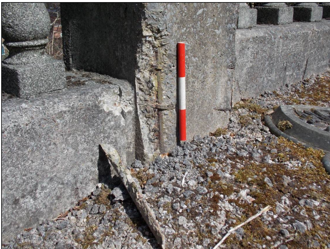
Figure 51: Exposed reinforced rod as a result of spalling.
