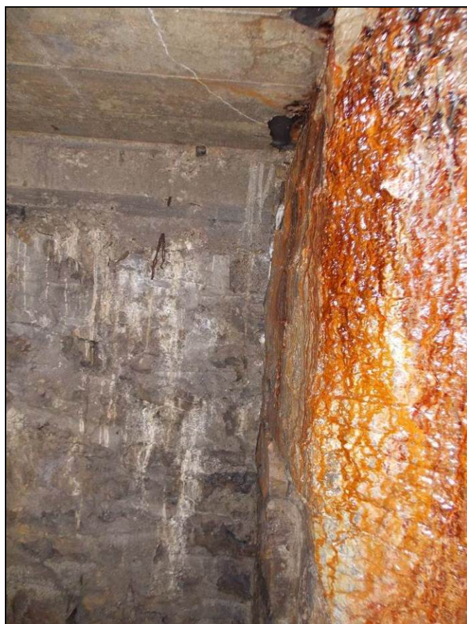
Figure 29: Further oxidation along the inner side of the blocked-up doorway.
