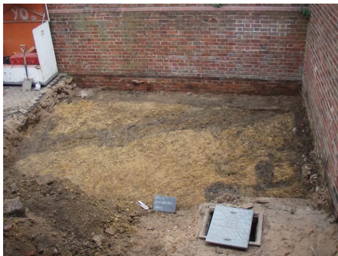
Drain running east-west across the site with manhole cover in the foreground.
