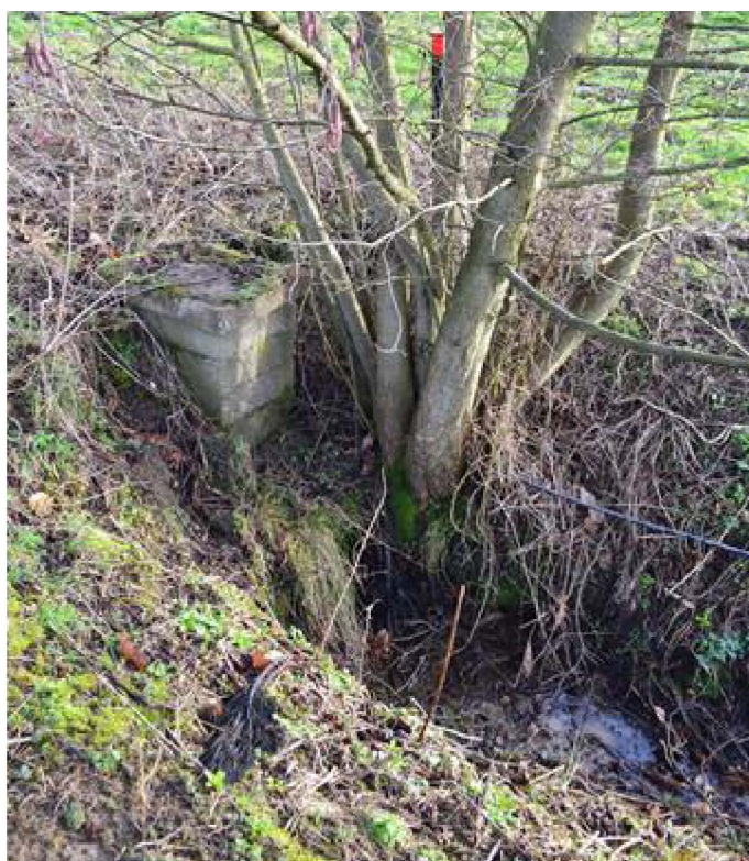
Figure 7: View NE at pipe and concrete housing at north end of ditch
