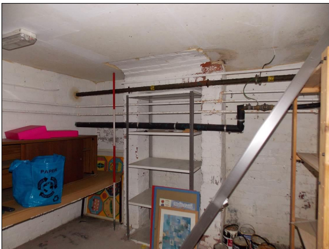
Figure 36: Cellar with brick pillars supporting the chimney breast within the Reception Room.
