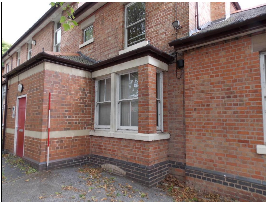
Figure 13: Eastern side of the south elevation showing inserted bay window and entrance porch.
