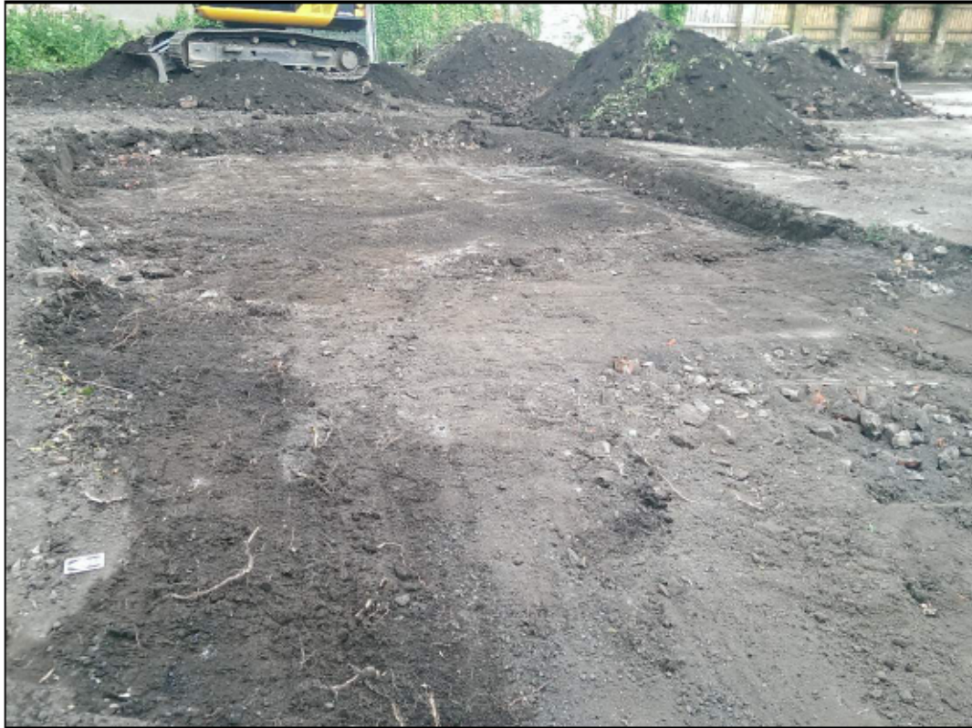
Figure 29: Area 2 following removal of the concrete pads (003 and 004) of the former structure. Facing east, showing context (002).
