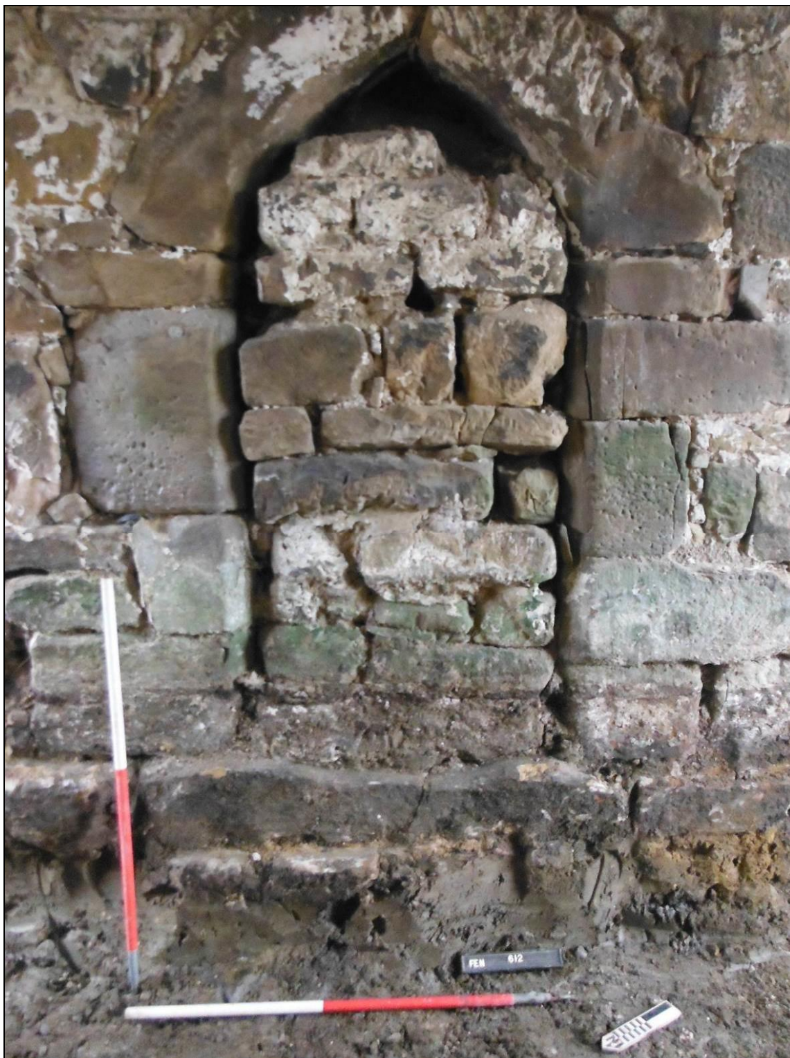
Figure 42- E-facing elevation of the 16 th -17 th century byre doorway within the western gable end wall of the bastle (Scale- 2 x 1m)
