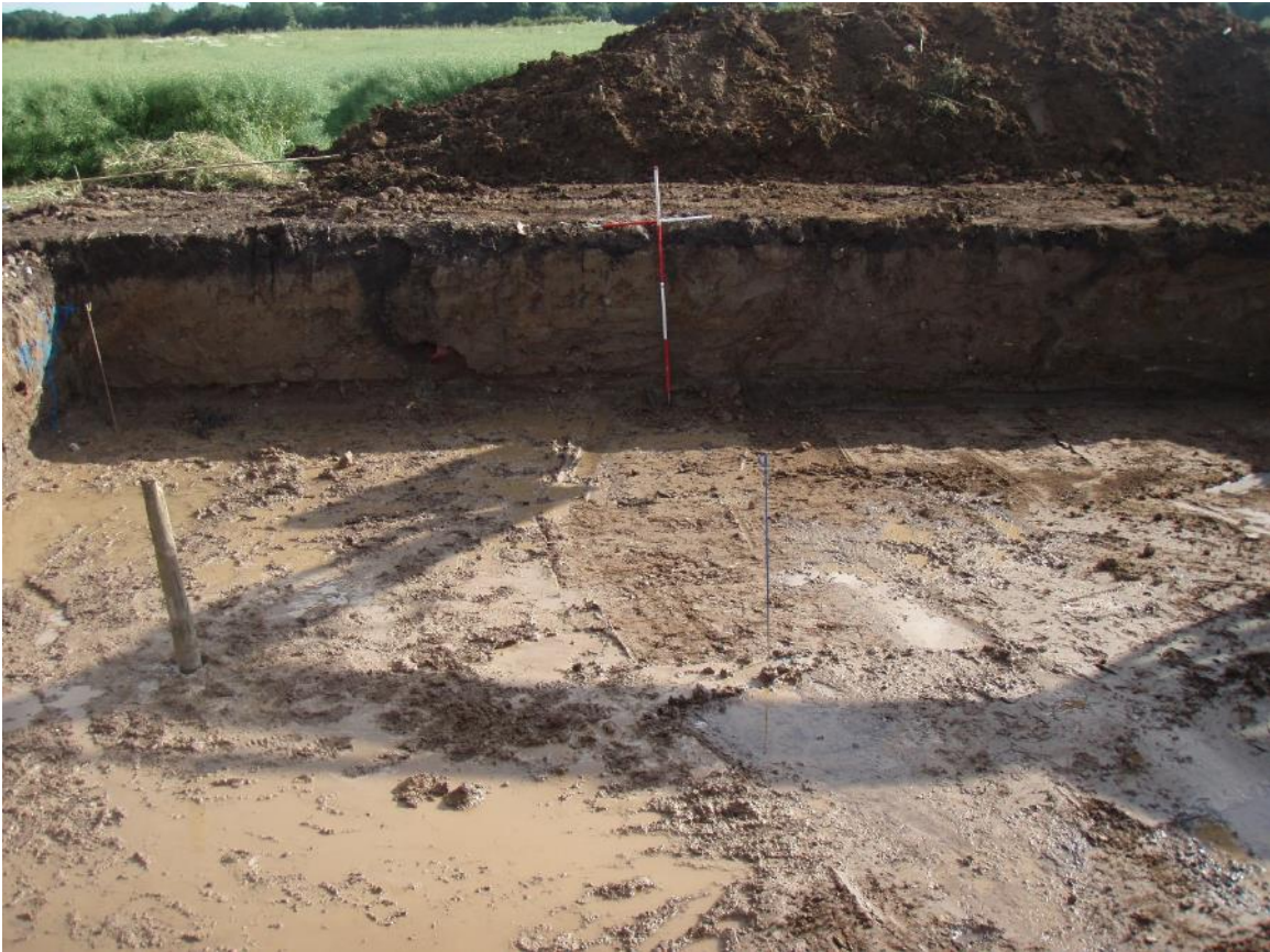
Figure 9. Section of turbine foundation looking south west showing topsoil (001), the natural geology (002) of the site and a modern land drain.
