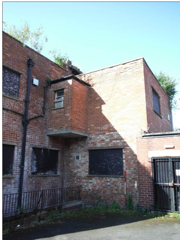
Figure 18: Detail of alterations to the north-east elevation of Building A (Scale = 2m).
