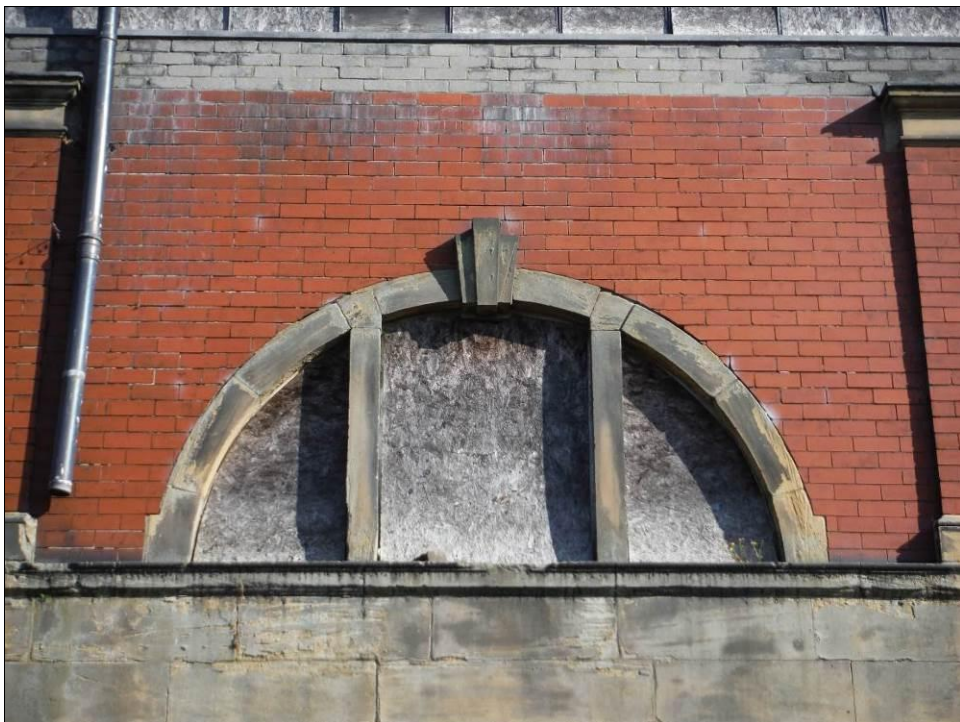
Figure 15: Detail of easternmost Diocletian window in the South East elevation of Building A.
