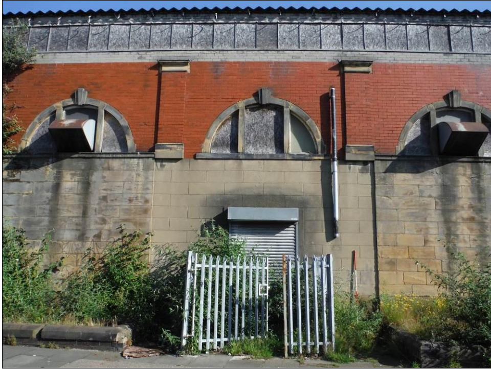
Figure 16: Detail of the scar of the original porch in the South East elevation of Building A (Scale = 2m).
