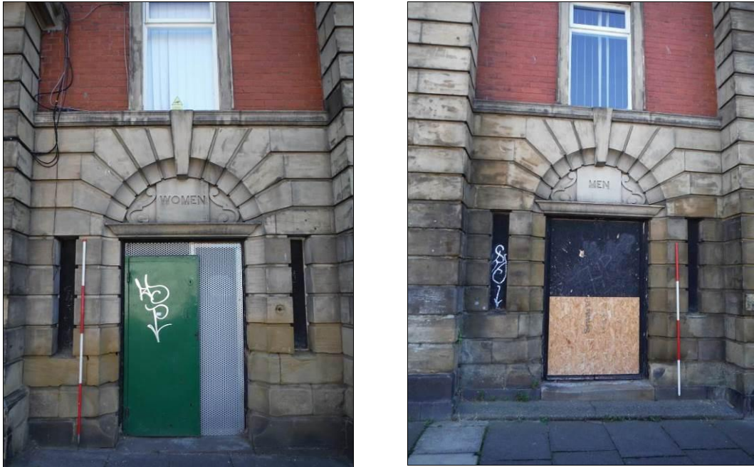
Figure 9: Detail of Mens' and Womens' entrances in South West elevation (Scale = 2m).
