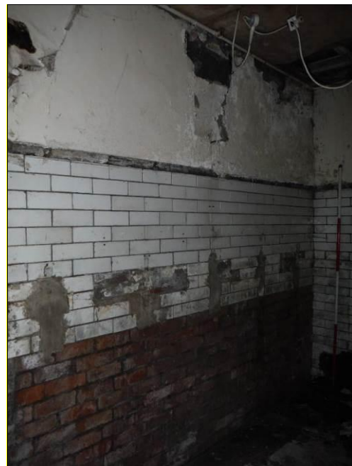
Figure 61: North wall of Room G12 showing the location of former urinals (Scale = 2m).
