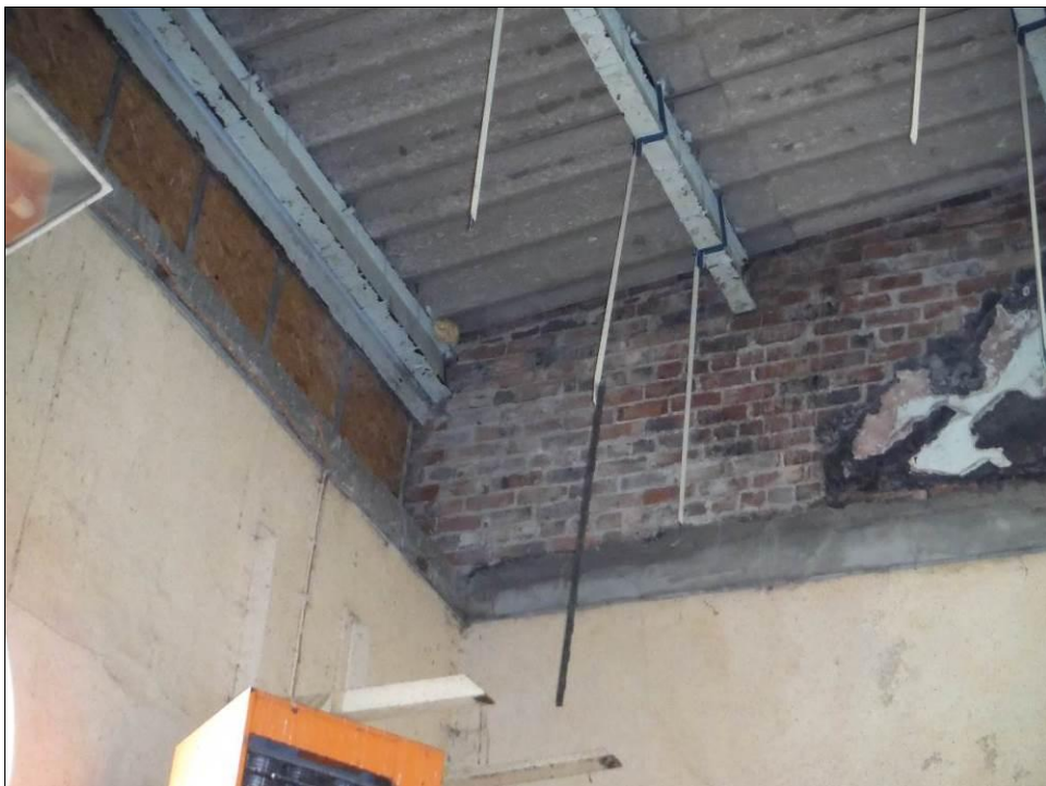
Figure 27: Detail of roof extension in the west wall of Room G1 in Building A.
