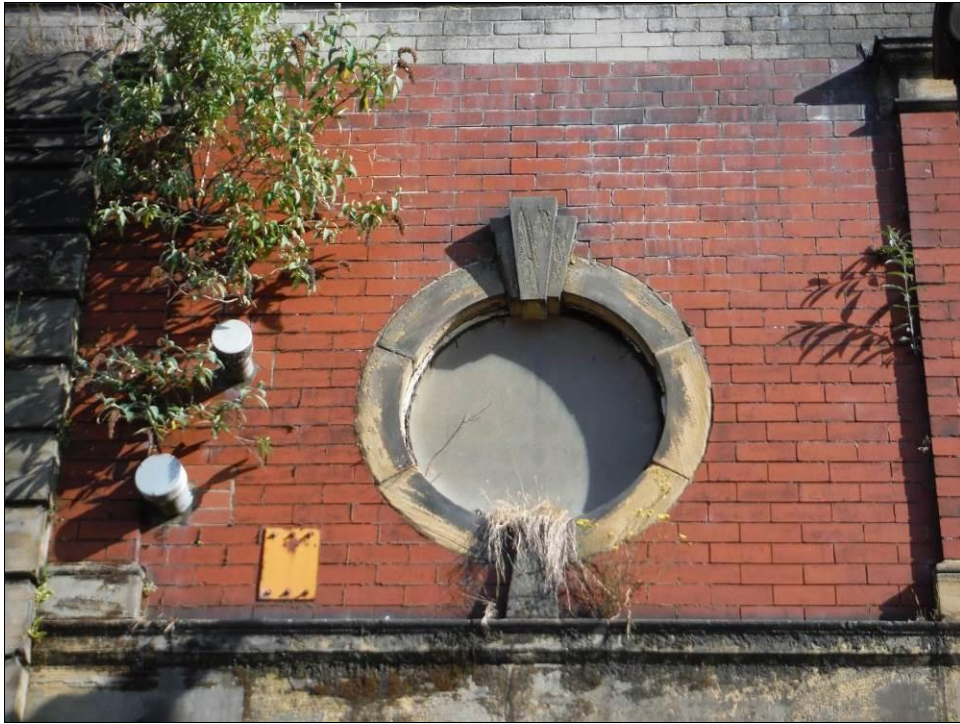
Figure 14: Detail of the westernmost roundel window in the South East elevation of Building A.
