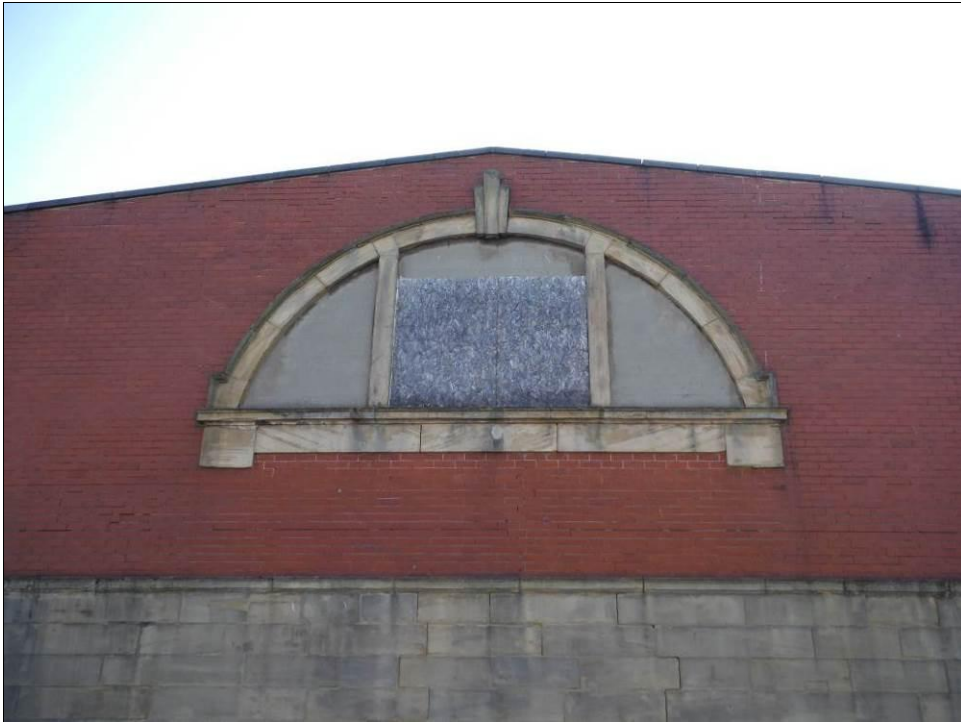
Figure 11: Detail of the Diocletian window in the South West elevation in main pool Building A.
