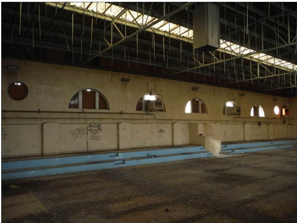
Figure 21: South facing oblique view of the south wall of Room G1 in Building A (Scale = 2 x 2m).
