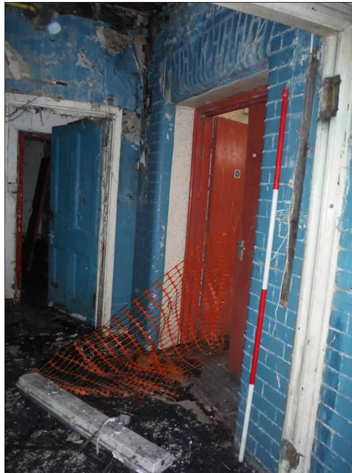
Figure 38: Detail of brick-built original doorway in south wall of Room G2, Building A leading to Room G1 (Scale= 2m).
