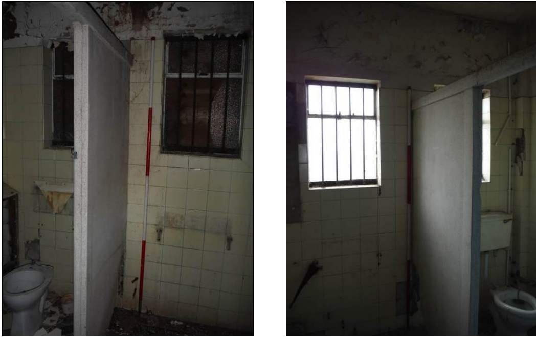
Figure 118: East wall of Rooms F2 (left) and F3 (right), Building B (Scale = 2m).
