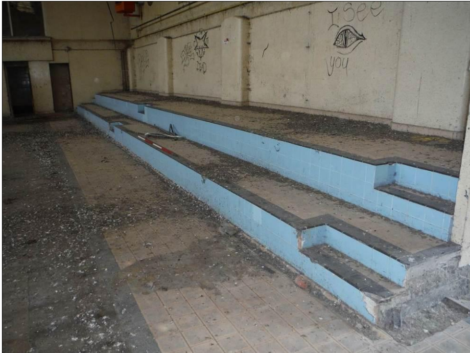
Figure 22: Detail of poolside steps on the south wall of Room G1 in Building A (Scale = 2m).
