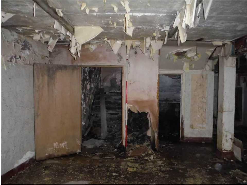
Figure 108: Detail of stairway in south-east corner of Room B5, Building B (Scale = 2m).
