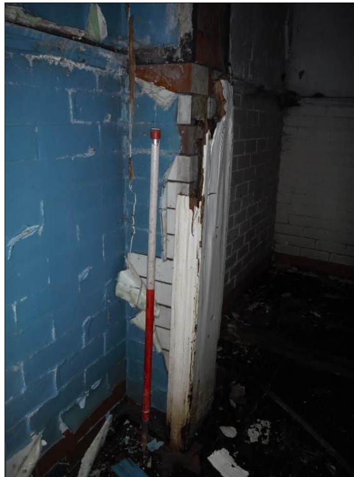
Figure 49: Detail of timber-moulded doorframe leading from Room G7 to Room G8 (Scale = 1m).
