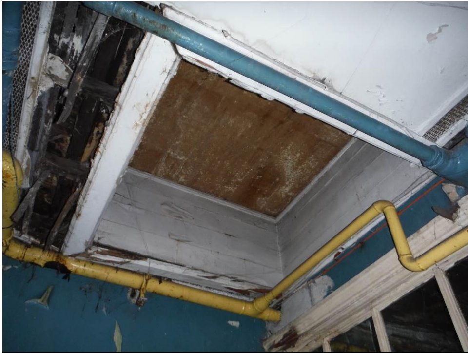
Figure 50: Detail of timber skylight in Room G7, Building A outside the entrance to Room G8.
