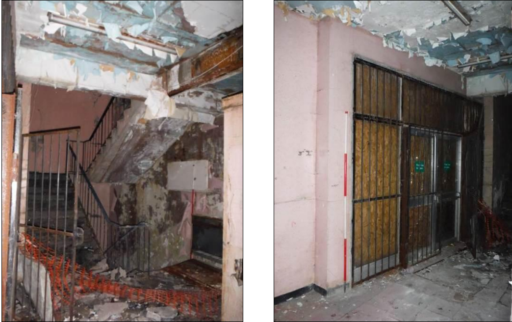
Figure 84: West wall (left) and south wall (right) of Room G5, Building B (Scale = 2m).
