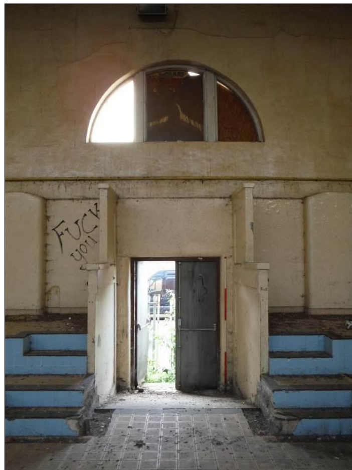
Figure 23: Detail of doorway and Diocletian window in the south wall of Room G1 in Building A (Scale = 2m).
