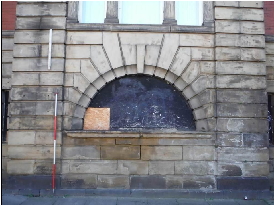
Figure 8: Detail of the ground floor Diocletian window in South West elevation (Scale = 2m).
