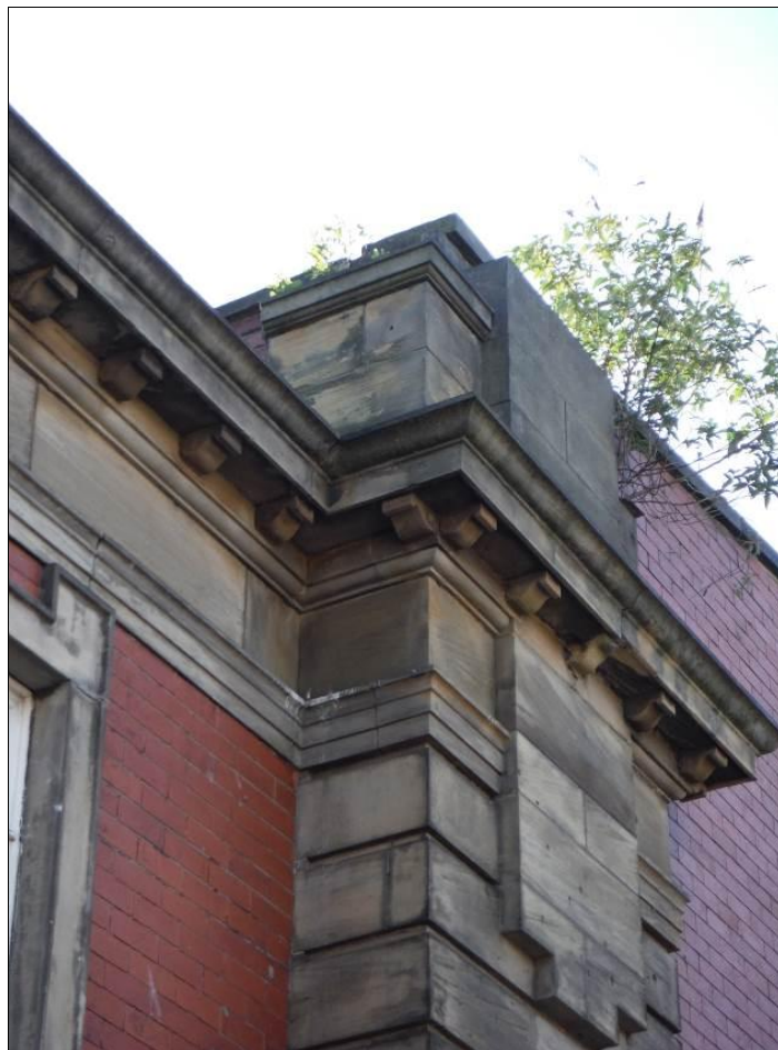
Figure 10: Detail of north-western corner pilaster of Building A pool building showing corning on the South West elevation.
