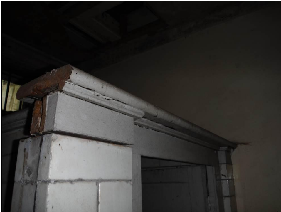
Figure 41: Detail of moulded cornice on toilet cubicle in Room G4, Building A.
