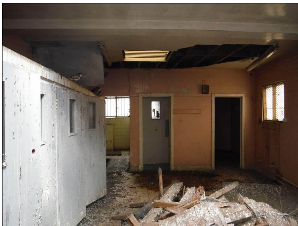
Figure 92: Room G11, Building B with Room G15 visible at the far left of the photograph.
