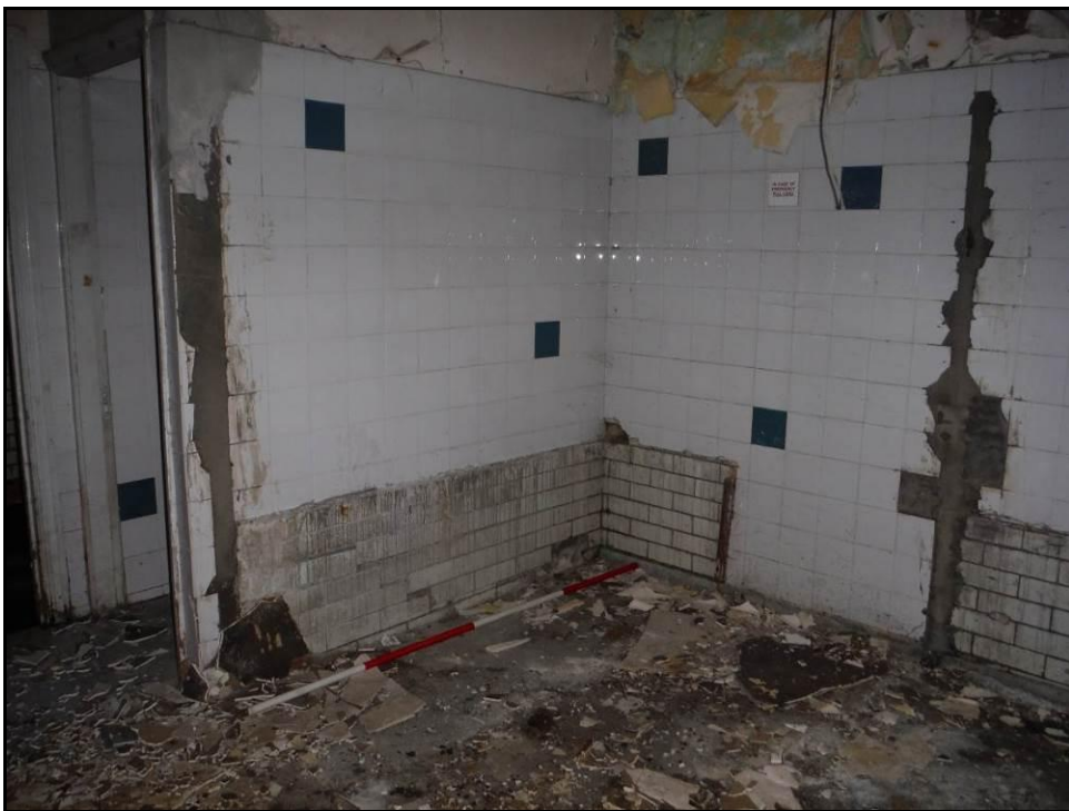
Figure 58: Detail of former bath and cubicle scars in the north west corner of Room G9 (Scale = 2m).
