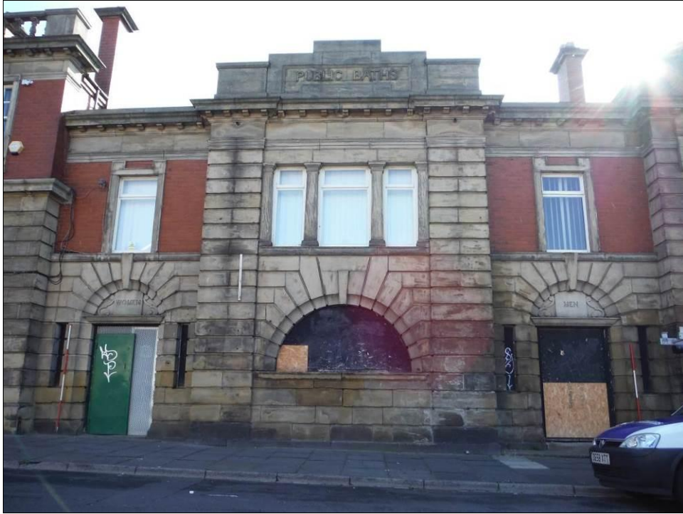
Figure 5: East south east facing view of the South West elevation of Building A (Scale = 2 x 2m).
