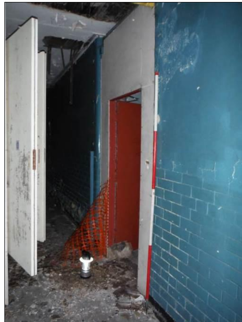
Figure 35: Detail of door in south wall of Room G2, Building A leading to Room G3 (Scale = 2m).
