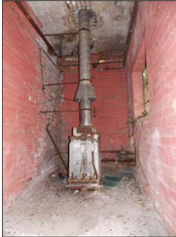
Plate 65: Gas boiler, looking south-east.
