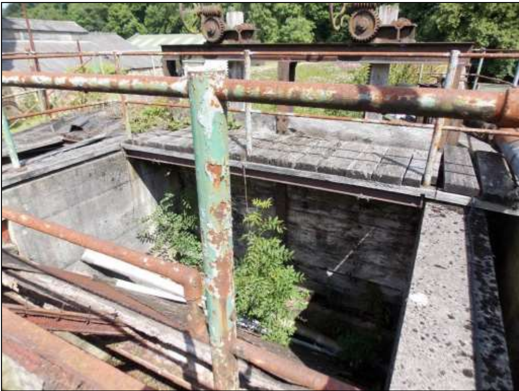
Plate 11: Penstock with sluice gate's mechanism and trash rack or grill, looking north.
