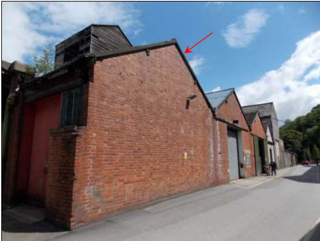
Plate 69: Gable wall of Units 5a (arrow) along the main access road of the works, looking east.
