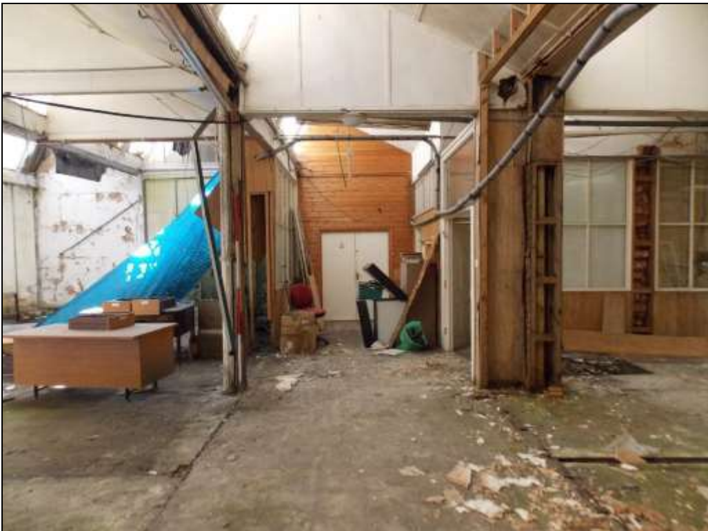
Plate 27: Office block (right) and inserted doorway to Fearnough House (centre), looking east.
