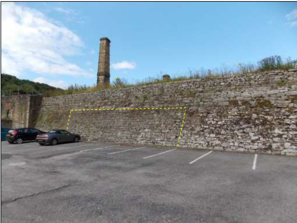
Plate 30: Retaining wall of the mill race with an area devoid of vegetation (yellow lines), looking south-west.
