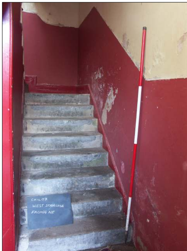
Fig. 33 Western staircase facing north-east showing concrete infilling to worn sandstone steps, scale 2m
