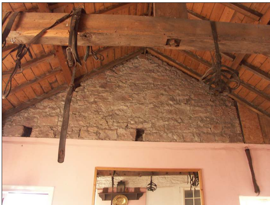
Fig. 43 Joist holes in north-west wall of Room Five
