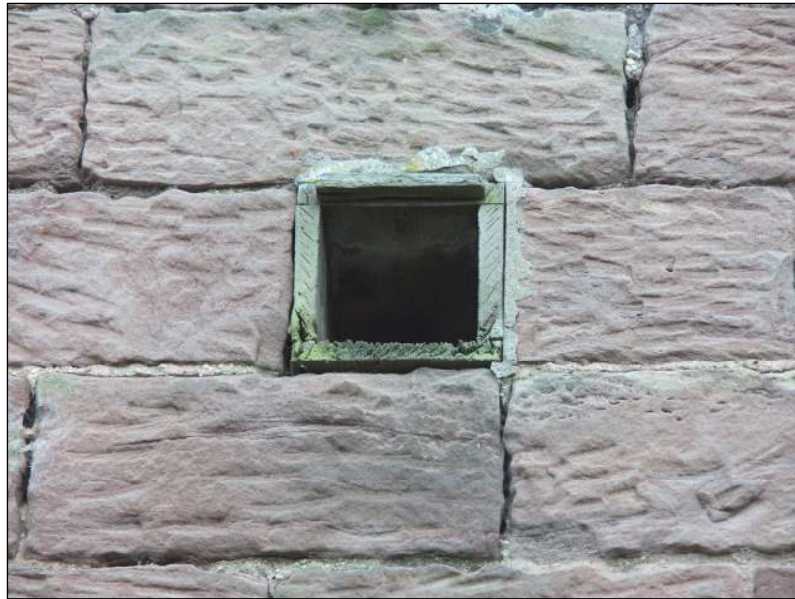
Fig. 9 Pigeon trap at western end of north-east facing elevation
