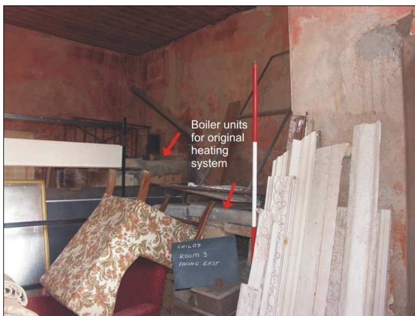
Fig. 30 Room Three facing east, the old heating system is indicated, scale 2m
