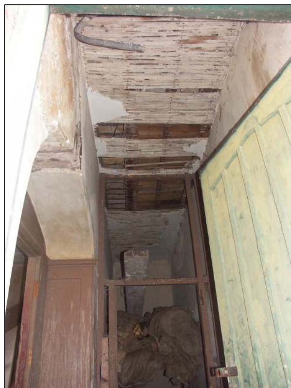
Fig. 34 Damage to ceiling in western central passageway
