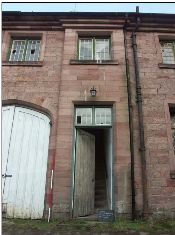
Fig. 21 South-west facing elevation showing the window above the east central doorway, scale 2m
