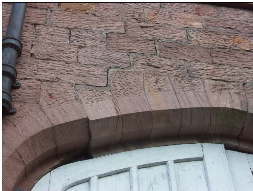
Fig. 19 Damaged archway in south-west facing elevation
