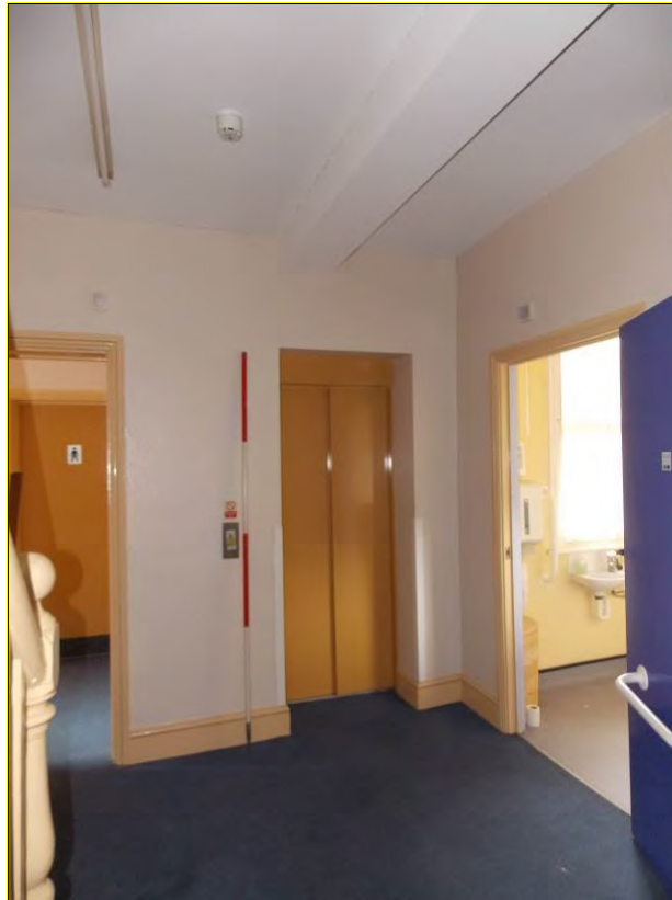
Figure 30: North wall of Room G3. Note the stub of a removed wall in the ceiling (Scale = 2m).
