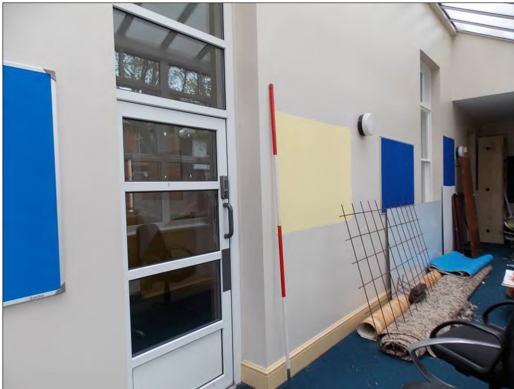
Figure 26: Detail of doorway inserted into an original window opening on the north wall of Room G1 (Scale = 2m).
