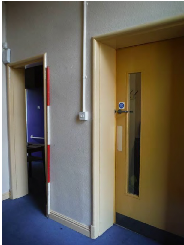
Figure 38: South wall of Room G7 showing doorways through to Room G3 and G12 (Scale = 2m).
