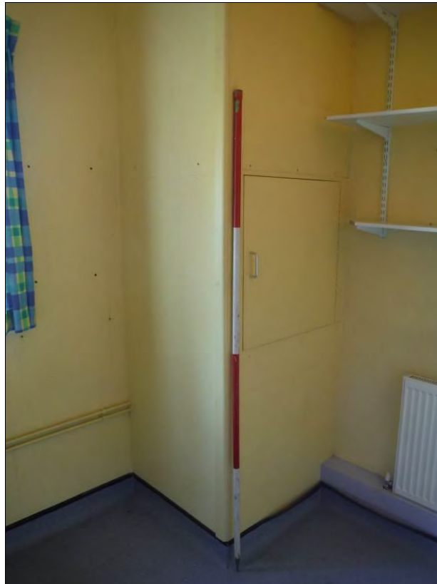
Figure 69: Inserted boiler cupboard in the north-west corner of Room F3 (Scale = 2m).
