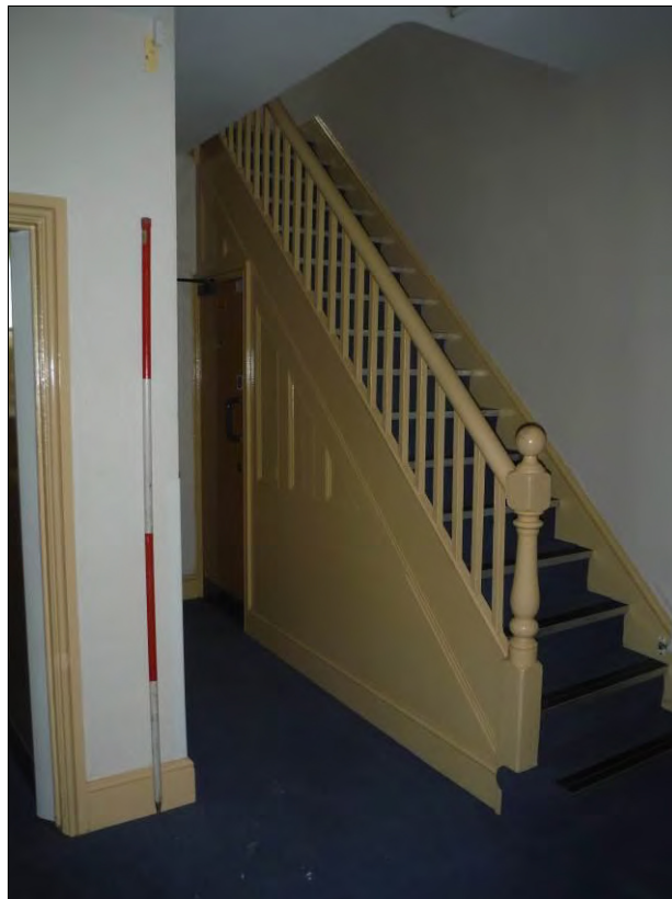
Figure 31: View south-west in Room G3 showing the remodelled straight staircase (Scale = 2m).
