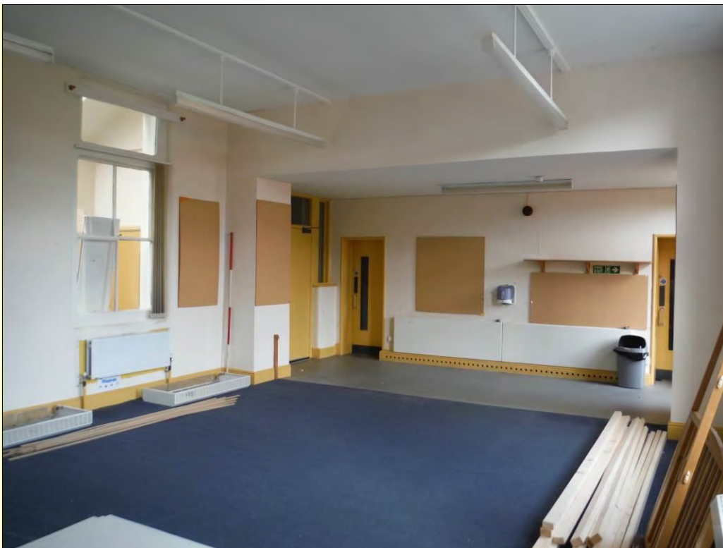
Figure 46: West end of Room G13a showing the wall opened out into Room G13b (Scale = 2m).
