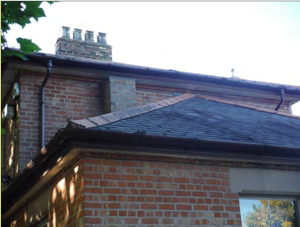
Figure 11: View of the awkward relationship between the overhanging eaves on the main building and the chimney stack rising from the eastern extension, note also the single course of modern bricks below the eaves on both roofs.
