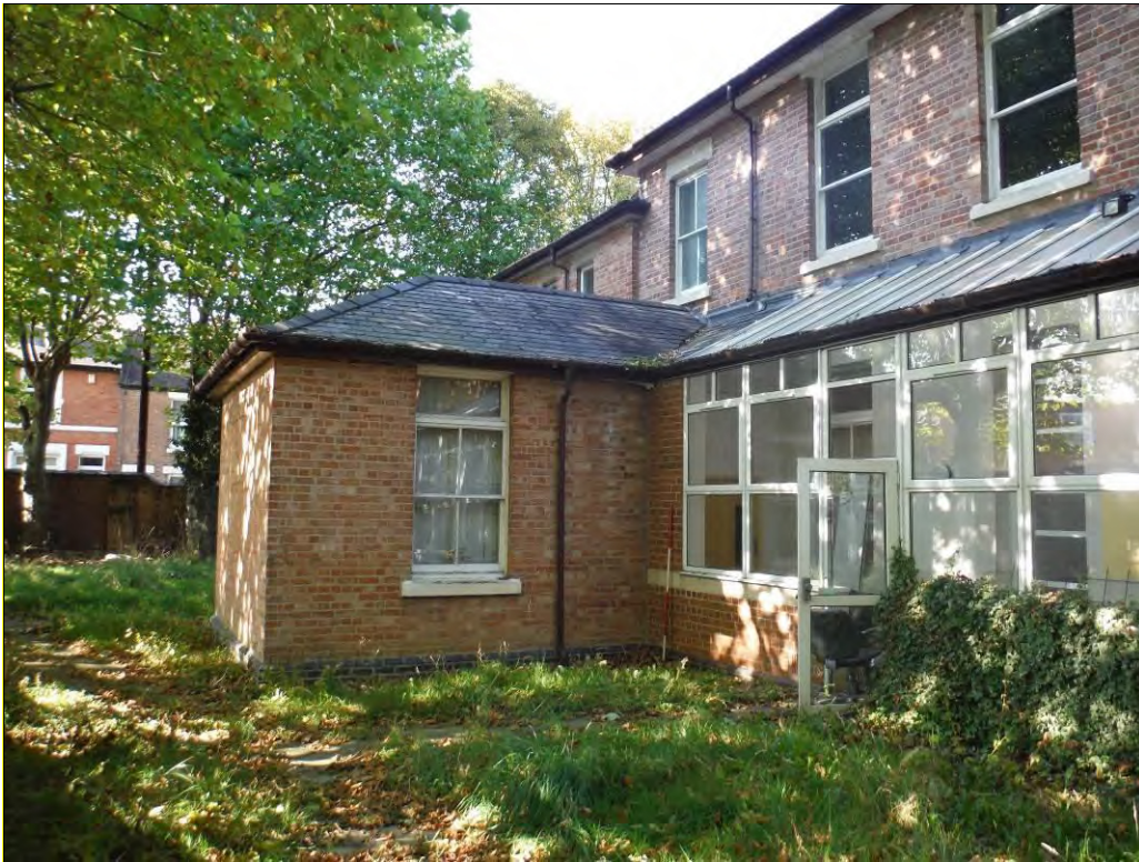
Figure 16: East elevation of southward extension to the south elevation, looking west (Scale = 2m).
