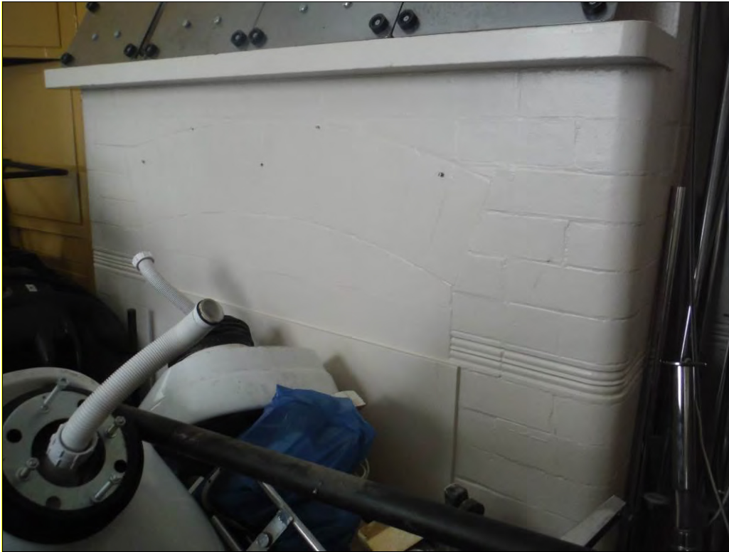
Figure 34: Detail of the glazed brick chimney breast in the west wall of Room G5.
