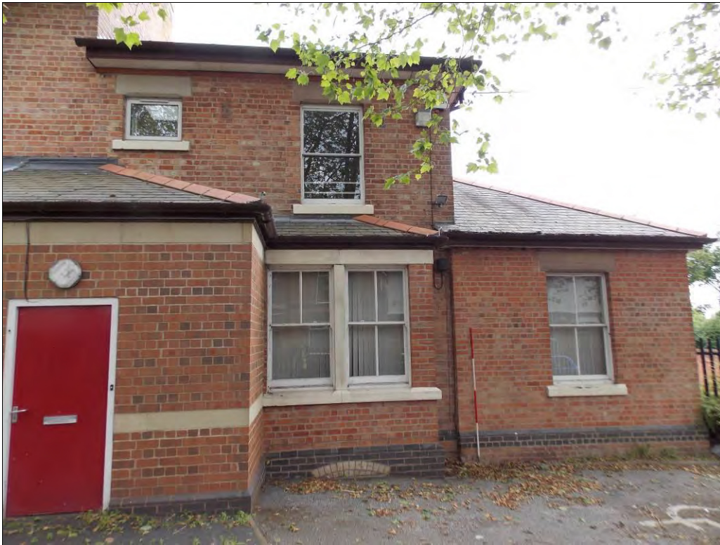
Figure 14: East end of the south elevation, looking north. Note the remodelled first floor windows – the western one much reduced in size and the eastern one with patched brickwork to its west side (Scale = 2m).
