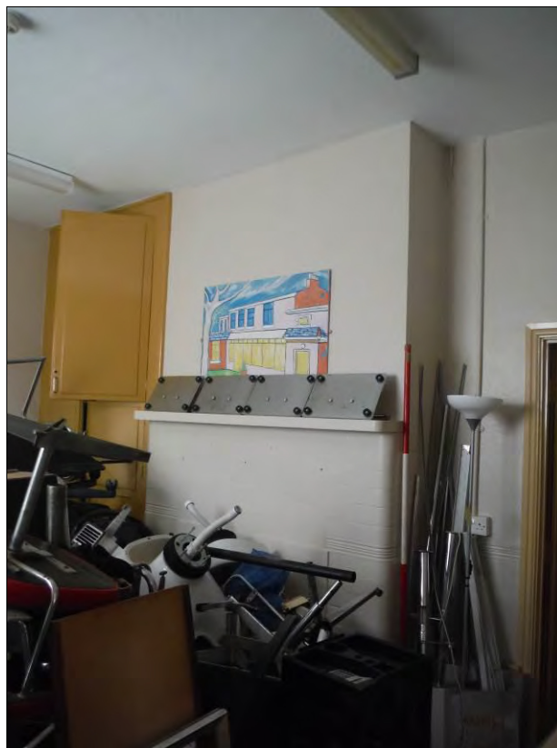
Figure 33: West wall of Room G5 showing the large fireplace and its adjacent cupboard (Scale = 2m).
