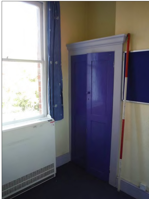
Figure 84: Detail of cupboard on the north side of the chimney breast in Room F13 (Scale = 2m).
