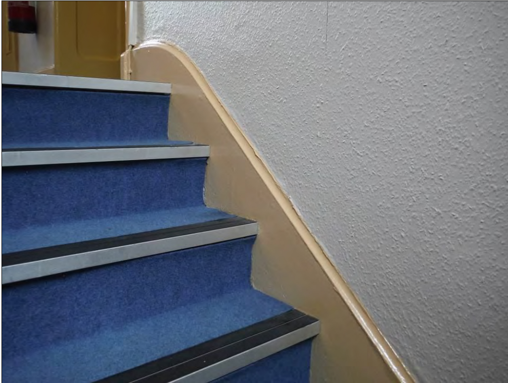
Figure 78: Original skirting board on the east side of the staircase in Room F8.
