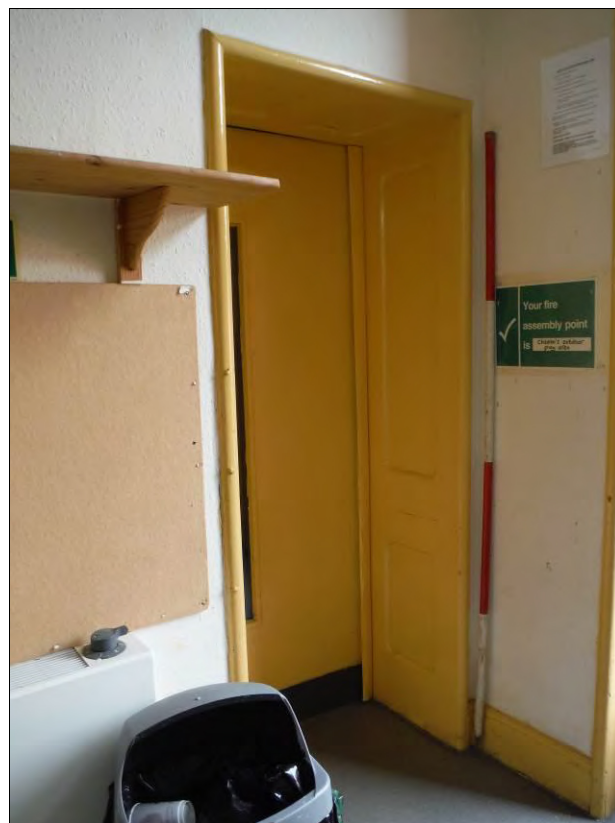
Figure 50: Detail of inserted doorway with a deep timber panelled doorcase in the west wall of Room G13b (Scale = 2m).
