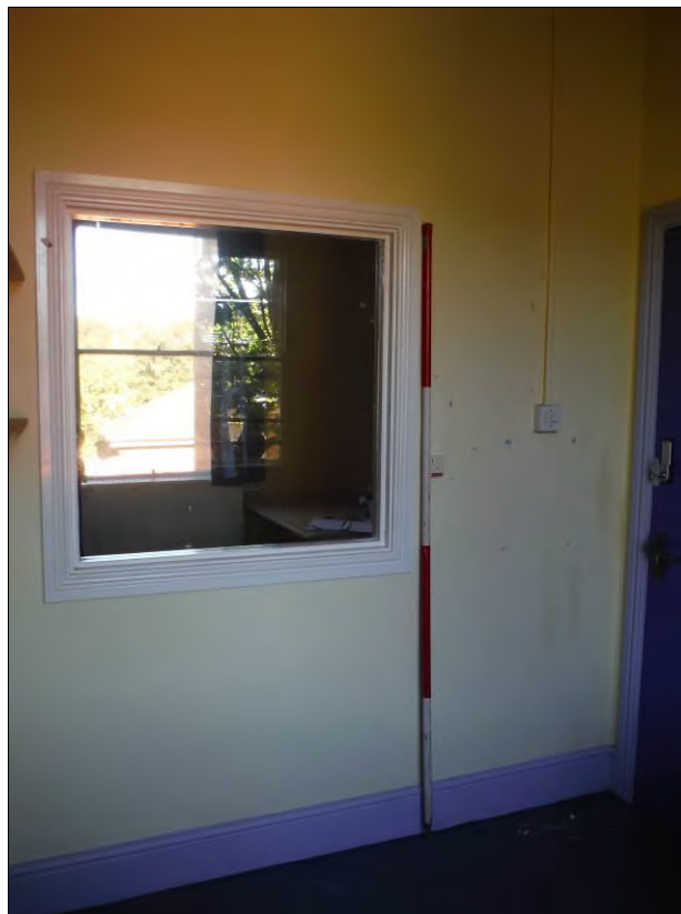
Figure 85: Inserted glazed hatch in the south wall of Room F13 (Scale = 2m).
