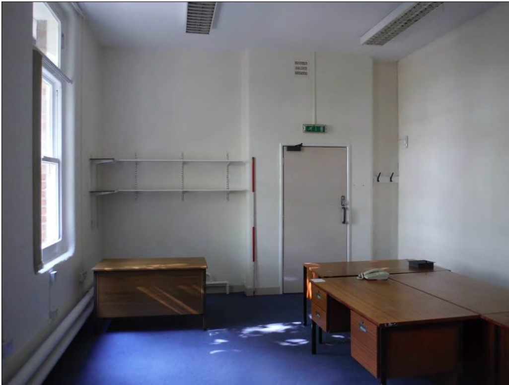
Figure 75: View west within Room F7 showing doorway inserted into former chimney breast (Scale = 2m).
