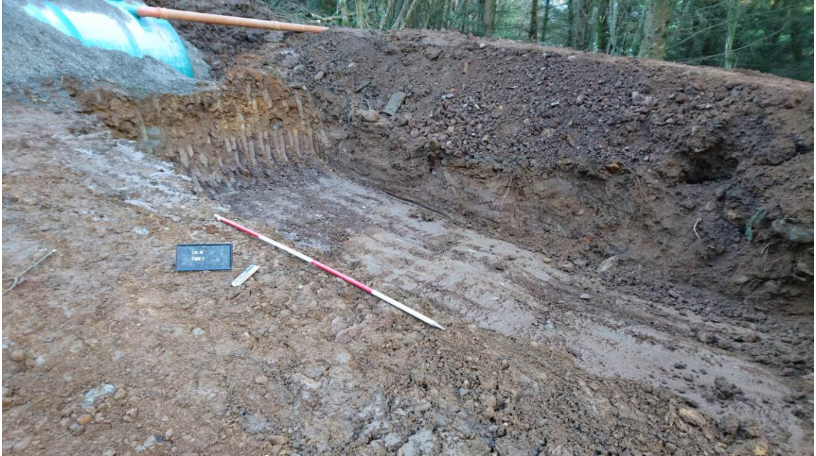
Figure 9. View facing south-east of septic tank area 1. Phase B (scale= 1 x 2m).
