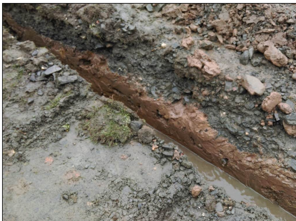
Figure 4. Excavation of a trench across a road showing tarmac with grey chippings (007) beneath. Orange/brown natural clay can be seen in the base of the trench. Phase A.
