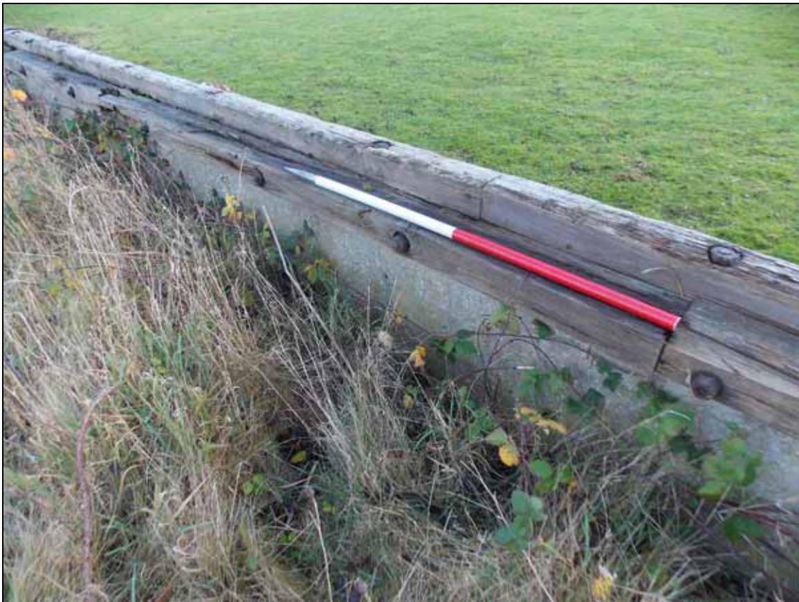
Figure 21: Detail of sill with scarf joint bolted up to the concrete plinth, looking north-west (scale 1m).
