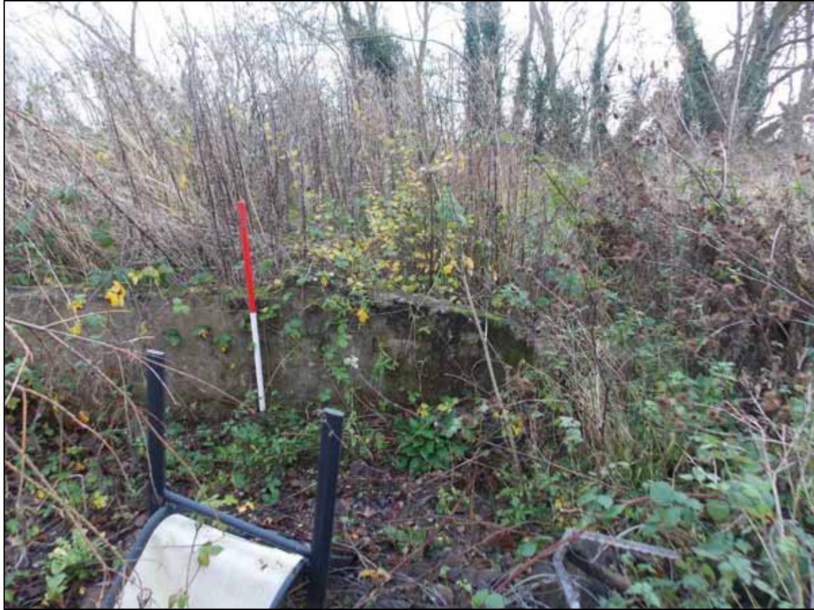
Figure 31: Detail of the sloped south-western end of the front plinth, looking south-east (scale 1m).
