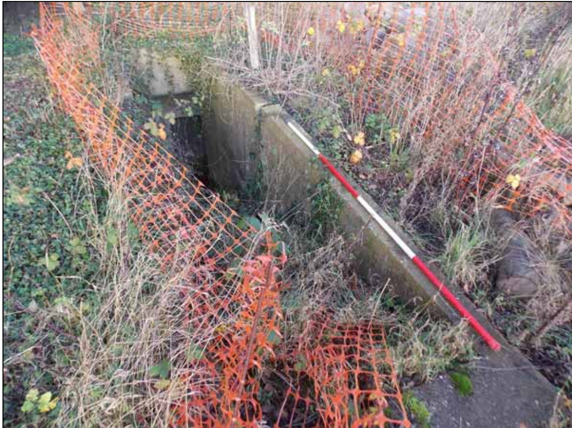
Figure 11: Flight of steps of Structure C flanked by blast wall, looking north-east (scale 2m).
