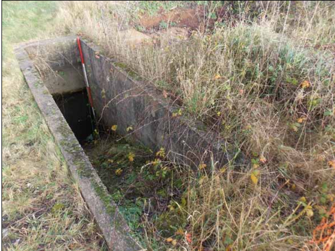
Figure 7: Flight of steps of Structure B flanked by blast wall, looking north-east (scale 2m).
