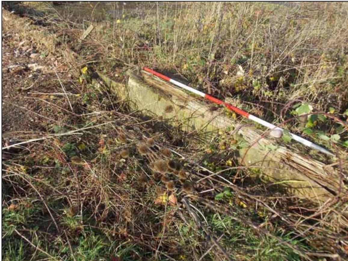
Figure 18: Detail of northern plinth with partially decayed sill attached with bolts (scale 2m).
