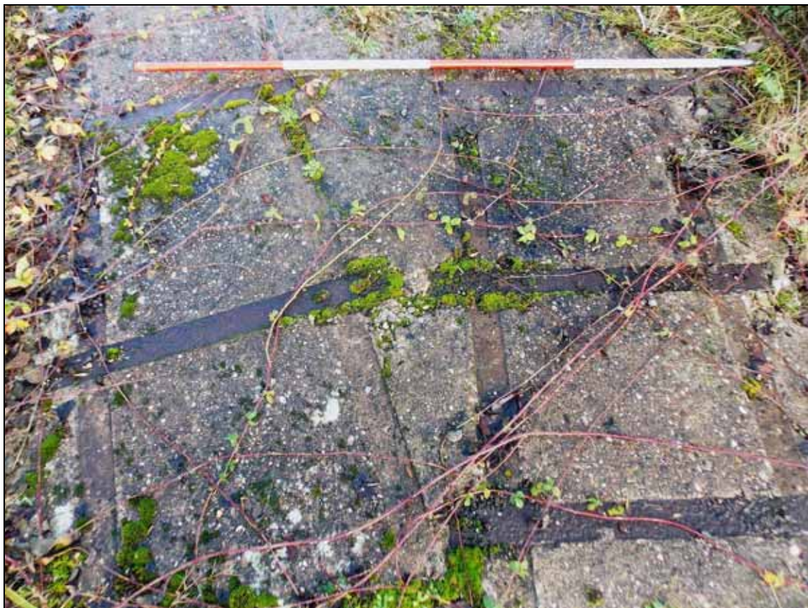
Figure 27: Detail of concrete pad with surviving cast-iron sleeper, looking north-east (scale 2m).
