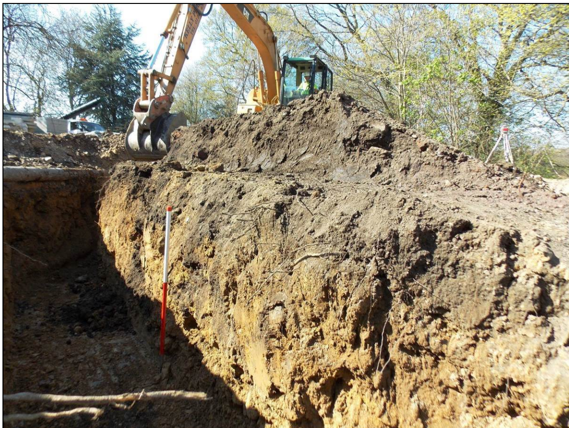
Figure 15: Excavated trench within the northern watching brief area, looking south-west (scale 1m).
