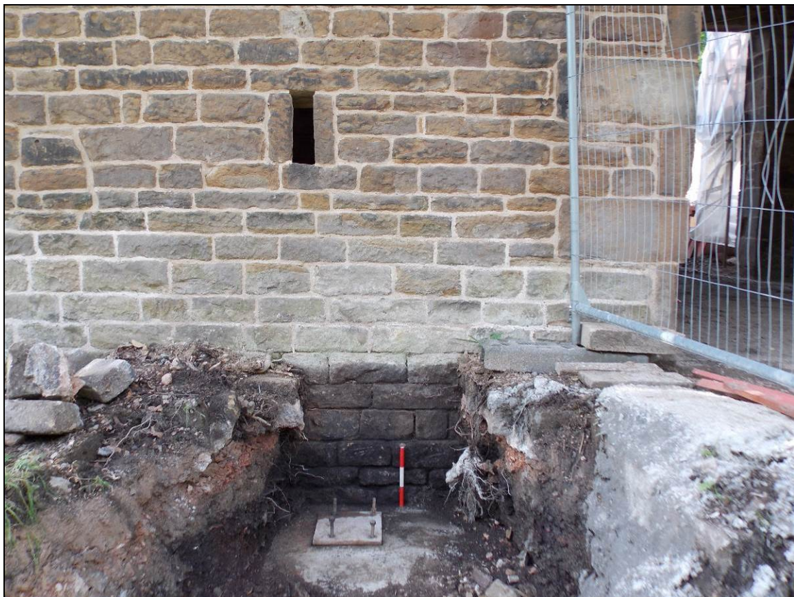
Figure 12: Fully excavated trench exposing the masonry of the Old Barn, looking south (scale 300mm).
