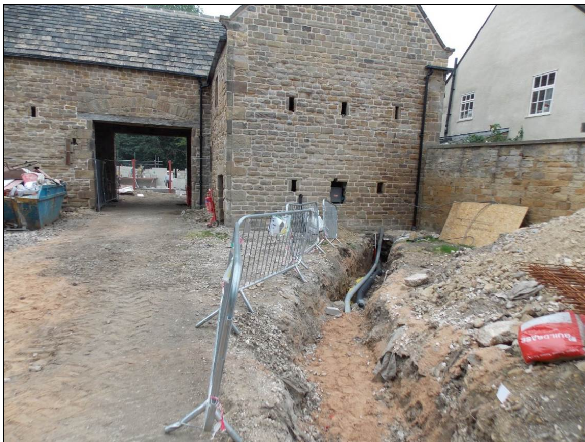
Figure 18: Service trench to the south of the Old Barn, looking north (scale 1m).
