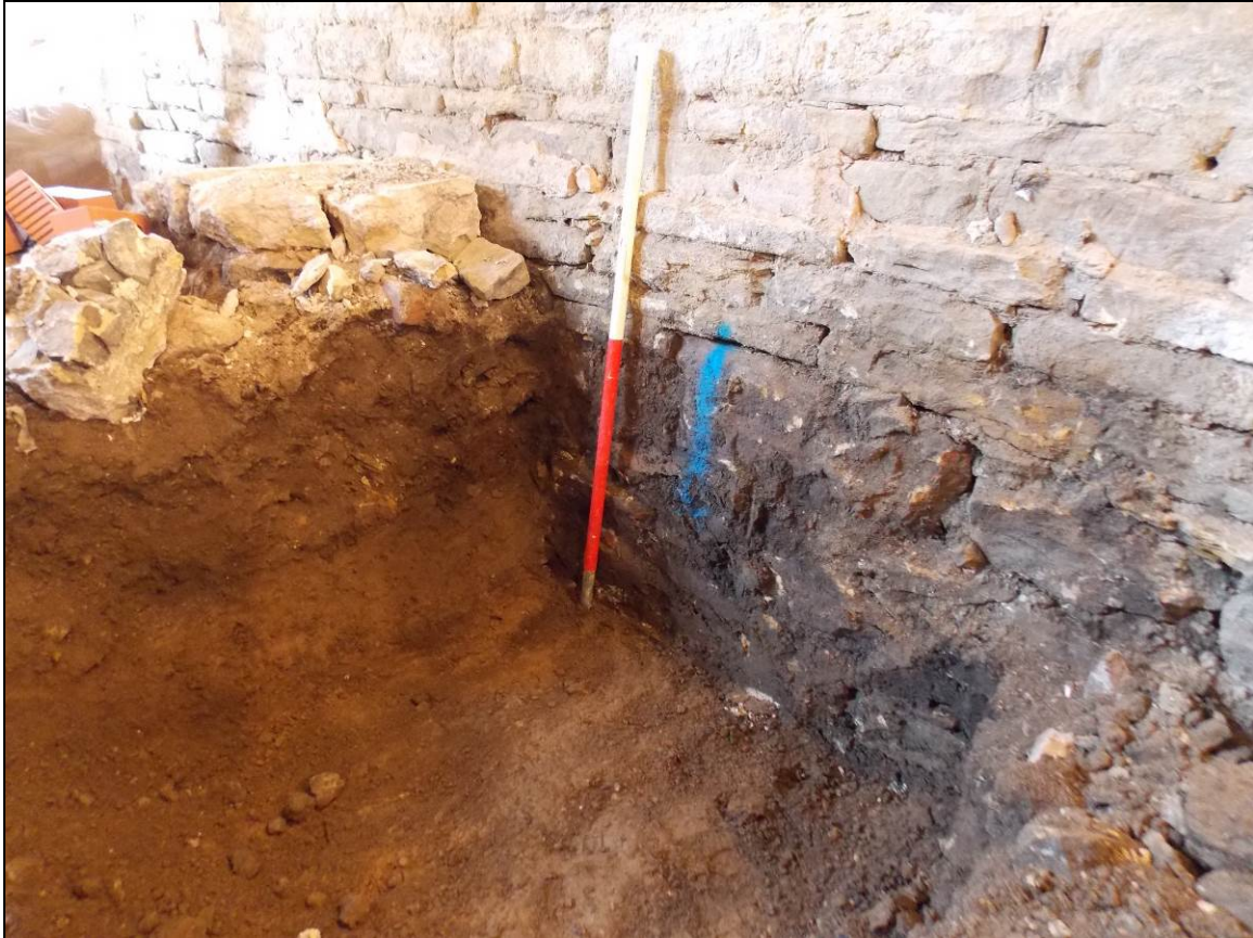
Figure 23: Underpinning trench against the eastern side of the north wall (scale 1m).
