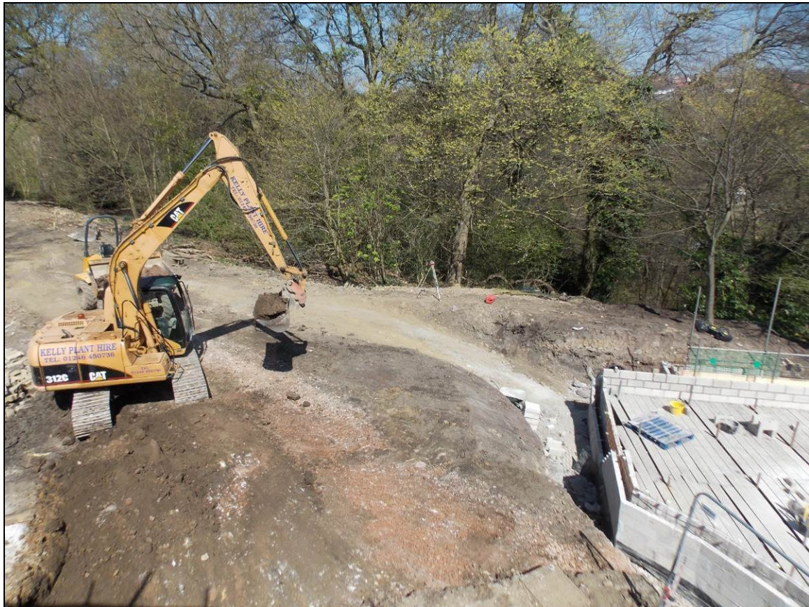
Figure 13: Excavation to the west of the main strip, map and sample area, looking north-west.
