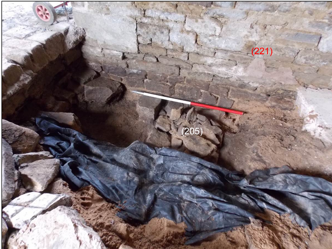
Figure 19: Foundation wall (205) abutting the northern wall (221) of the Old Barn (scale 1m).
