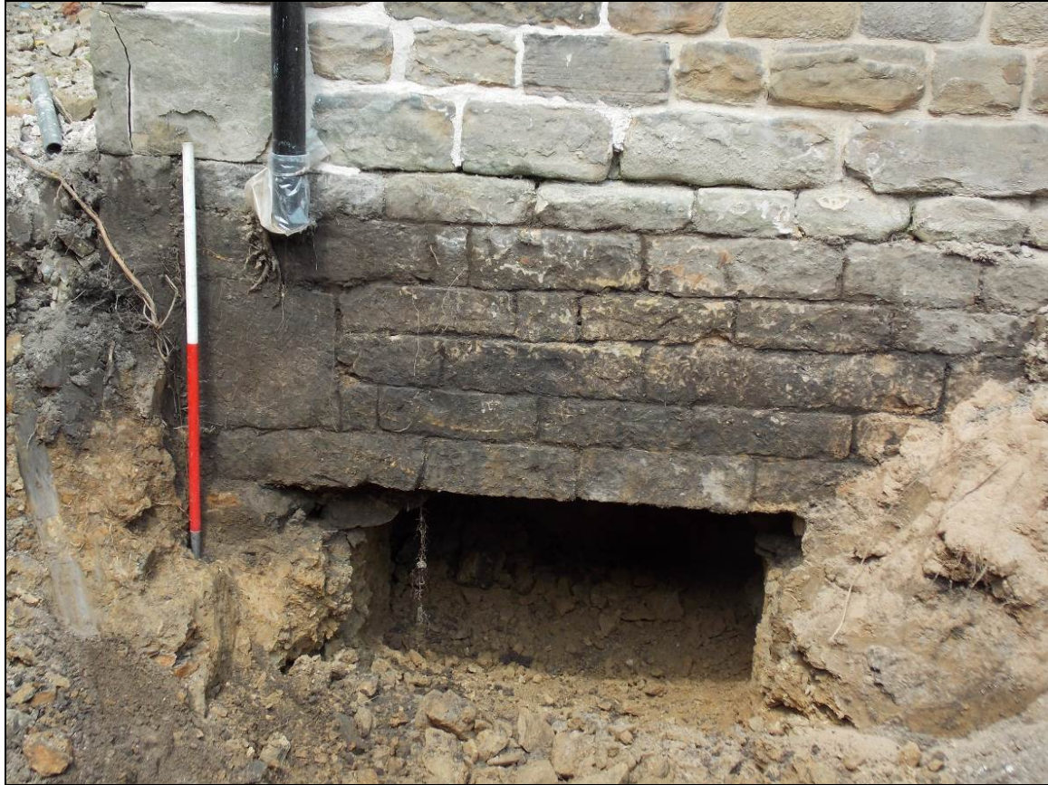
Figure 27: Underpinning trench against the external south wall adjacent to the main doorway (scale 1m).
