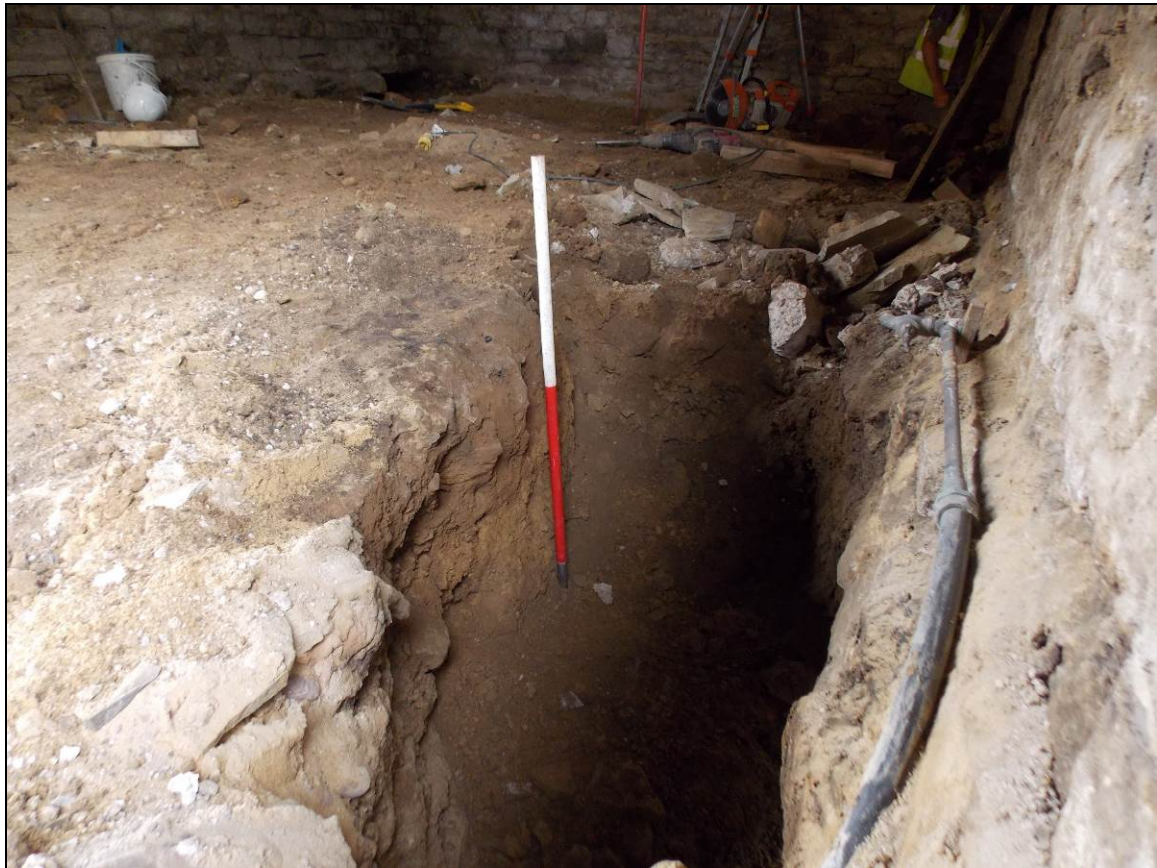
Figure 25: Underpinning trench against the western side of the north wall (scale 1m).
