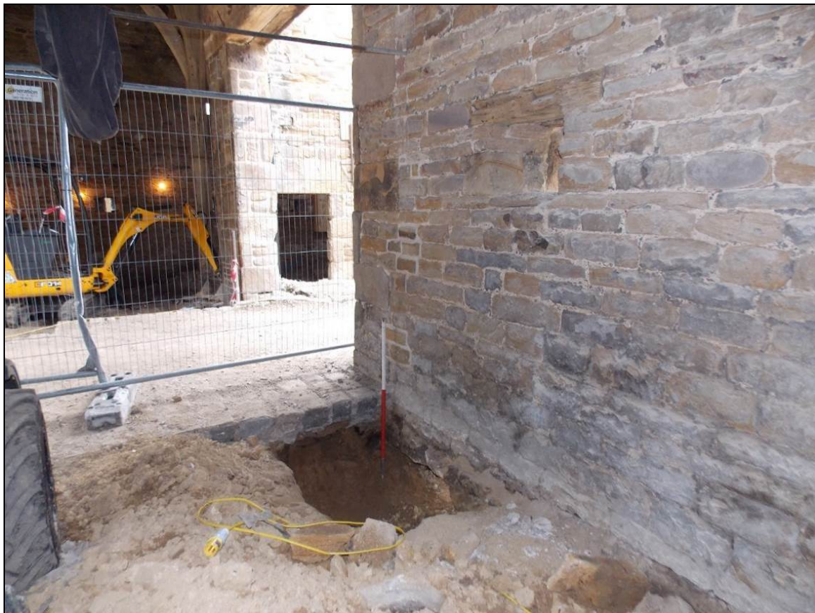
Figure 22: Underpinning trench adjacent to the central paved area, looking east (scale 1m).
