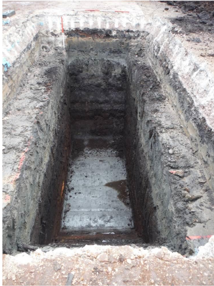
Figure 9. Trench 1 looking east showing the surface of the lower alluvium (scales = 1m and 2m).
