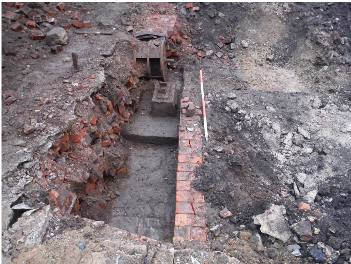
Figure 5. Excavation of the trench 1, with cellar workshop revealed, looking south-west (scale = 2m)
