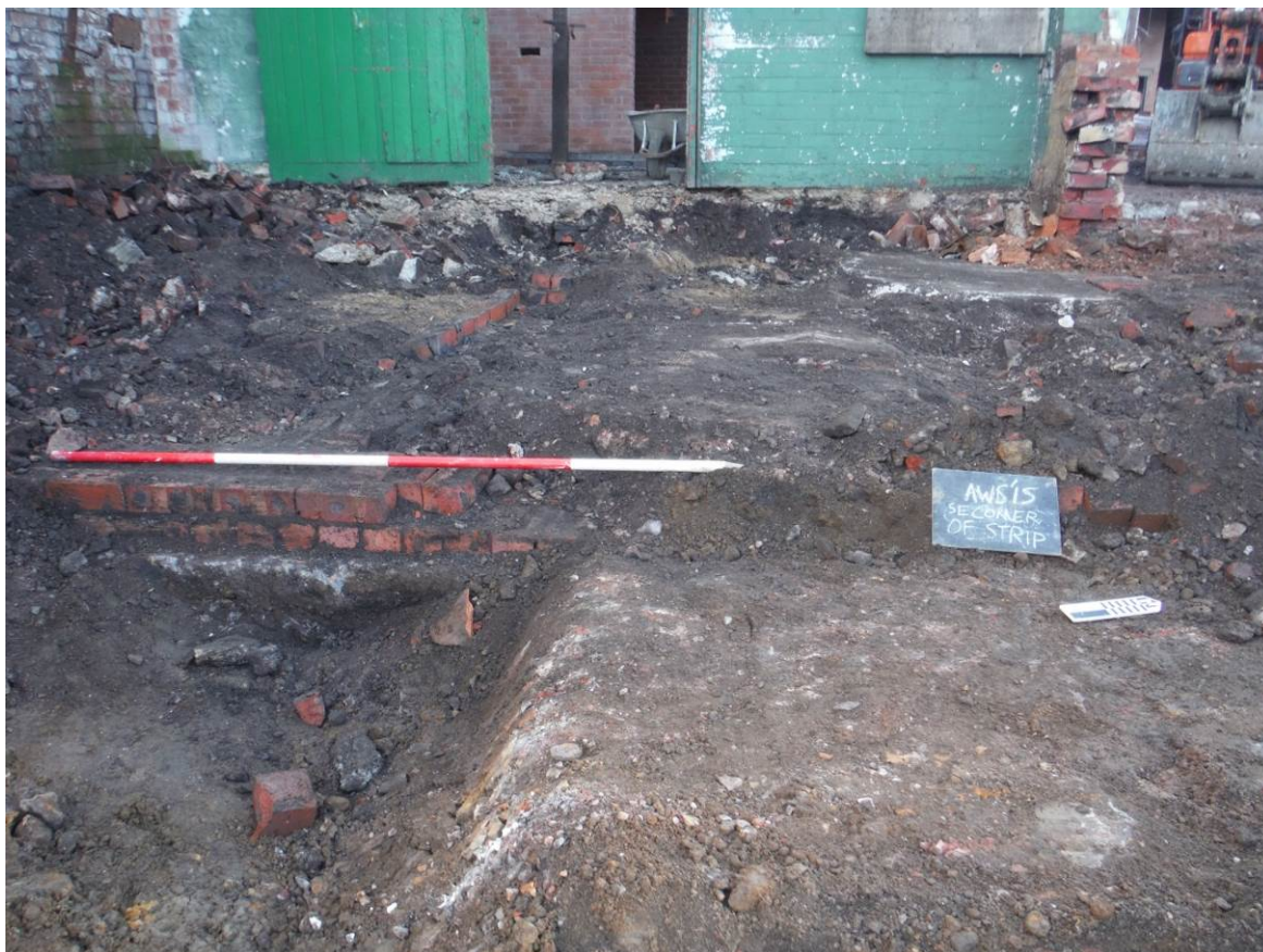
Figure 3. Initial excavation of southern end of stripping area, looking north-west (scale = 2m).
