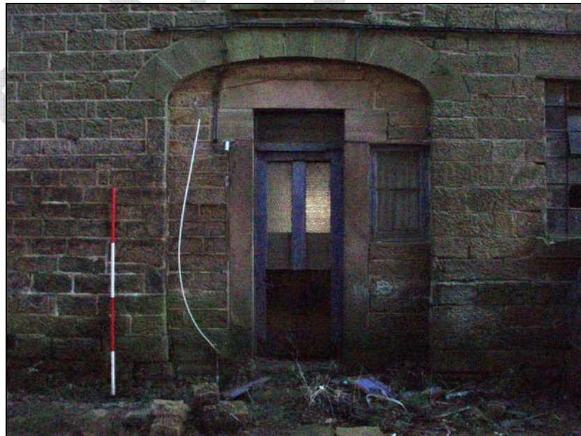
Fig. 27. Photograph of the doorway created within the original tunnel on the south-west façade of the house (facing north-east)
