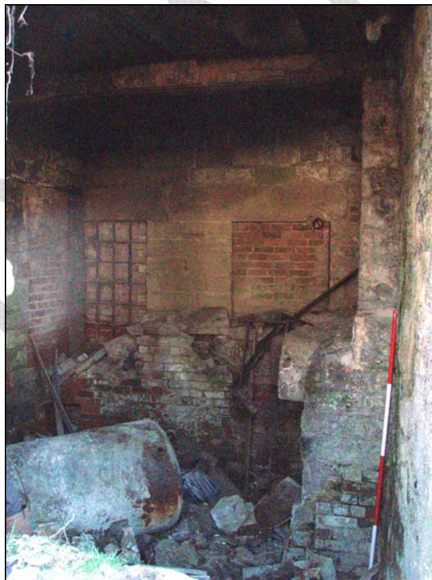
Fig. 10. Photograph of the interior of the boiler house and the infilled windows in the mill wall (facing south-west) (scale = 2m).
