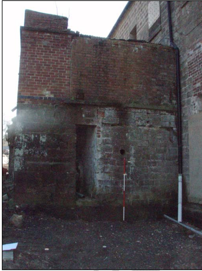
Fig. 15. Photograph of the brick extension located on top of the boiler house (facing south-east) (scale = 2m).
