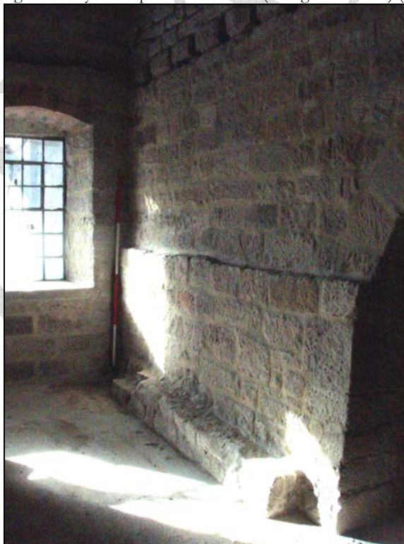
Fig. 39. Photograph of the south side of the south-east partition wall (facing west) (scale = 2m).
