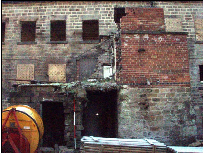
Fig. 9. Photograph of the boiler house and red brick extension (facing south-west) (scale = 2m).
