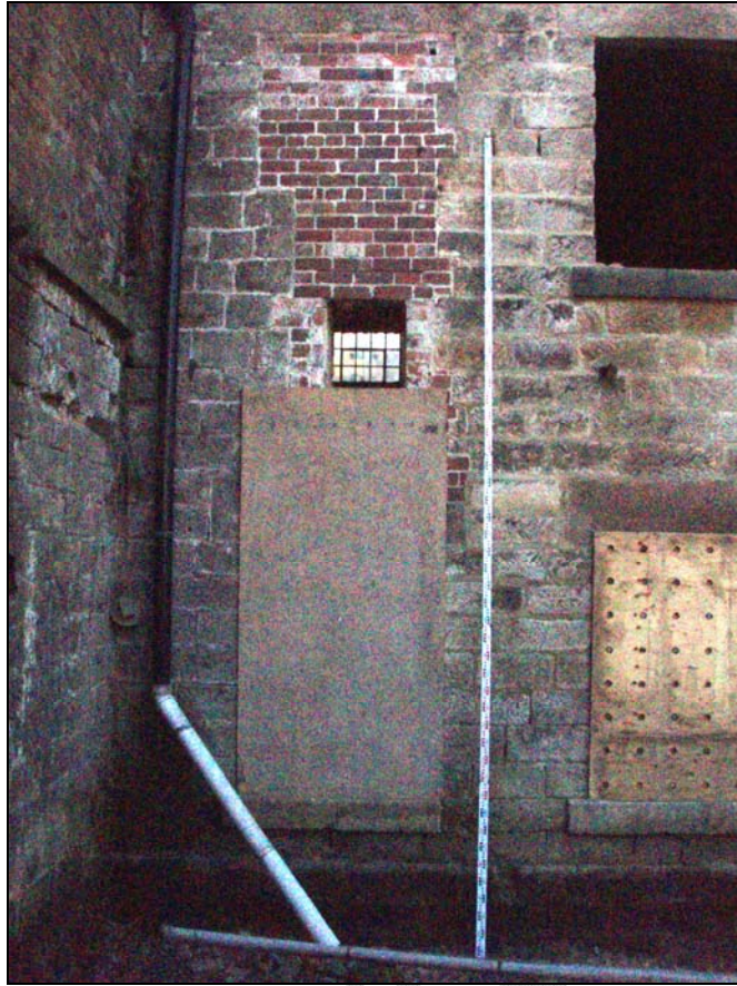
Fig. 8. Photograph of infilling of the wall and one of the windows in the north-east façade of Scholes Mill, Tansley (facing south-west).
