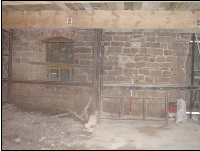
Fig. 52. Photograph of the south-east wall of the ground floor of the mill (facing south-east) (scale = 1m).
