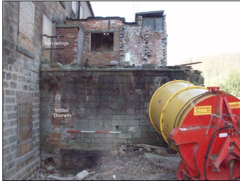
Fig. 13. Photograph of infilled doorway and iron railings in south-east wall of extension (facing north-west).
