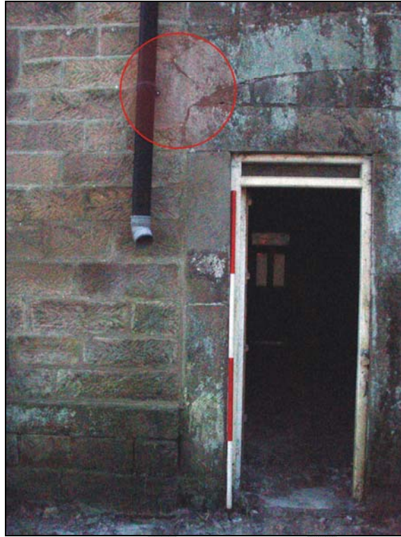
Fig. 23. Photograph of the stones of the arch which have been keyed into the construction of the mill (facing south-west) (scale = 2m).
