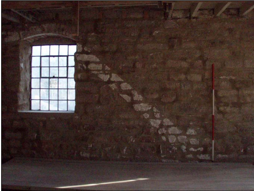
Fig. 50. Photograph of position of stairway which overlies a window in the south-east façade of the mill (facing south-east).
