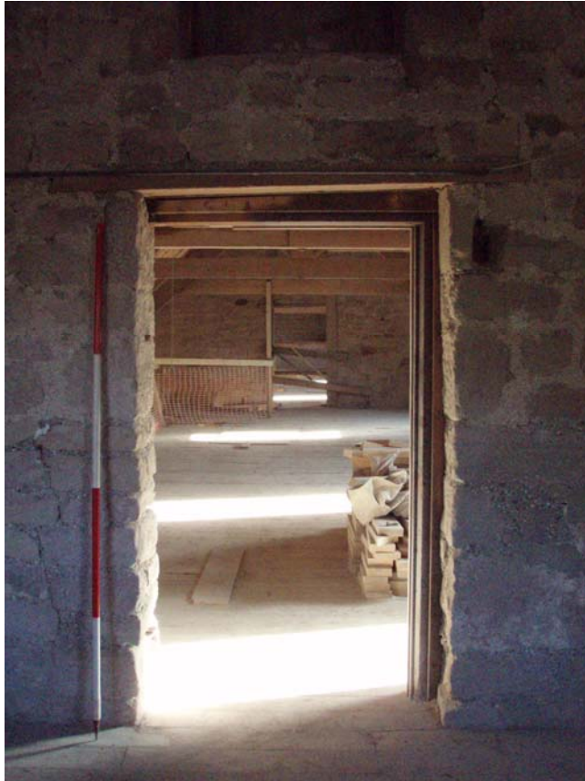
Fig. 53. Photograph from the first room at the top of the staircase in the attic of the mill (facing south-east) (scale = 2m).
