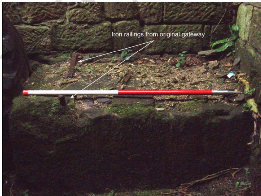
Fig. 19. Photograph of the remains of the iron gateway from phase one of the construction of the entrance to Scholes Mill (facing north-east) (scale = 1m).
