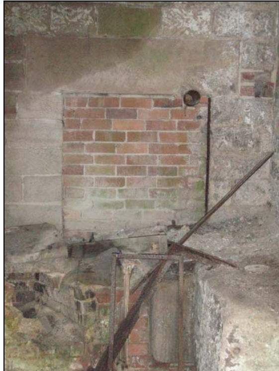
Fig. 11. Photograph of an infilled window on the south-east interior wall of the boiler house (facing south) (scale = 1m).
