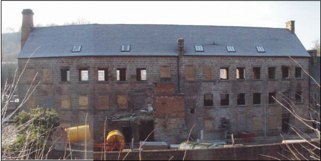
Fig. 3. Photograph of the windows in north-east façade of the mill (facing south-west) (scale = 5m).
