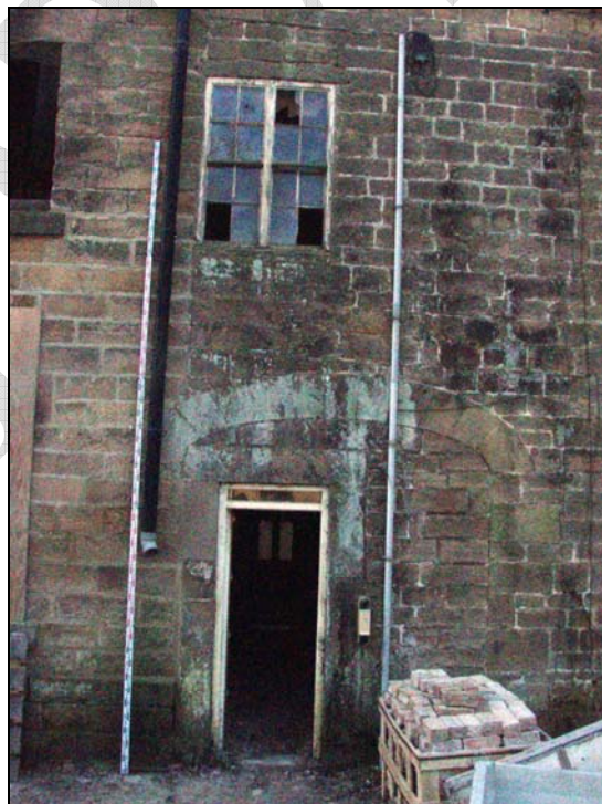
Fig. 24. Photograph of the join between the mill and the house and the infilled archway on north-east façade of the house (facing south-west) (scale = 5m).
