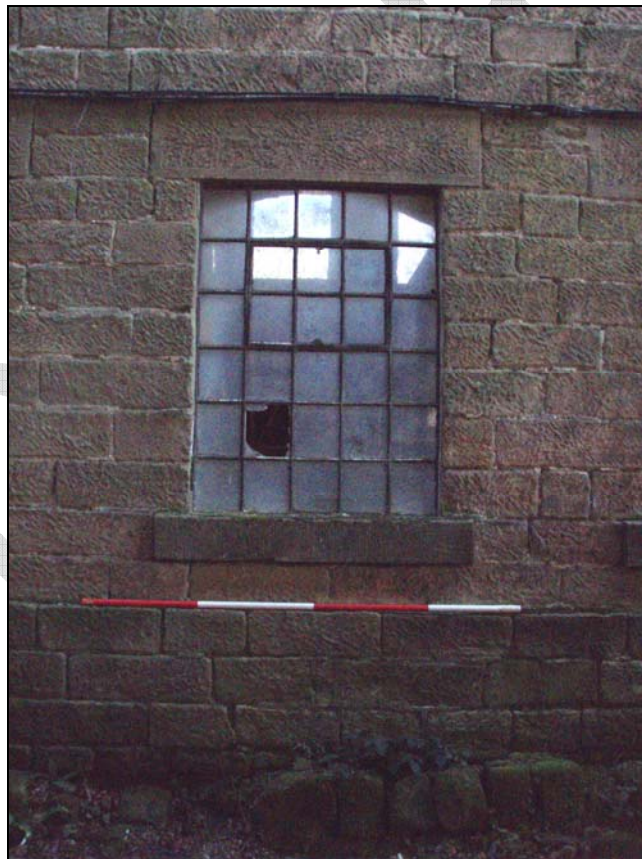
Fig. 4. Photograph of the lower course blocks of stone, the foundations and a standard window in the south-west façade of the mill (facing north-east) (scale = 2m).
