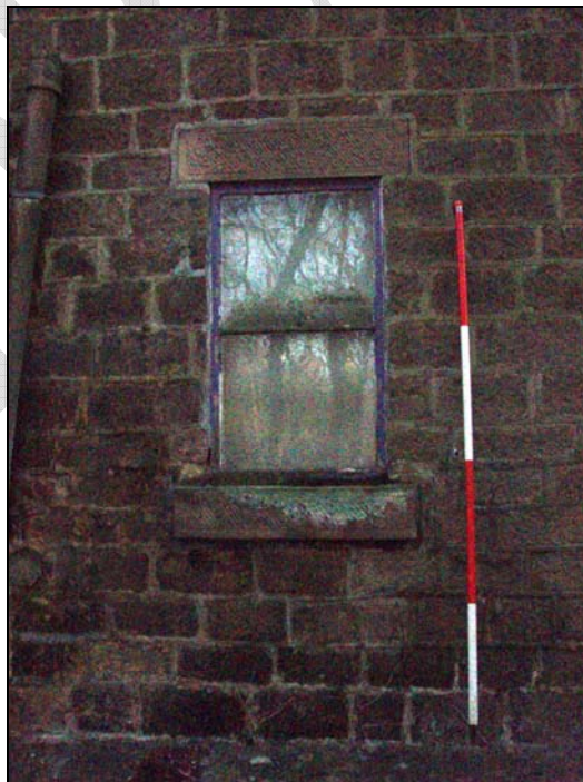
Fig. 32. Photograph of the window in the north-west façade of the house (facing south-east) (scale = 2m).
