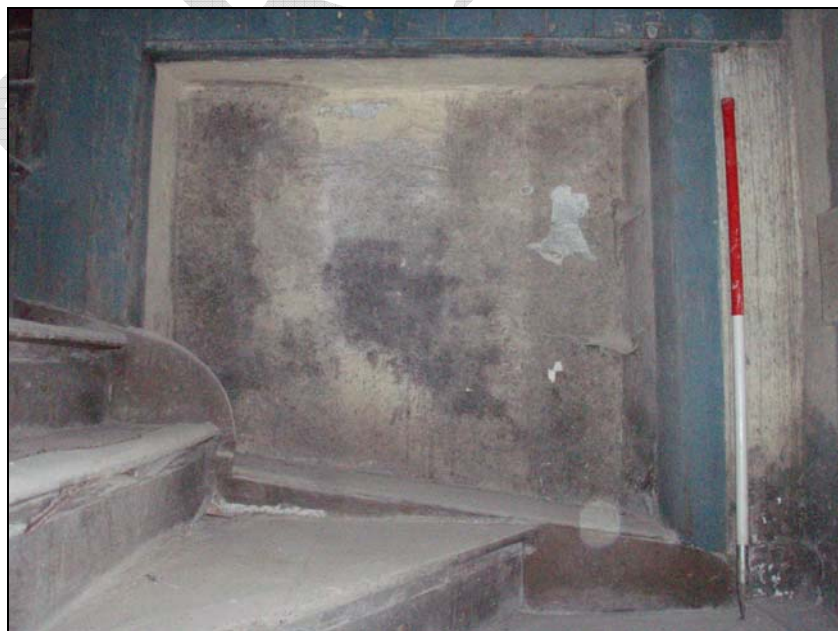
Fig. 47. Photograph of an infilled window which was covered by the staircase of the mill (facing north-west) (scale = 1m).
