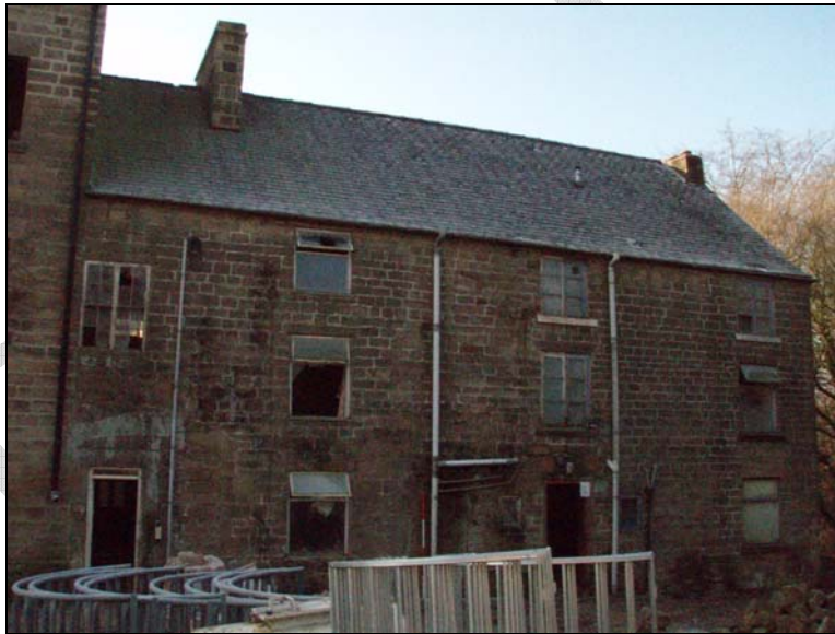
Fig. 28. Photograph of the windows and doors on the north-east façade of the house (facing south-west) (scale = 2m).
