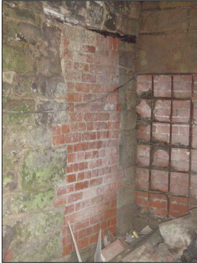
Fig. 14. Photograph of an infilled doorway on the interior south-east wall of the boiler house (facing south) (scale = 1m).
