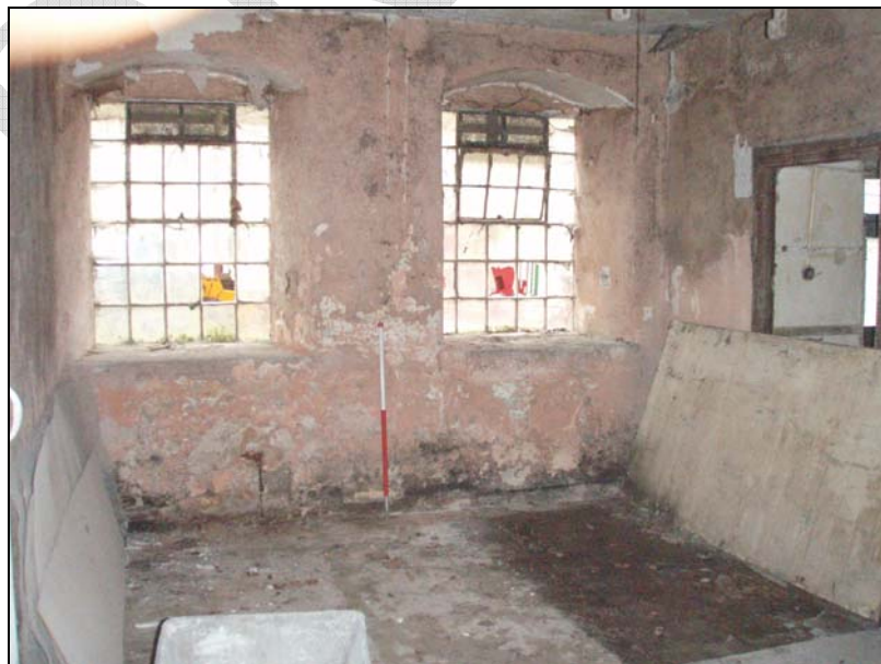
Fig. 34. Photograph of ground floor back room showing windows (facing south-west) (scale = 2m).
