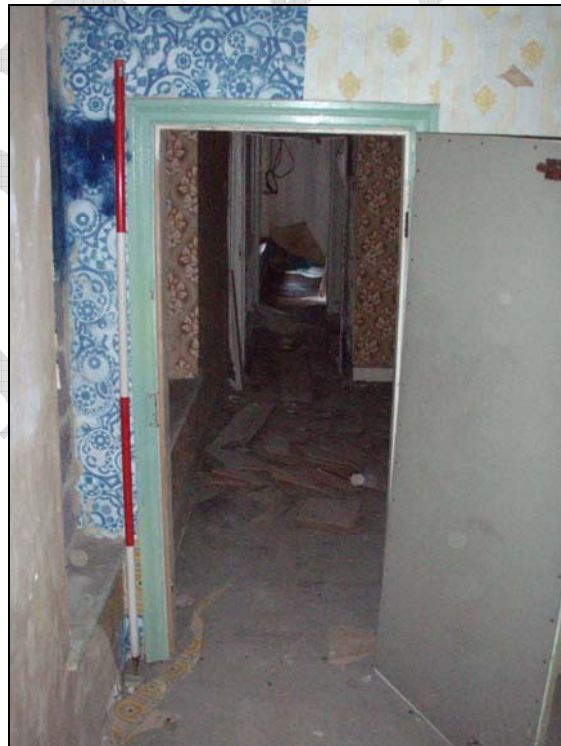
Fig. 59. A doorway on the first floor of unit one into the rest of the structure (facing north west) (scale = 2m).
