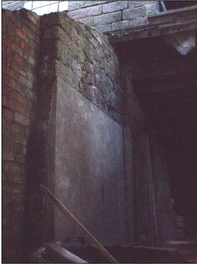
Fig. 22. Photograph of the plastered section of the porch (facing north) (scale = 1m).
