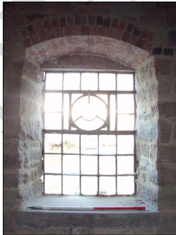
Fig. 41. Internal window with arched lintels and angled brick surrounds on the ground floor of the mill (facing north-east) (scale = 1m).
