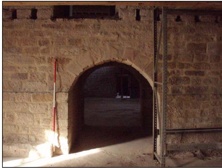
Fig. 40. Photograph of the south-east partition walls and arch on the ground floor of the mill (facing north-west) (scale = 2m).
