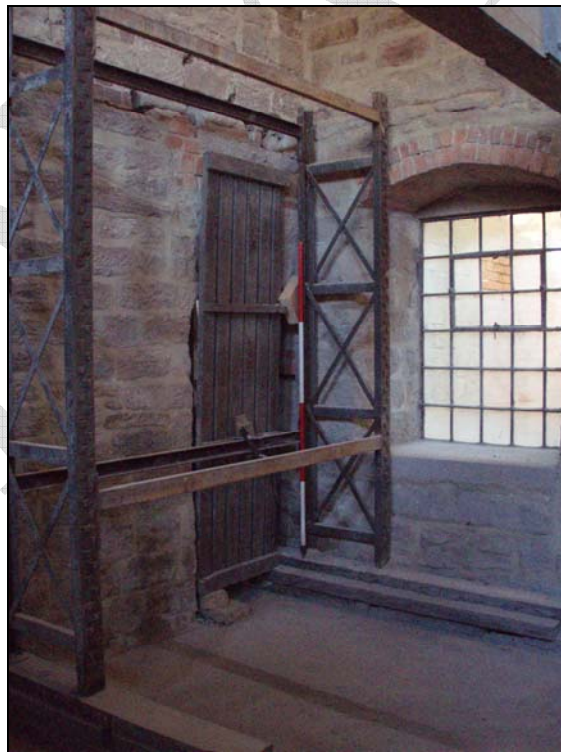
Fig. 37. Doorway in the north-west partition wall of the ground floor of the mill (facing south-east) (scale = 2m).
