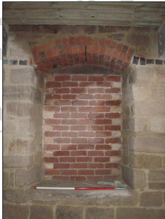
Fig. 12. Photograph of an infilled window on the north-east façade of the mill which abuts the boiler house (facing north-east) (scale = 1m).
