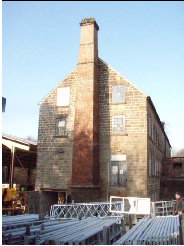
Fig. 6. Photograph of the standard windows in the South-east façade of Scholes Mill, Tansley (facing north-west).
